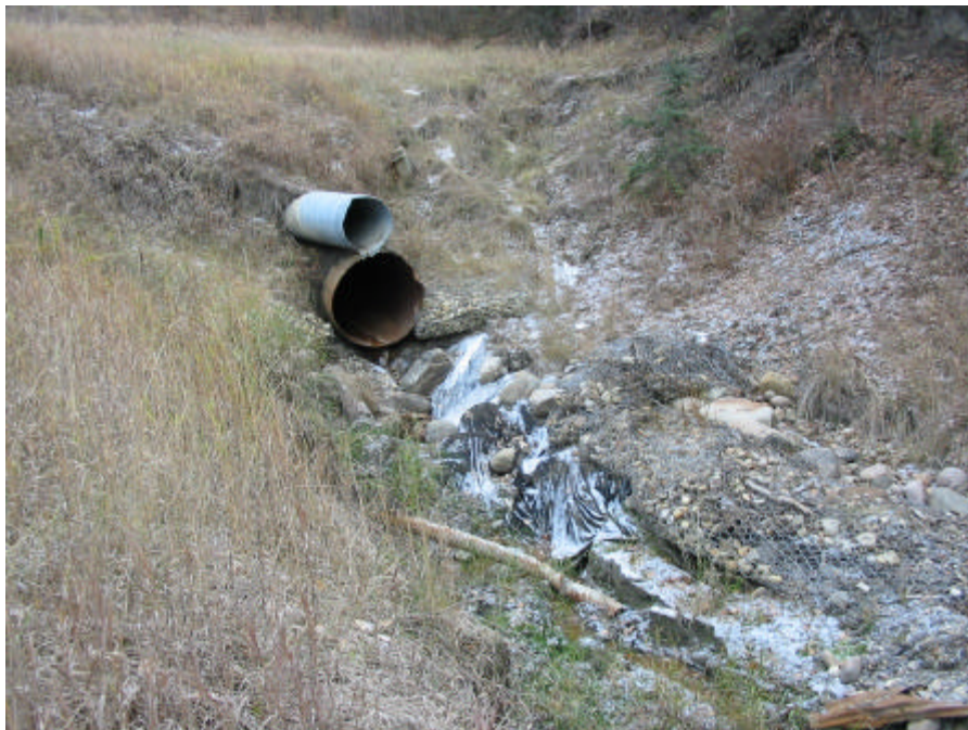
Photo 3: Whitemud River, culvert outlet erosion of gabions, 2002
