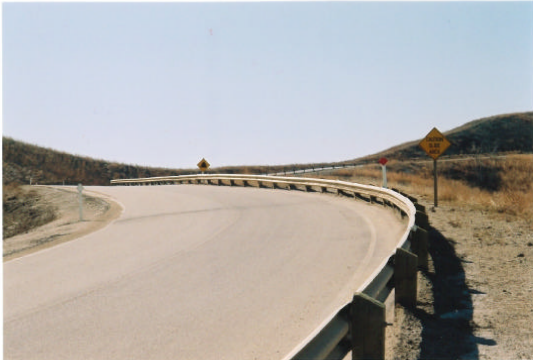
Photo 4: Judah Hill, north of Zone D2, settlement and cracks in pavement, May 2002.
