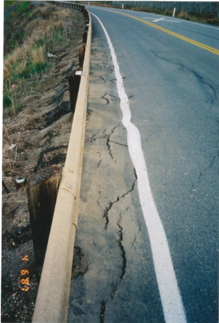
Photo 6: Judah Hill, Zone B1, settlement and cracks in pavement, October 2002.
