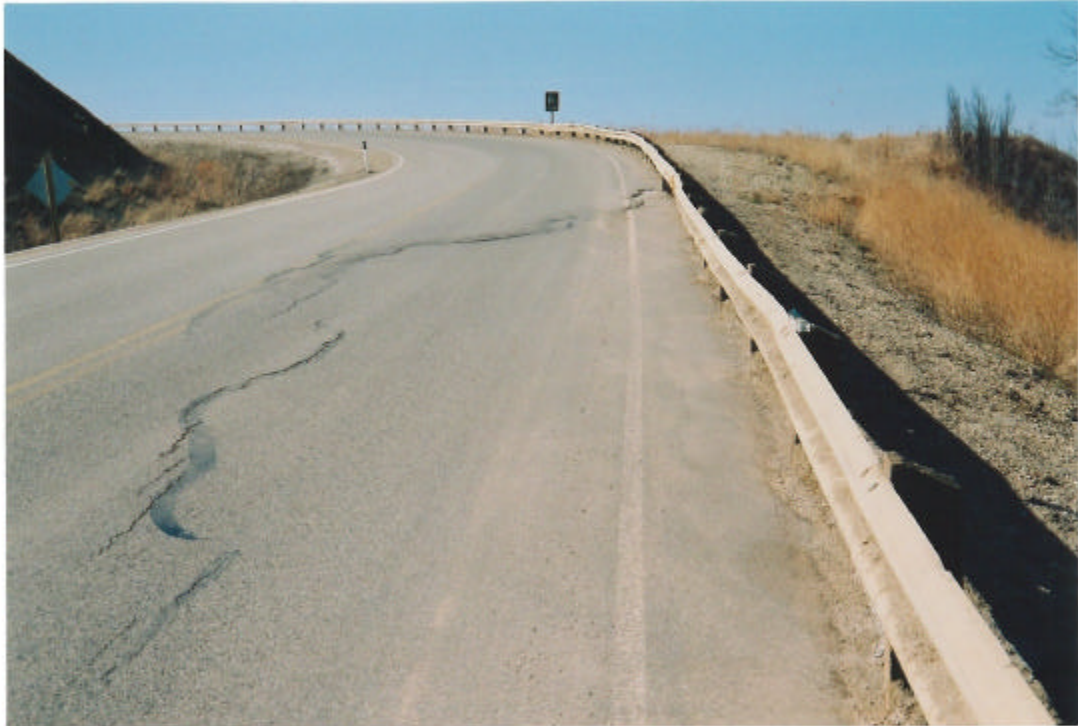
Photo 1: Judah Hill, Slide # 1 in Zone D1, settlement and cracks in pavement, May 2002.
