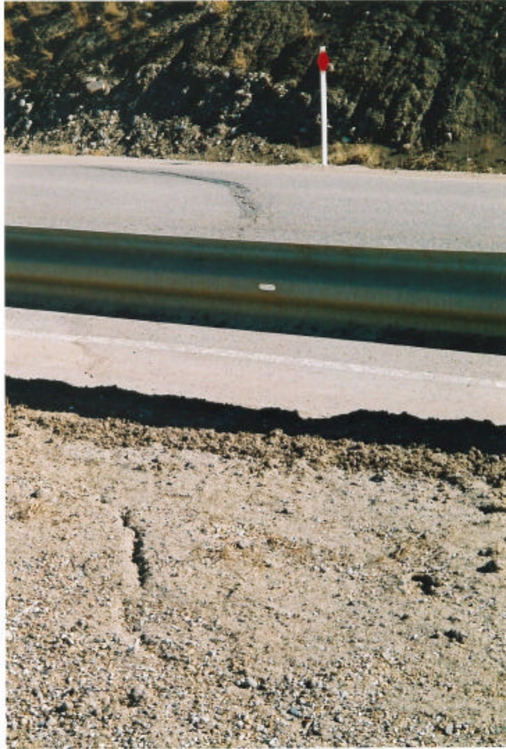
Photo 5: Judah Hill, north of Zone D2, settlement and cracks in pavement, May 2002.
