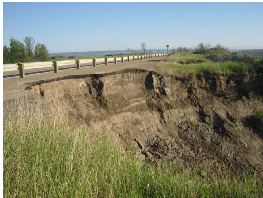
Photo 5. North side of Slide 3. Substantial retrogression of the backscarp, dark zones of seepage are visible from 1m to 3 m below the top of asphalt pavement, the Telus communications cable has fallen into the slide debris with additional debris flow observed below the backscarp.
