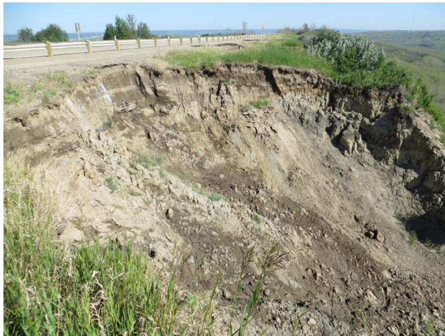
Photo 7. Looking northwards across the backscarp of Slide 4. There has been retrogression since August 2011 and some movement in the slide bowl, which is now 35 m in width. The backscarp is now at about 4m from the new guardrail alignment (increase of 0.4 m since 2011).
