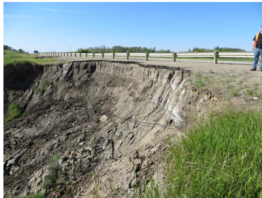
Photo 3. Retrogression movement in the backscarp of Slide 2. The backscarp is now at 1 m from the new guardrail alignment. The Telus telecommunications cable is hanging in the same position as in 2011. Some fresh debris is visible below the scarp and dark seepage stains are also visible from about 1 m to 2 m below the top of the asphalt surface.
