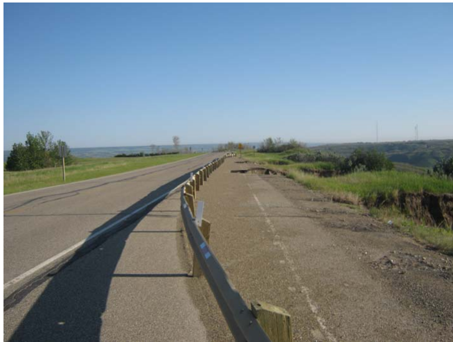
Photo 1. Looking north along Hwy744 from the south end of Slide 4.
