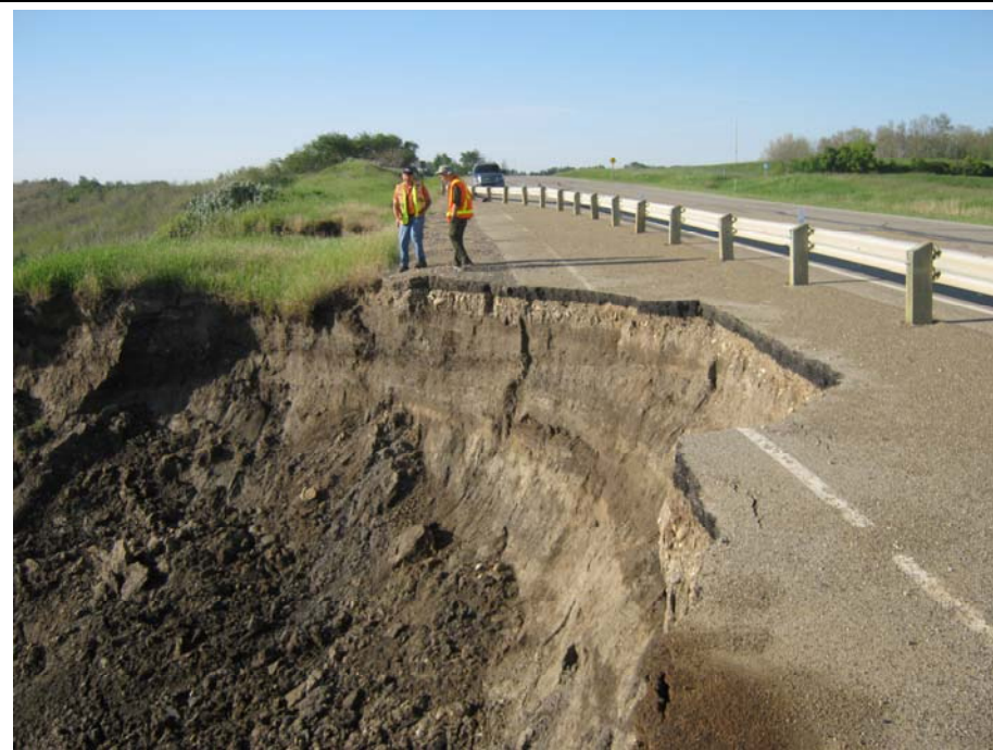
Photo 6. Looking south at the significant retrogression of the backscarp of Slide 3 (about 5 m since August 2011), now at 1 m from the new guardrail alignment and about 32 m in width.
