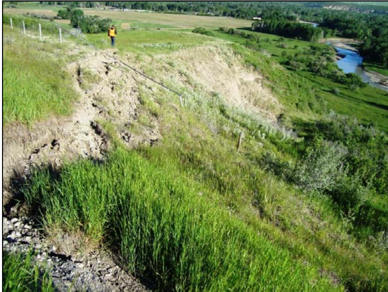
Photo 3 (June 21, 2011) Facing northwest from the north edge of the road at the landslide headscarp. The west flank of the landslide is active. The slide is well developed, with slide movement likely ongoing for many years and having displaced the fenceline north of the road, as shown in this photo.
