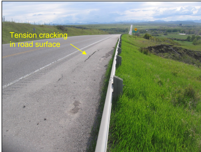
Photo 1 (June 1, 2011) Facing westbound along the highway with the position of the recent tension cracking along the north shoulder as marked. The landsliding in the valley slope is visible on the right hand side of the photo, just downslope of the highway.
