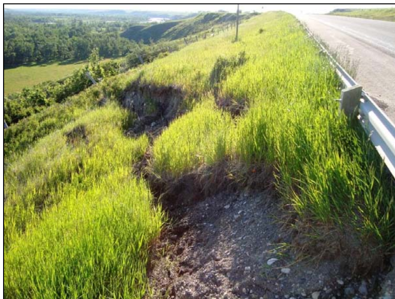
Photo 2 (June 21, 2011) Facing east along the north/downslope edge of the road at the landslide headscarp. The headscarp has fresh soil exposed, and is immediately adjacent to the road surface.
