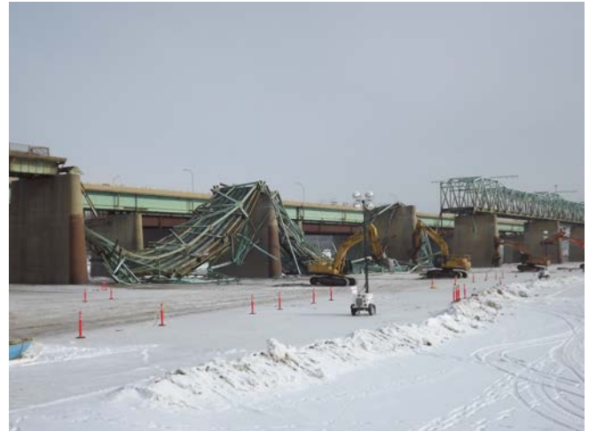
The 1965 truss design bridge is demolished to make way for the new Grant MacEwan Bridge and Franklin Avenue tunnel.
