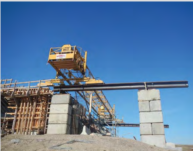
4.53 Deck finishing machine run-off rails.
