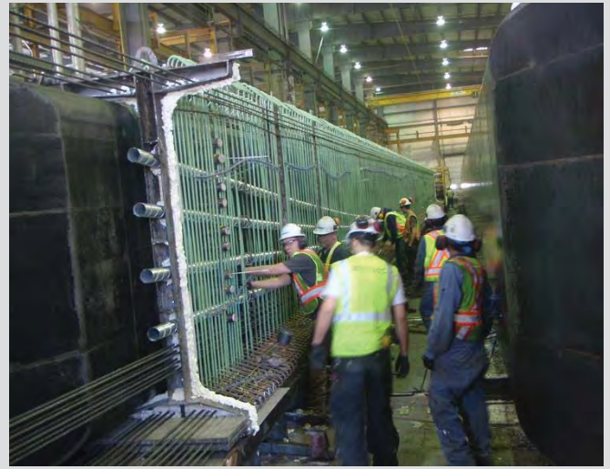
7.18 Post tensioning ducts within NU girders at fabrication shop.
