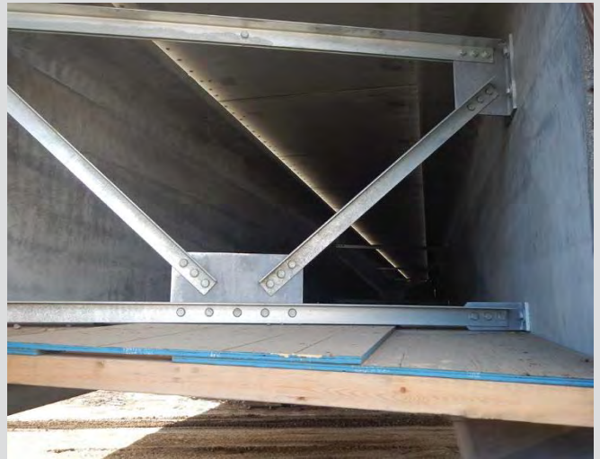
7.16 Galvanized diaphragm cross bracing installed. False deck used as a work platform.
