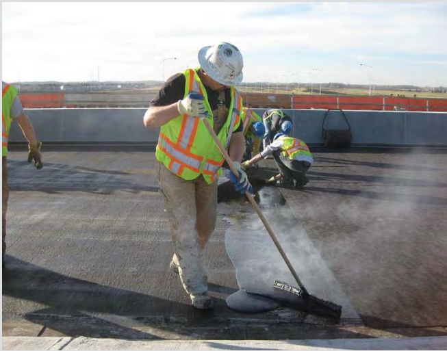
16.9 Asphalt membrane is poured from a pail and spread with a rubber squeegee.
