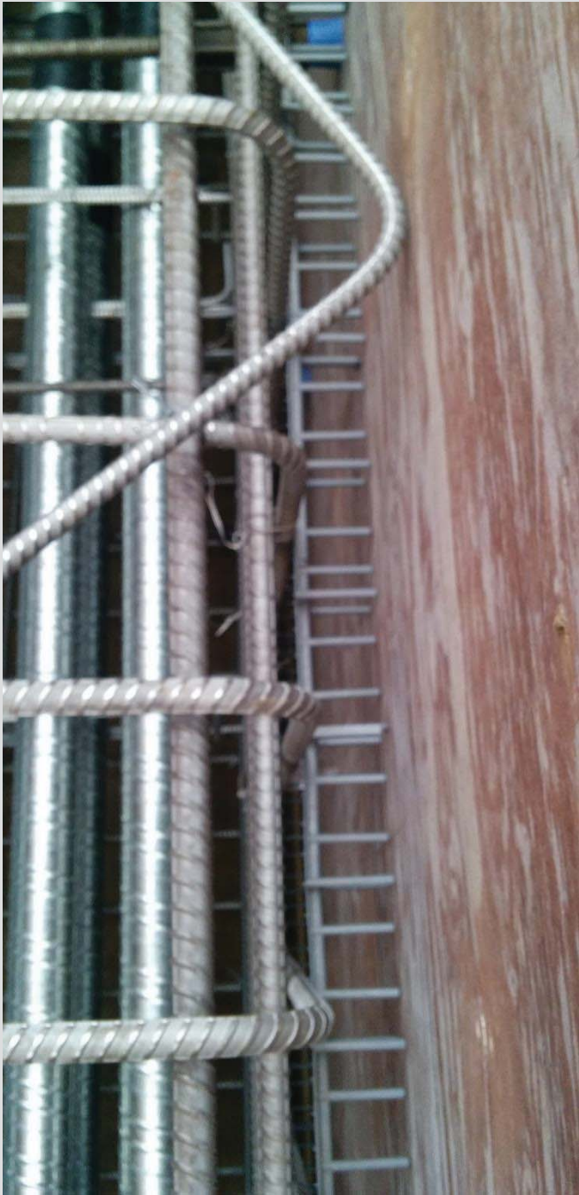
4.21 Plastic supports or chairs used to maintain required cover to edge of formwork.
