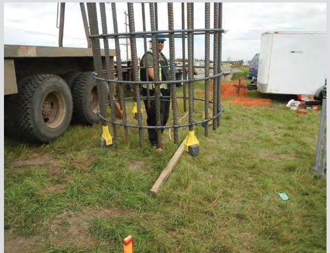
24.4 Plastic chairs used to maintain bottom cover and prevent cage form punching into ground at base.
