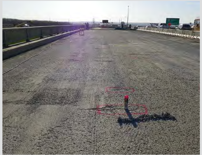
20.2 ACP removed and locations requiring full or partial depth repair are identified and marked out with paint by the inspector.
