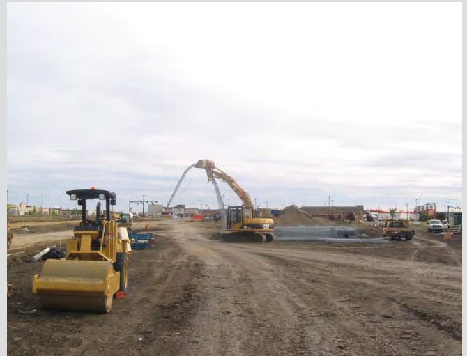
25.22 Poor handling of soil reinforcement. Fabric slings and spreader bar should be used.
