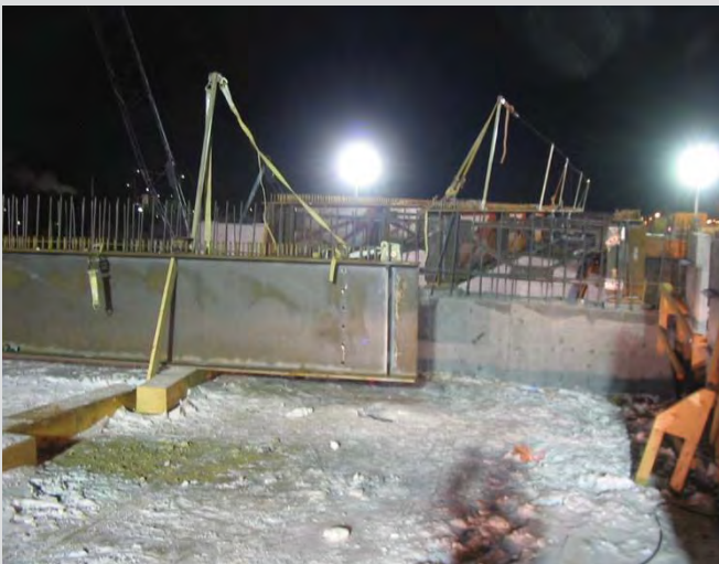
6.24 Fall protection system consisting of uprights and cables used during girder erection and deck overhang bracket installation.
