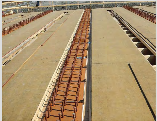
4.36 Joists and plywood are placed onto ledgers. Neat chamfers must separate the haunch and interior bay formwork. Holes through plywood to accommodate coil bolts must be properly sealed.
