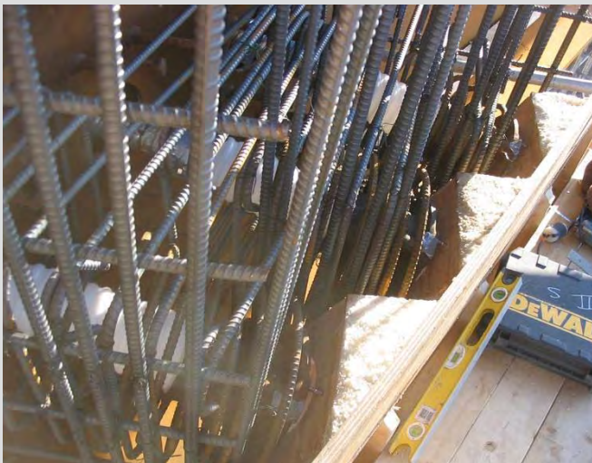
7.19 Post tensioning ducting in pier cap. Congested reinforcing steel exists at pier cap ends.
