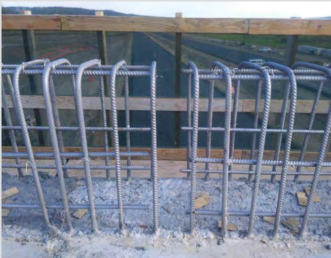
4.77 Typical gap at barrier reinforcing steel at control joint.
