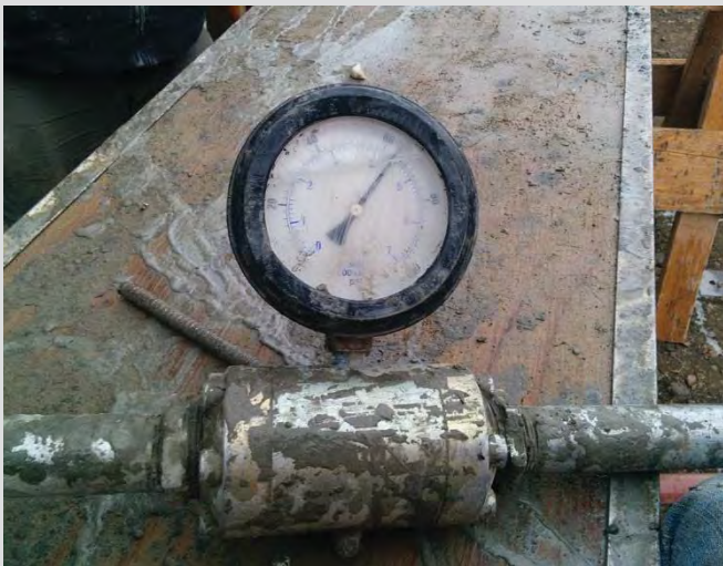
7.34 Grout pump pressure gauge.
