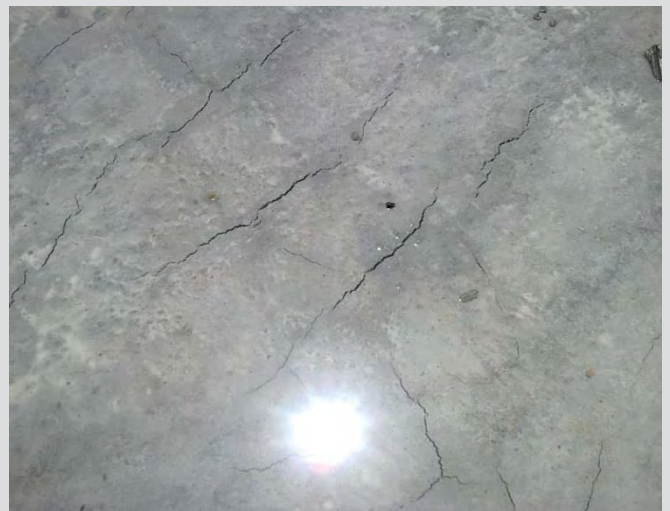
4.98 Plastic shrinkage cracks on deck slab surfaces.
