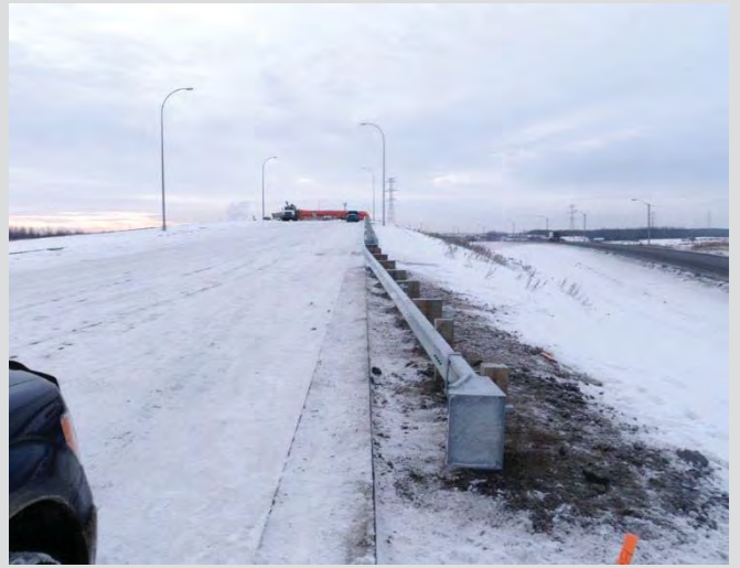
14.6 Guardrail and posts with end treatment.
