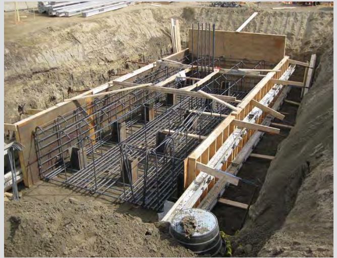
4.2 Pile cap partial formwork and reinforcing steel. Formwork braced from excavation walls.
