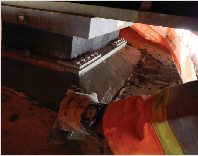
8.12 Trimming grout after form removal. Note that top of grout pad elevation is not higher than the underside of masonry plate elevation.
