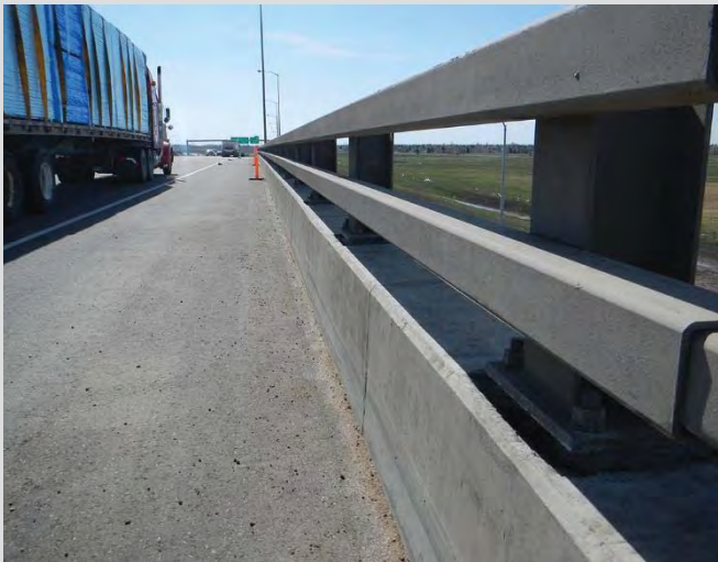
12.2 Bridgerail alignment and elevation adjusted prior to grouting. Alignment and elevation to required lines is important for overall functionality and appearance of the bridgerail.
