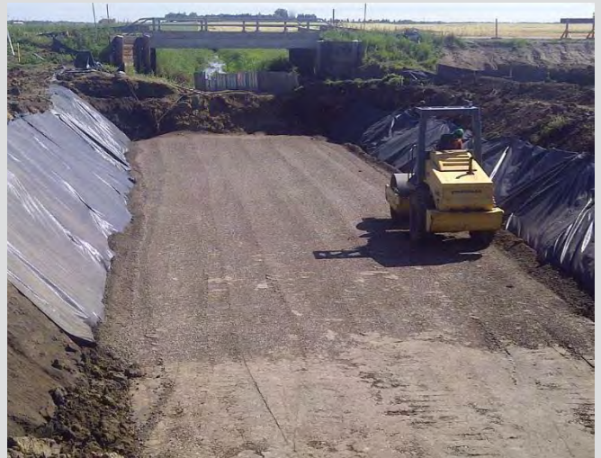
2.8 Smooth-drum roller compacting culvert bedding material. Geotextile and safe side slopes shown.
