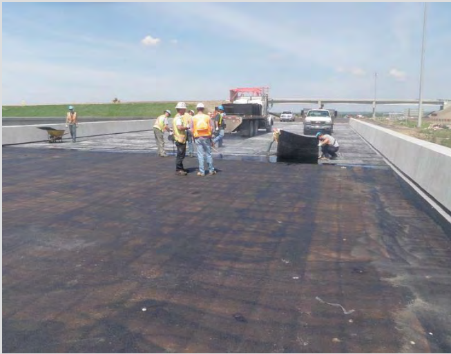
16.5 Tack coat on deck surface. Tack has changed from a dull black to a dull brown, indicating the tack coat has cured and is ready for the next stage.
