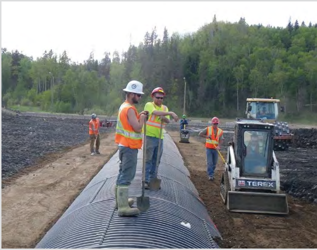
18.9 Backfilling of SPCSP. Small equipment only permitted to work within 1.0 m of pipe. Backfill progressing evenly on both sides of the pipe.
