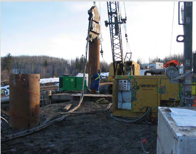
3.22 Vibratory hammer used to advance drilling casing. Worker checking if casing is plumb.
