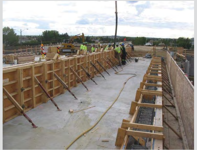
4.82 Wooden forms for barrier and curb formwork. Form attachment to deck concrete must be avoided.
