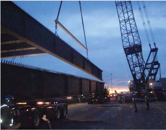
6.1 Steel girder delivery and erection. Spreader bar used for unloading and erecting girders when using a single crane.
