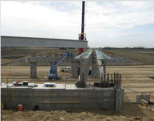
7.3 First girders erected and stabilized with temporary shoring and bracing. Short H-pile section bolted to the abutment to provide additional lateral stability at the bearing.
