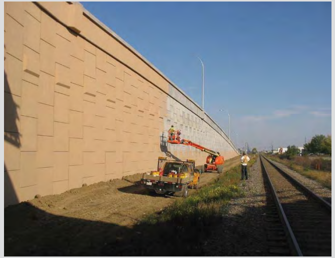
4.93 Applying pigmented sealer to MSE wall fascia panels and barriers by spraying.
