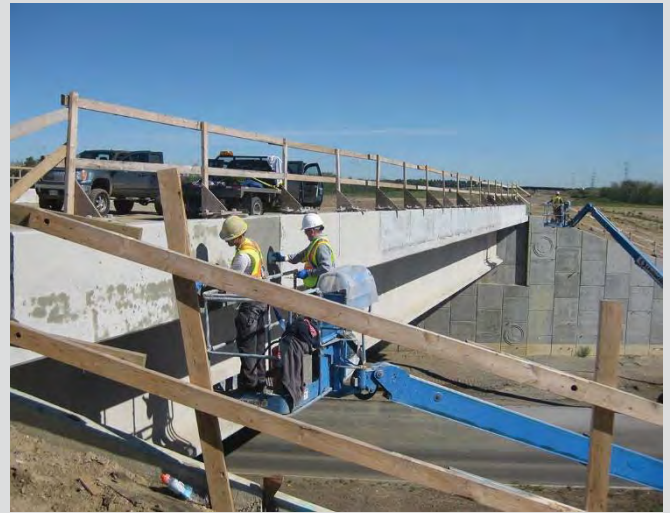
4.89 Concrete surface finishing at exterior faces of barriers. Workers using aerial work platform to access work. Class 2 rubbed surface finish followed by two applications of pigmented sealer.
