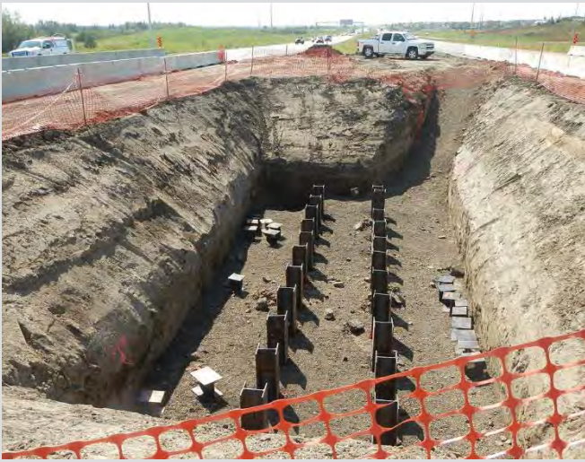
1.1 Pier excavation for pile cap. Piles cut off at elevation. Safe slopes and good access to excavation shown.
