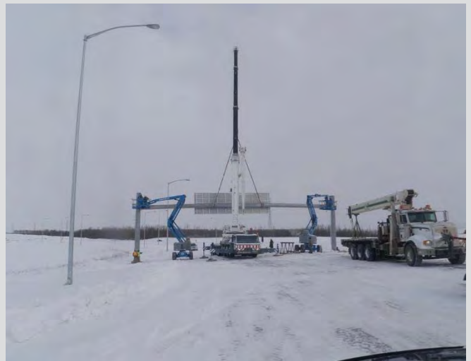
24.8 Sign structure erection. Workers tightening bolts to connect horizontal and vertical columns using aerial lifts.
