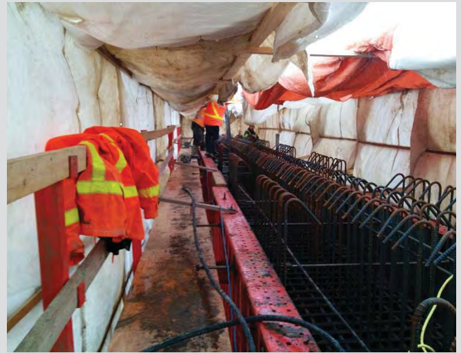
4.32 Cold weather concreting. Hoarding for pier cap pour. Room for workers and equipment to work within the enclosure. Roof tarps open to allow for concrete pump access.
