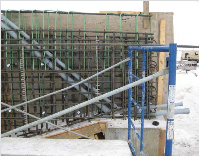
11.5 Electrical ducts exiting bottom of wingwall below grade.
