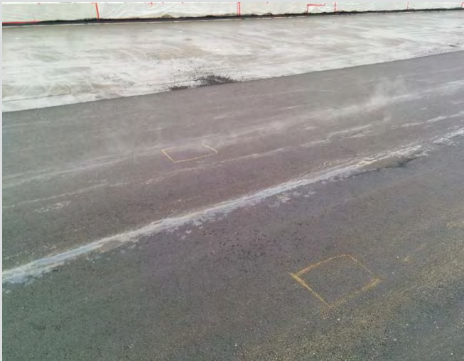
17.7 Control strip method used to determine maximum density. Location for nuclear densometer marked for consistent testing.
