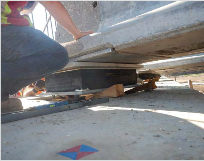
7.13 Setting NU girder onto bearing. Survey layout/control visibly marked on abutment seat.
