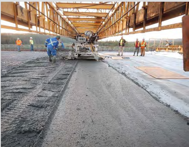
4.61 It is important that concrete be screeded and raked before consolidation. Workers must not walk through or place additional concrete at locations where vibration has already taken place.
