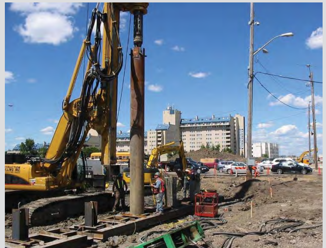
3.23 Drilling rig used to advance drilling casing. Kelly bar advances the casing into the excavation. For larger diameters, a vibratory hammer or an oscillator is used to advance the casing.
