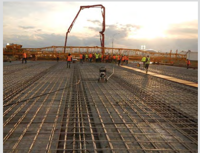
4.54 Start of deck pour. Plywood walkway on deck reinforcing steel for safety and protection of reinforcing steel. Pressure sprayer for cleaning and wetting deck.
