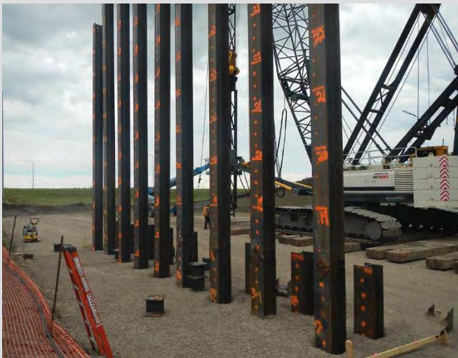
3.7 Pile driving at abutment seat location. Piles are marked at 250 mm intervals.
