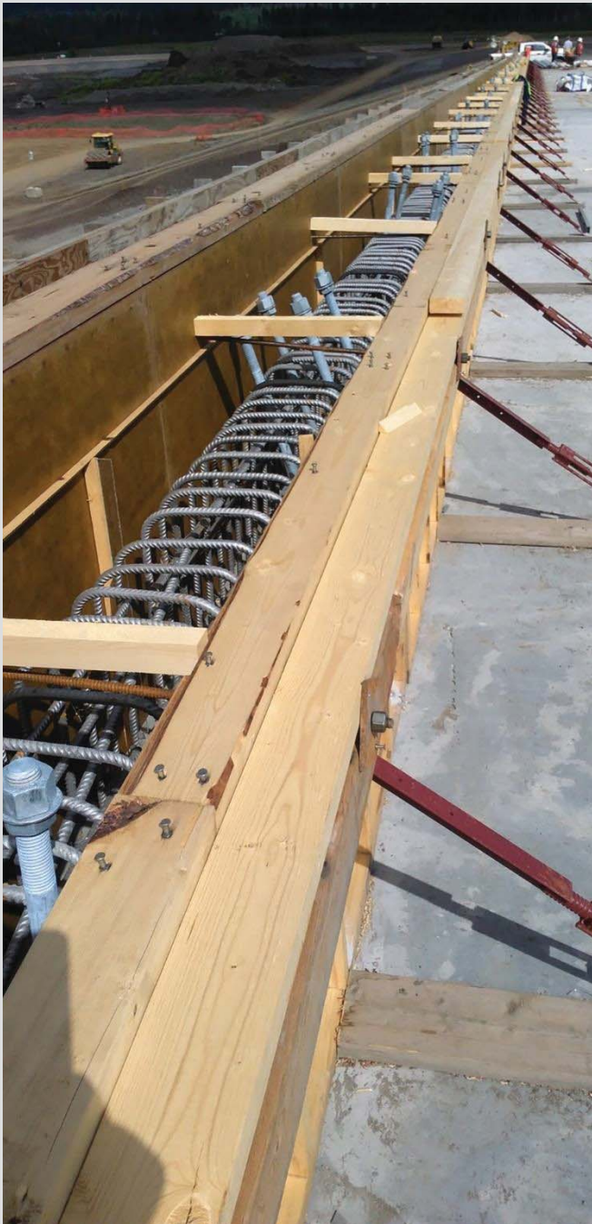
4.80 Barrier formwork showing anchor bolt assemblies, chamfer strip, and control joint crack initiator.
