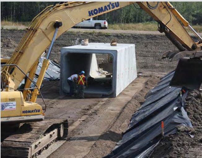
26.15 Installation of PCB units onto prepared bed, using string for alignment control.
