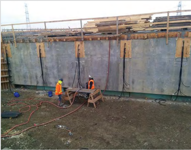
7.32 Workers open and close bleed tubes as instructed by the post-tensioning supervisor.
