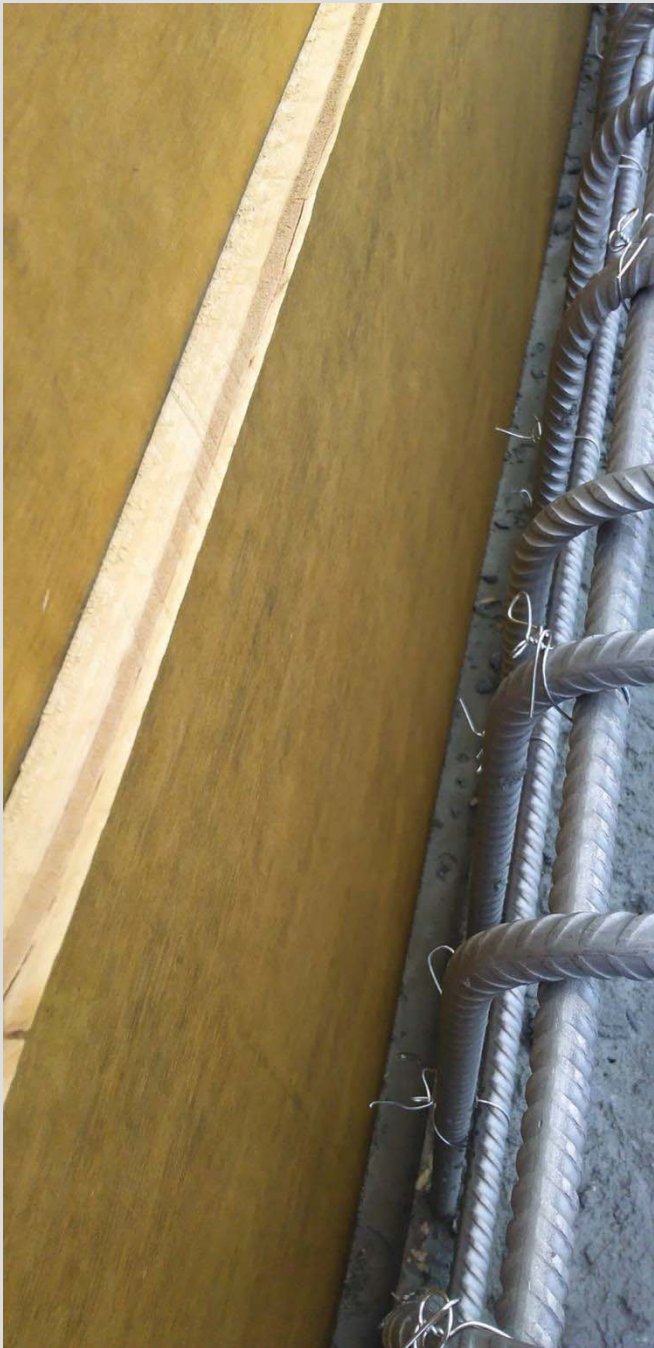
4.83 Typical formwork and pour strip at outside face of barrier. Note that forms are tight to the hardened concrete to prevent paste leakage.
