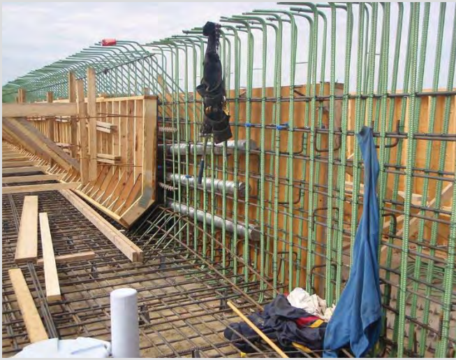
7.17 Cast-in-place girders with post tensioning ducts. U-bars set at 1.0 m spacing to secure duct elevations.
