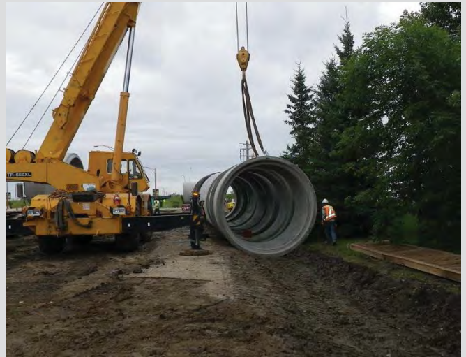
26.4 Crews unloading RCP. RCP lifted with slings from truck bed. Small swale dug at unloading area.
