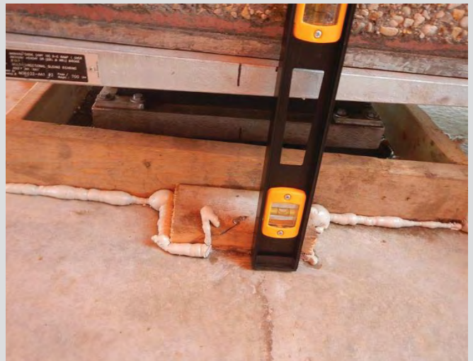
8.22 Setting bearing offset to "X" value in accordance with bearing temperature chart, just prior to grouting.
