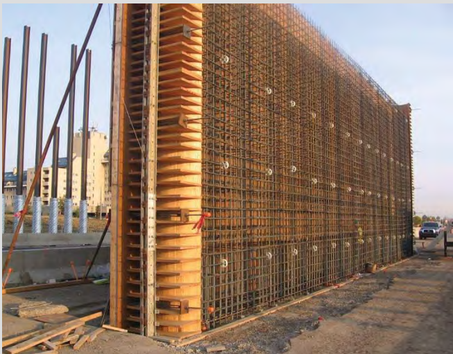
5.7 Pier shaft plain reinforcing steel. 50 mm wagon wheel chairs attached at open face.
