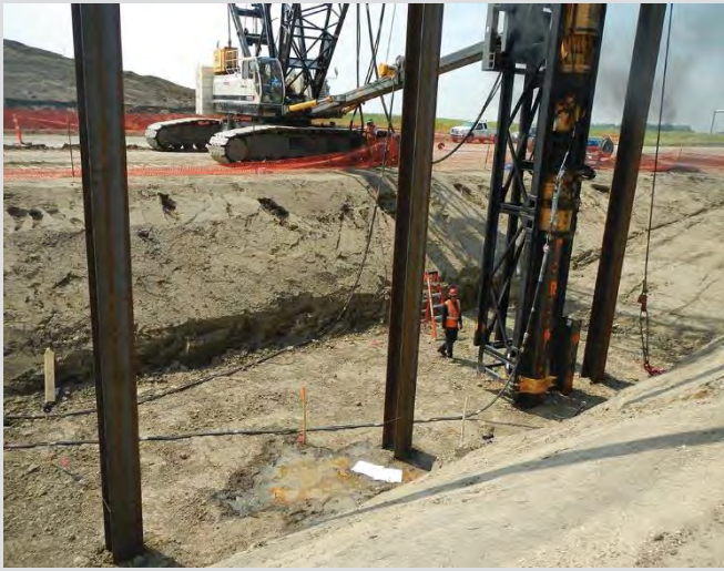
3.5 Diesel hammer piling rig shown. Centre of pile marked out by pins or flags. H-pile orientation painted on ground.
