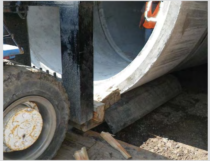
26.10 Joining RCP sections. Typically done with chucks or winches. Rubber softeners and 2x6 blocks used here to lift and push pipe.
