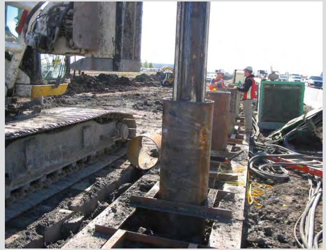
3.21 Drilling pile holes with casing installed. Casing is used temporarily to keep the excavation from caving in, or to stop seepage. Casing is removed during concrete placement.
