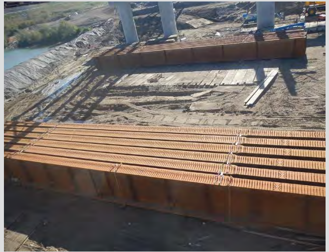
6.2 Girders stored at bridge site. Storage of girders is on timber dunnage and free-draining ground.
