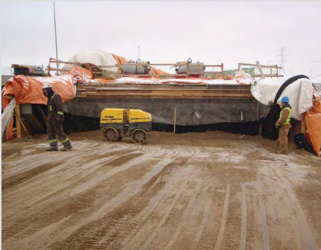
2.3 Compaction of granular backfill behind abutment diaphragm and wingwalls using walk behind remote controlled compaction equipment.
