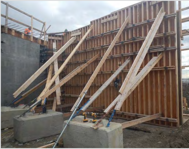
4.8 Formwork bracing for wingwall. Waler form construction used. Forms braced using deadman lock-block anchors.
