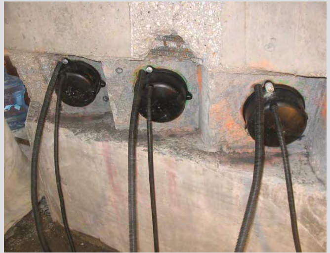
7.29 Tendons cut and capped, ready for grouting. Grout flow tubes protruding from cap.
