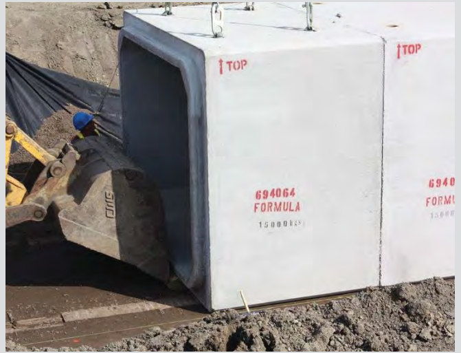
26.18 Positioning of PCB unit. Hydraulic excavator bucket is positioning unit with timber cushion.
