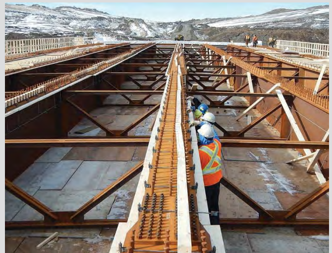
4.34 Timber deck formwork is typically hung from coil bolt hangers supported on girder top flanges. False deck working surface shown.
