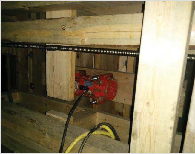
4.27 External vibrator attached to form. Due to congestion of reinforcing steel and post-tensioning ducts, internal vibration difficult.
