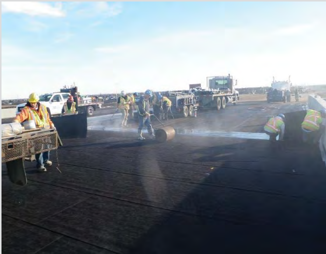
16.11 Protection board is rolled with a water-filled garden roller before membrane cools.
