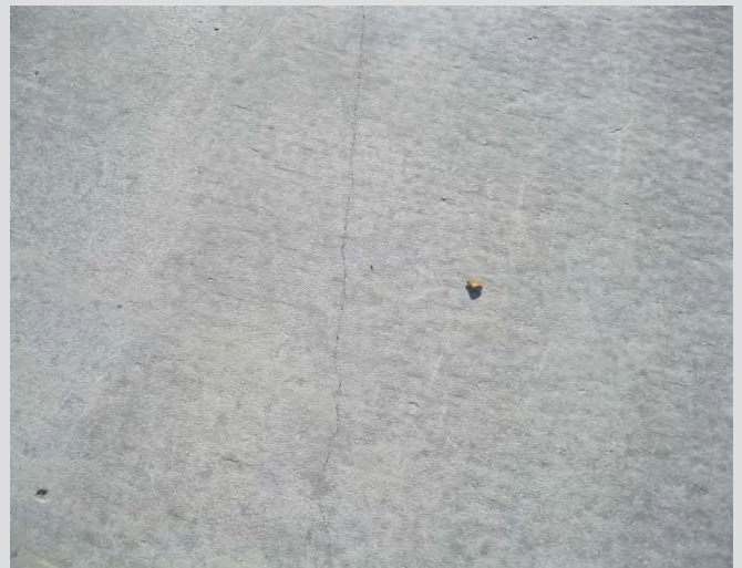
4.96 Transverse-direction deck slab drying shrinkage crack.
