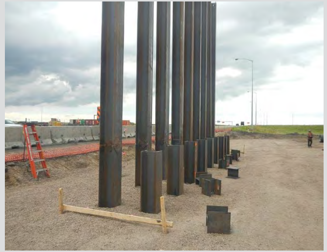
3.6 Batterboards and string line set up with 2x4s. String line offset to re-establish pile location.
