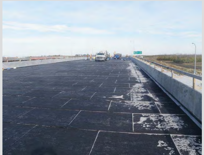
16.12 Waterproofing complete. Clean up of sand and debris from protection board required before tack coat for ACP. Joints and laps in protection boards shown.
