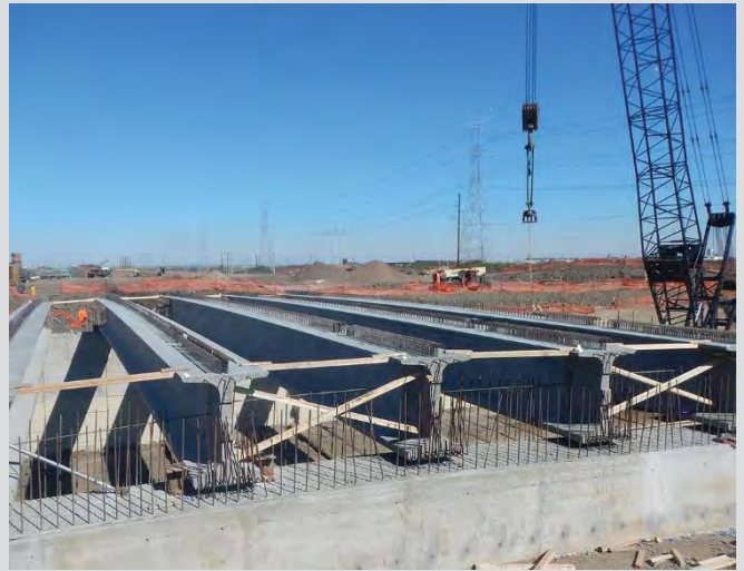
7.6 Subsequent girders erected, stabilized with temporary bracing until installation of steel diaphragms is completed.
