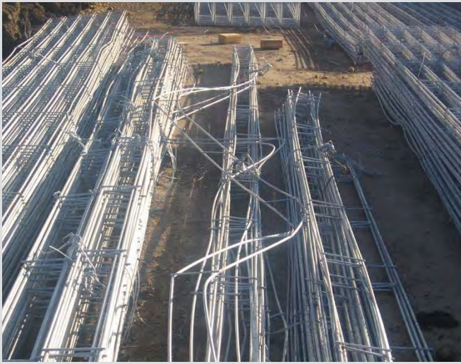
25.23 Damaged soil reinforcement.
