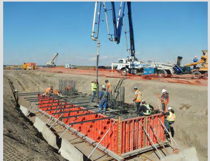
4.19 Concrete pump used for pile cap pour. Forms braced against precast concrete deadmen.
