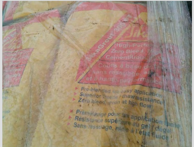
7.39 Approved grout product stored on site. Expiration dates need to be labelled on package.
