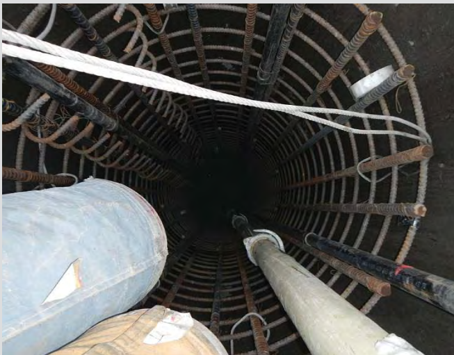
3.34 Concrete pumped through tremmie pipe. Cross-hole Sonic Log (CSL) pipe attached to reinforcing steel (black pipes).
