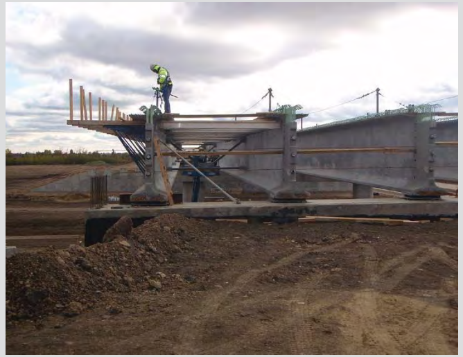
7.14 Installing deck overhangs and galvanized cross bracing. Fall protection system is in place.
