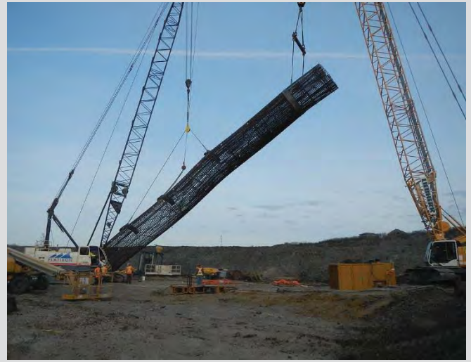
3.41 Double crane pick for reinforcing steel cage installation. Halo ring and extra reinforcement required to pick large cage.
