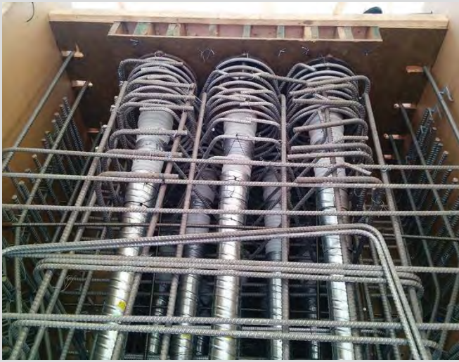
7.21 Post tensioning duct anchors in straddlebeamb. Congested reinforcing steel at pier cap ends.
