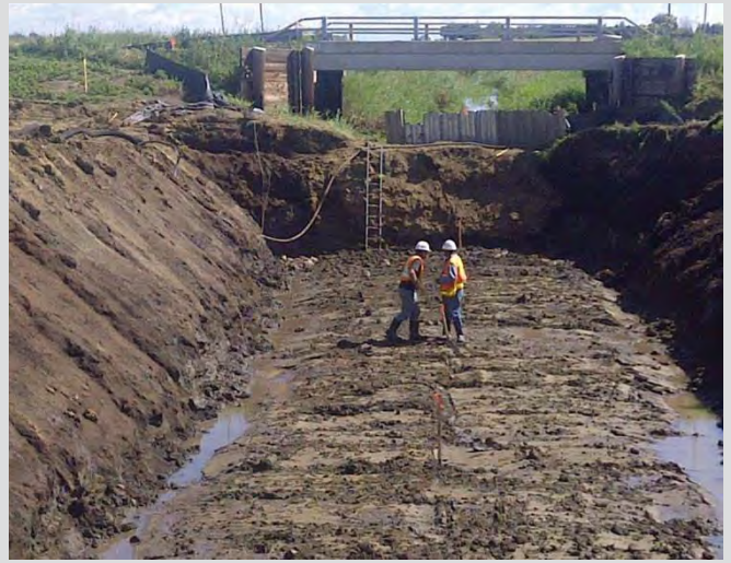
1.2 Channel excavation for culvert construction. Channel bed crowned and graded to shed water. Existing stream diverted with sheet piling and clay berm. Slopes cut at 1:1 for safety.
