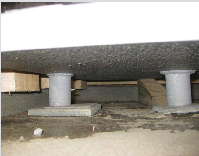
8.7 Bearing elevation set using shim stacks placed under pintles. Pintles allow bearing to rotate. Underside of plate is coated to prevent direct contact between zinc and grout.
