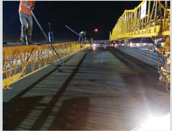
4.60 Concrete finishers bull floating concrete deck immediately after screeding. Finishing done from work bridges.
