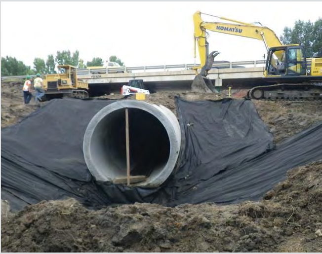
26.13 Clay seal compacted at end of pipe. Filter fabric material in place.
