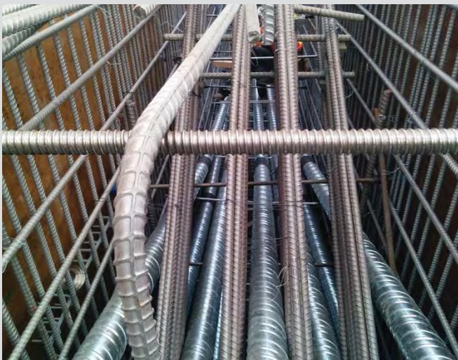
7.22 Post tensioning ducts at pier cap. Smooth profile throughout length of tendon.
