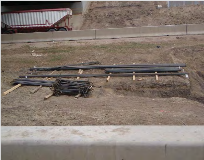
5.1 Proper storage of plain reinforcing steel on timber dunnage in dry location.
