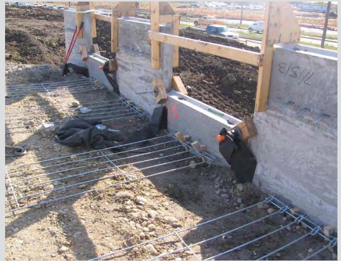
25.10 Wooden wedges used to engage panels. Filter fabric placed over panel joints to prevent loss of material through gaps.
