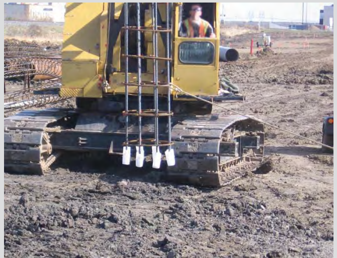
3.31 Plastic spacer chairs attached to bottom of reinforcing steel cage to prevent the cage from punching through the base of the excavation.
