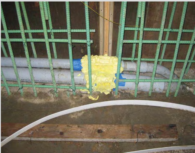
11.7 Improper connection at expansion joint using expanding foam.
