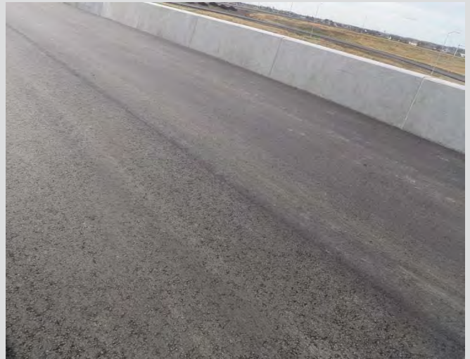
17.12 Unacceptable segregation in travel lanes.
