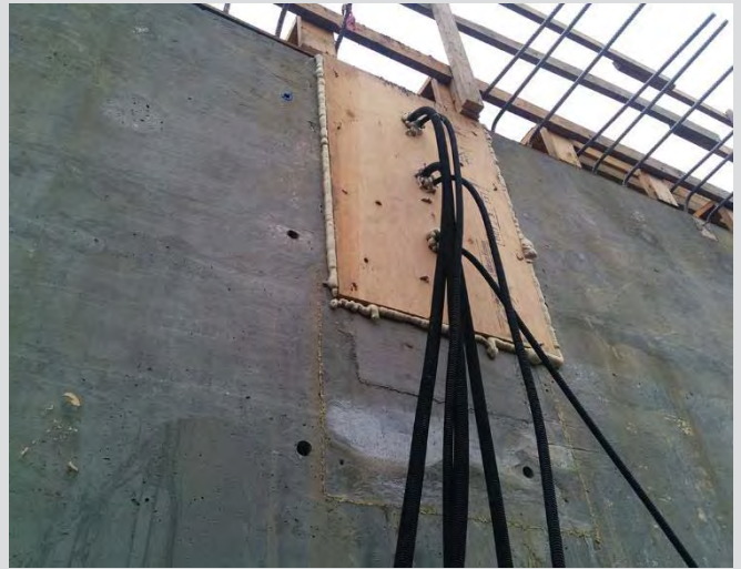
7.33 Diaphragm end ready for grout. Blockout formwork is sealed to prevent grout leakage.
