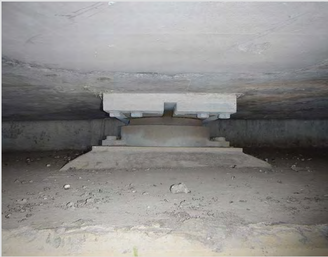
8.19 Grout pad constructed at 45 degree slope from abutment seat to bottom of base plate.
