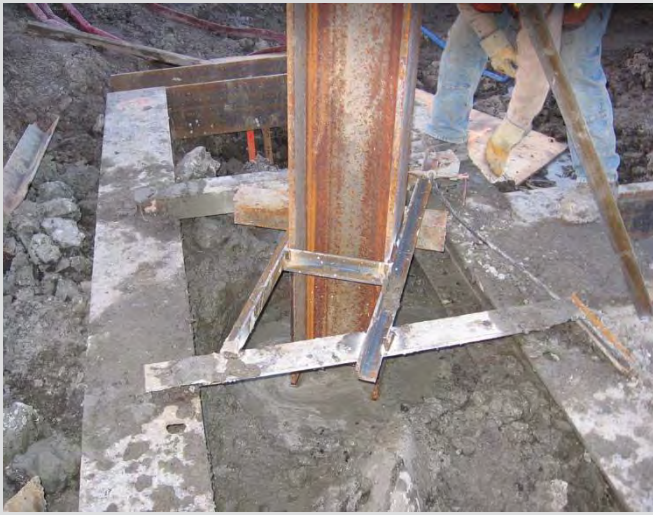
3.36 H-pile set into centre of concrete pile. Steel frame used to set location and elevation.
