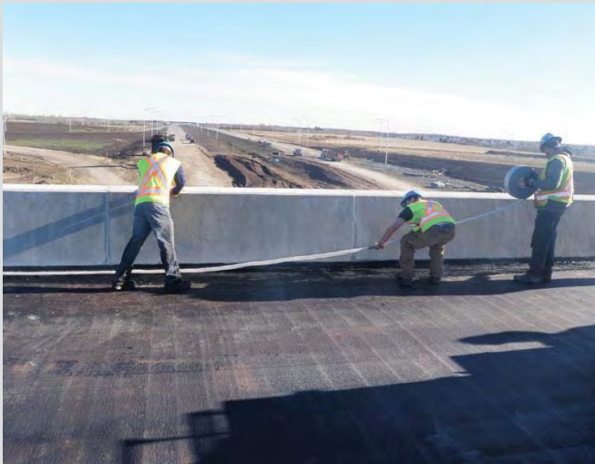
16.7 Wick drain placement along edges of barriers. Wick drains are installed over the asphalt membrane while it is still tacky. Protection boards are not placed over wick drains.
