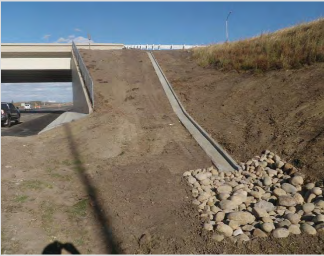
9.1 Riprap drain trough terminal protection.
