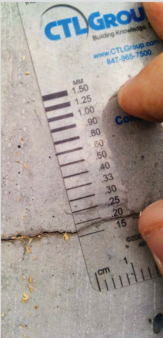
4.97 Crack comparator gauge used to measure crack width.
