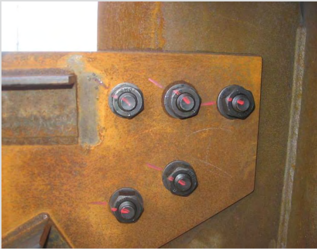
6.9 Bolting of diaphragms. Bolts presently in snug tight position. Tightening of bolts to be done by turn-of-nut method. Bolt markings shown prior to tightening.
