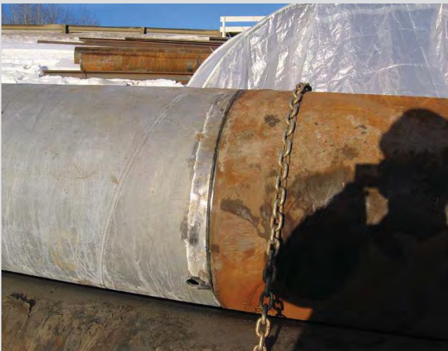
3.26 Splicing of galvanized and plain pipe piles. Galvanized pipe piles used above grade.
