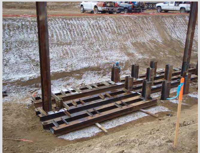
3.4 Pile driving frame used to position piles accurately at the start of driving. Frame is anchored by welding to soldier piles.
