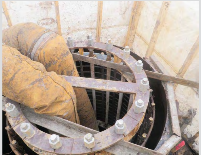
24.6 Anchor rod assembly installed. Angle iron on formwork to hold anchor rod assembly at correct elevation.
