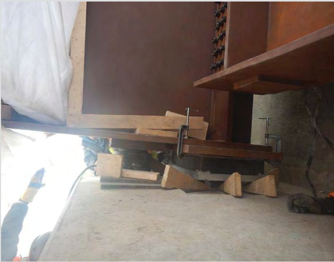
6.26 Setting elastomeric bearing. Wood wedges used to adjust and secure the bearing until girder is in place.
