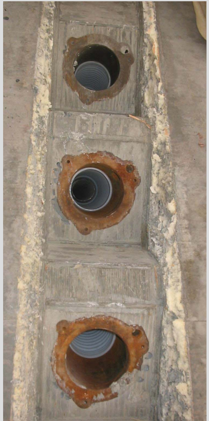
7.23 Post tensioning ducts cast into pier cap. Tendons to be installed, stressed and grouted.
