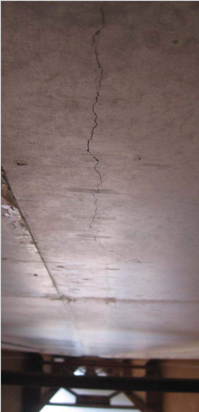
4.99 Deck slab soffit drying shrinkage crack.
