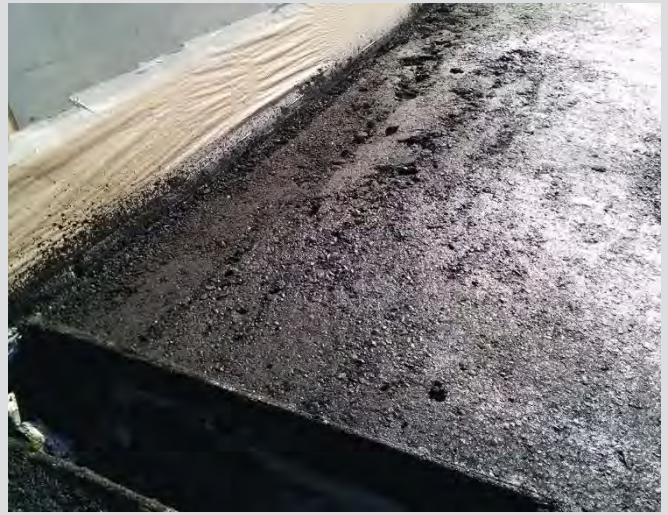
17.10 Unacceptable segregation near barrier face.
