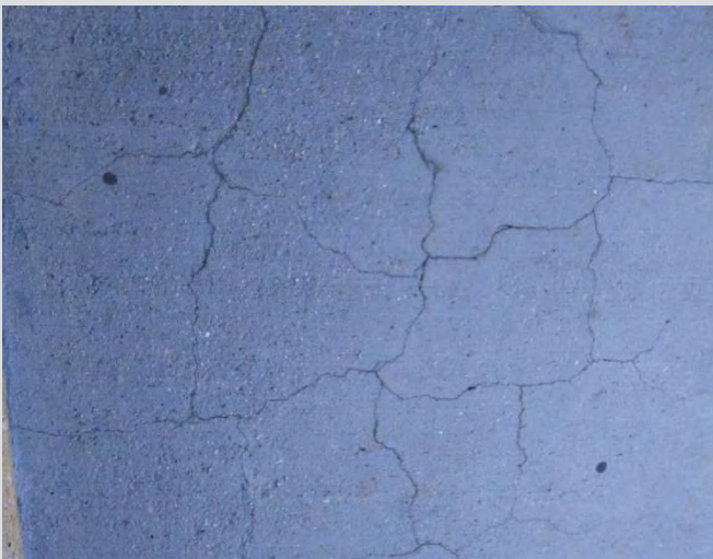
4.103 Drying shrinkage cracks on substructure.
