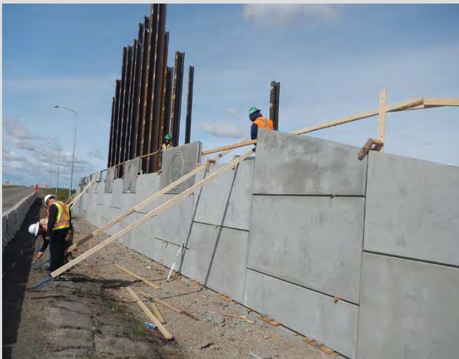
25.7 Panels set at batter. Turnbuckle on bracing used to set batter. Panels clamped together at edges to maintain alignment.
