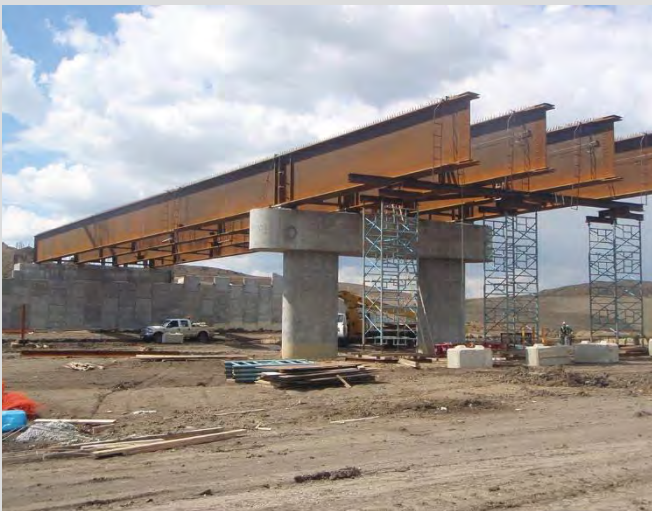
6.3 Girder erection. Scaffolding shoring towers used at splice connection between girder segments.
