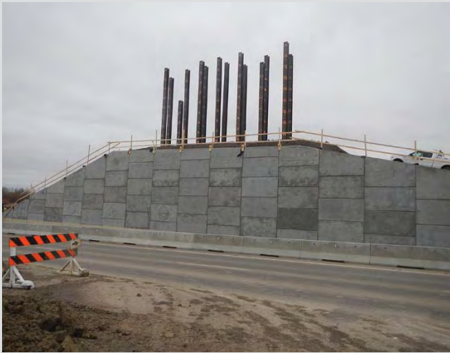
25.16 Completed backfilling and panel installation. Panels require cleaning prior to application of pigmented sealer.
