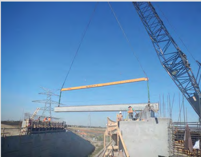
7.7 Erecting concrete box girders from approach fill, using a spreader bar to achieve vertical forces at lifting points.
