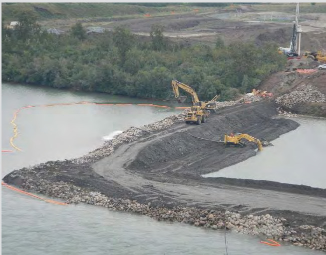
1.7 River berm construction. Infill material and riprap being placed, pumping out water from work area.
