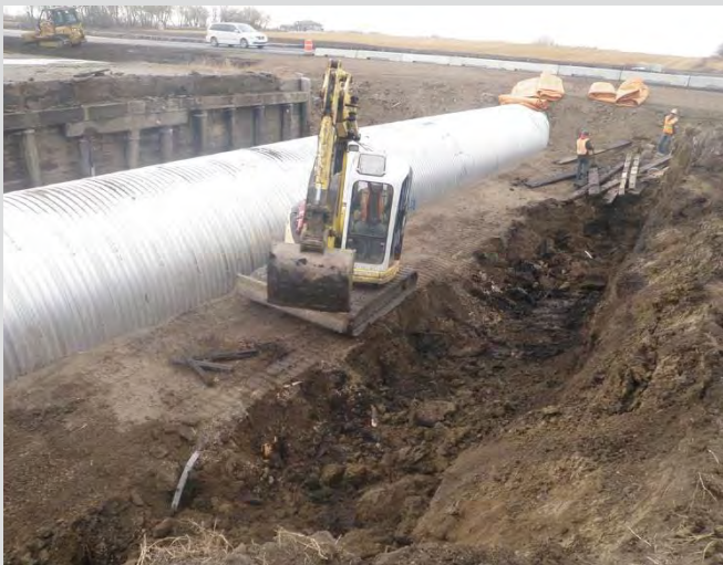
18.19 Removal of existing bridge structure. Abutment piles removed to specified depth below streambed.
