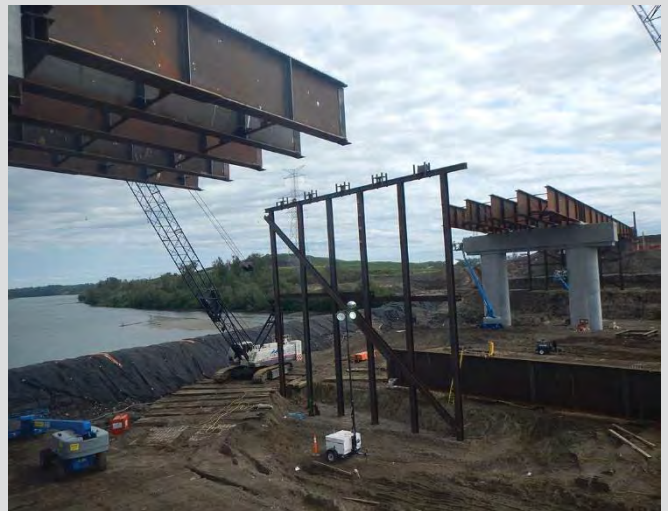
6.4 Girder erection. H-pile shoring towers used to support girders at splice connection between girder segments.
