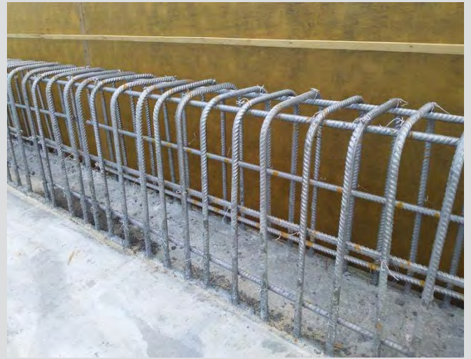
4.79 Typical rough vibrator-finish at barrier construction joint. Note that concrete surface at construction joint slopes towards deck and away from outside face of barrier.
