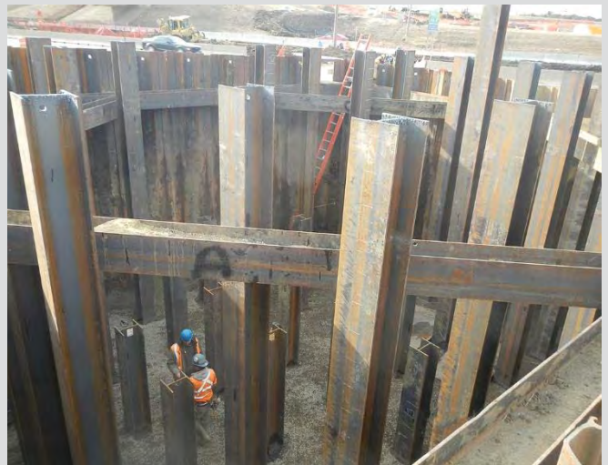
1.4 Sheet piling installed for pier piling cofferdam. H piles placed horizontally as bracing. Ladder access to excavation.
