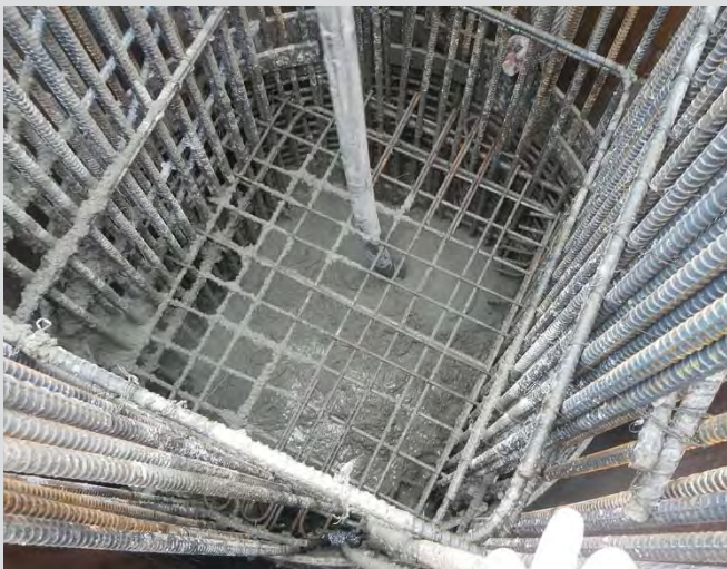
3.42 Concrete discharge down centre of pile by pump. Pump hose centred so that concrete does not impact reinforcing steel.
