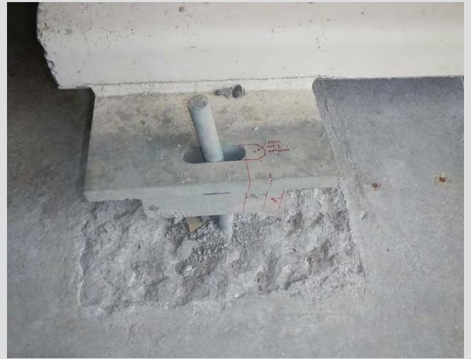
8.16 Improperly set bearing resulting in bent anchor rods and failed grout pad.
