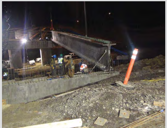
7.4 First girder erected, stabilized with temporary shoring and braced to the abutment seat.
