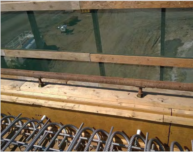
4.47 Finishing machine screed rail cups are installed and rail is set by instrument to the design gradeline.
