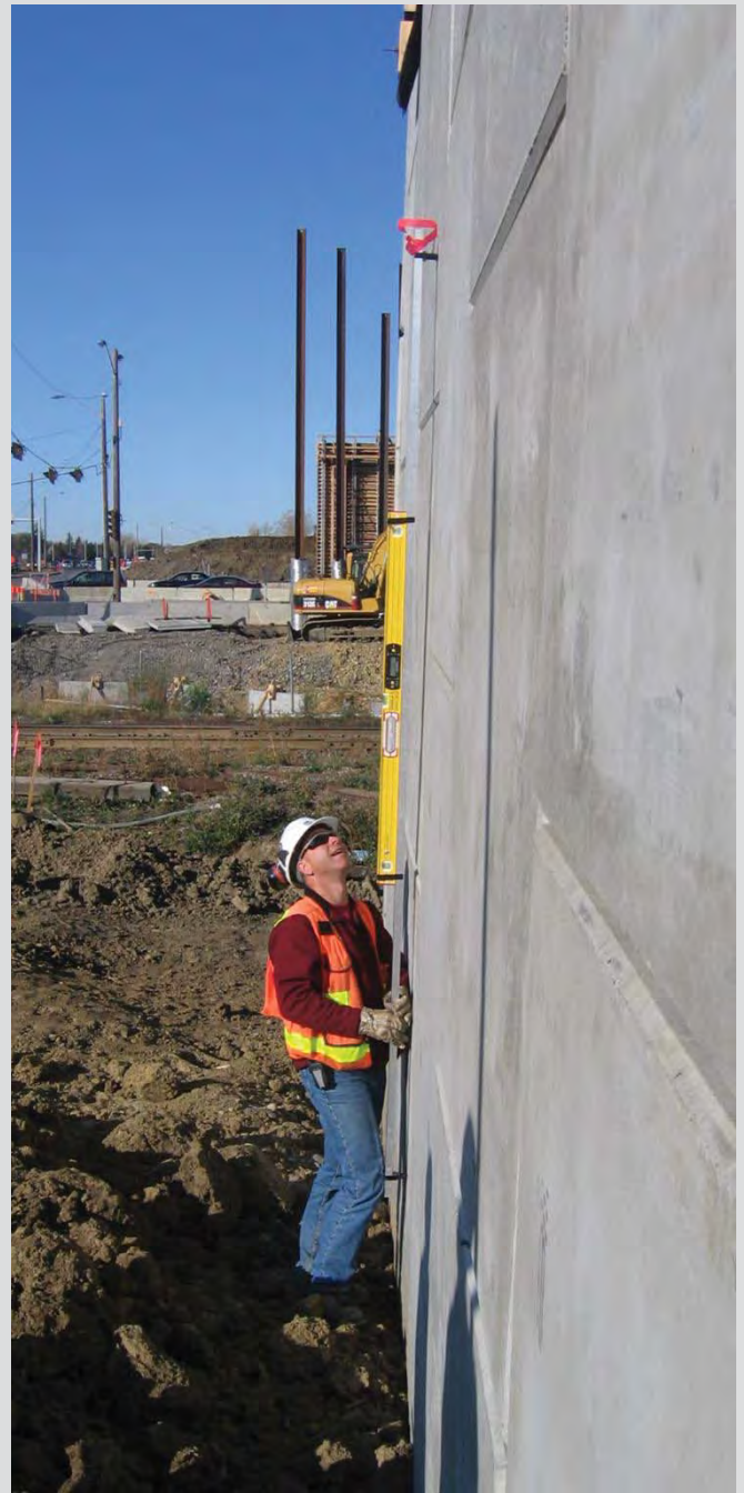
25.15 Checking wall batter and panel alignment with digital level and 3.0 m straight edge.
