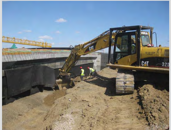
2.4 Hydraulic excavator placing granular backfill material against abutment backwall. Sheet drain placed against abutment seat.
