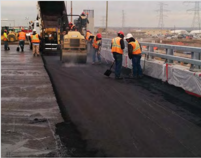
17.5 Placing first lift of ACP. Small smooth drum roller following as soon as practical.
