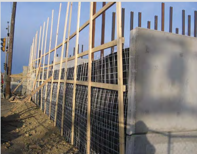
25.14 Two stage wall construction. Backfilling against wire wall. Fascia panels not in contact with fill.
