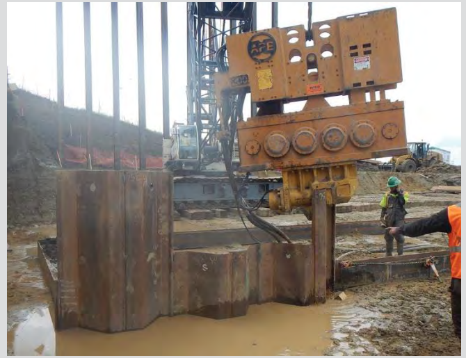
1.13 Sheet piling and frame for pier offerdam. Vibratory hammer advancing sections of sheet piling.
