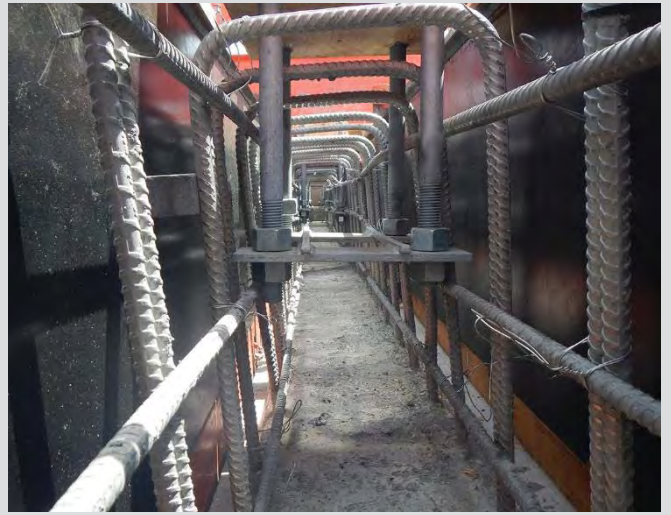
4.76 Barrier reinforcing steel and formwork. Bridge rail anchor bolt assembly secured to reinforcing steel.
