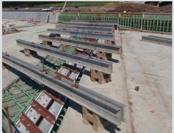
6.12 Deck joint installation. Deck joint gap set in accordance with the "Expansion Gap Setting Table" found in the design drawings.
