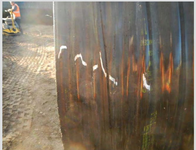
18.36 Damage to polymer coated CSP structure. Special adhesive tape or approved brush on coating is required.
