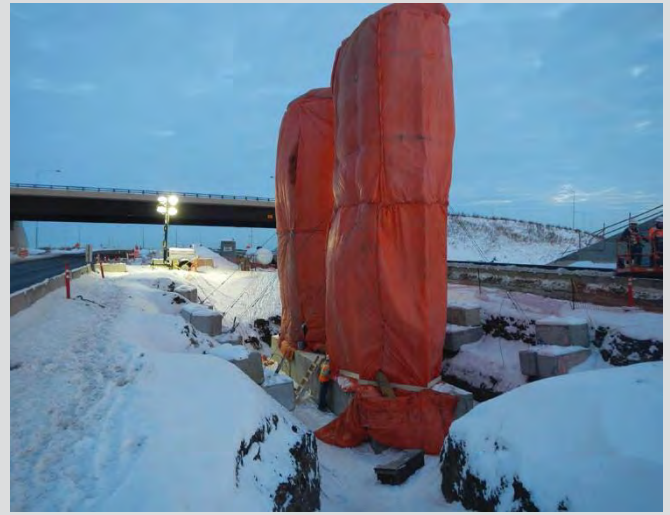
4.28 Cold weather concreting. Hoarding for pier columns consists of insulated tarps and heaters.
