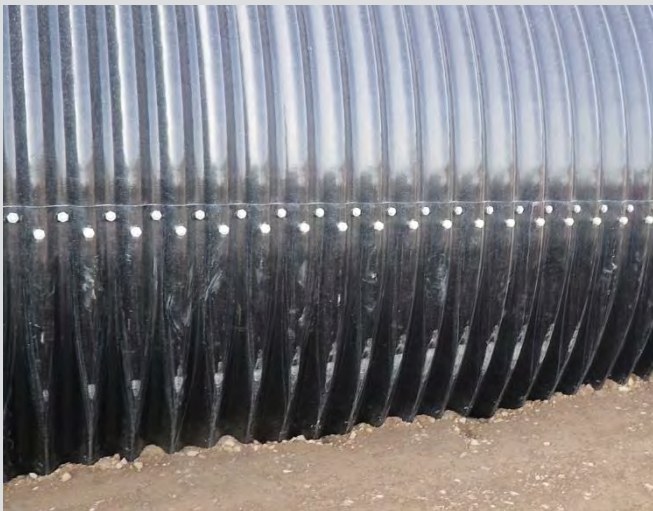
18.7 SPCSP showing that bolts in the valley of each longitudinal seam are nearer to the visible edge of the plate than the bolts in the crest.
