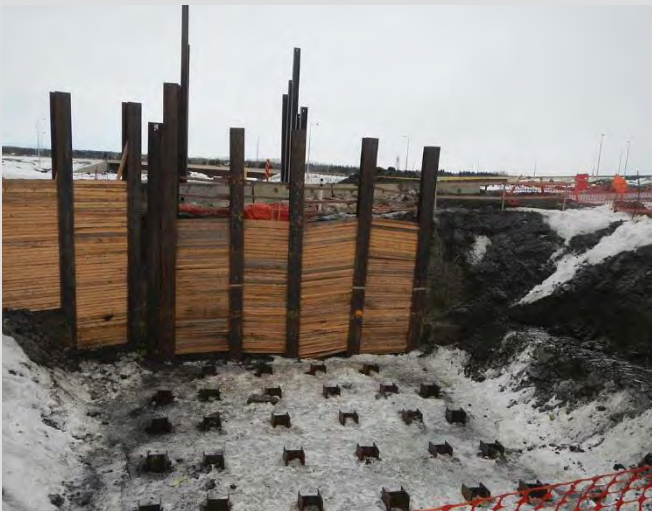
1.3 Pier excavation for pile cap. Piles cut off at elevation. H-piles and lagging for temporary retaining wall shown.
