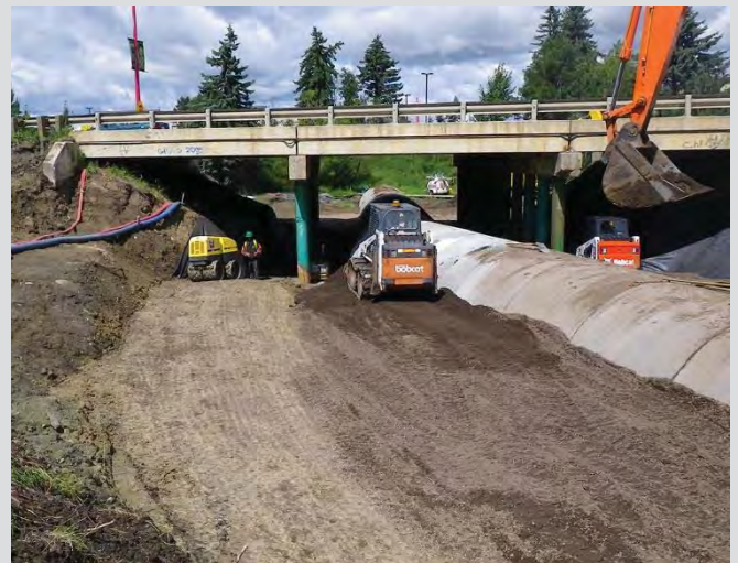
26.12 Both sides of pipe simultaneously backfilled. Skid steer and remote controlled walk behind packer used to compact material.
