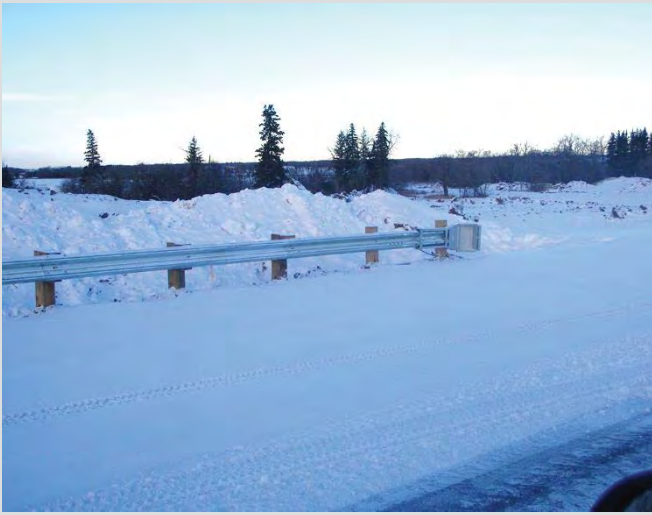
14.5 Guardrail and posts with end treatment.
