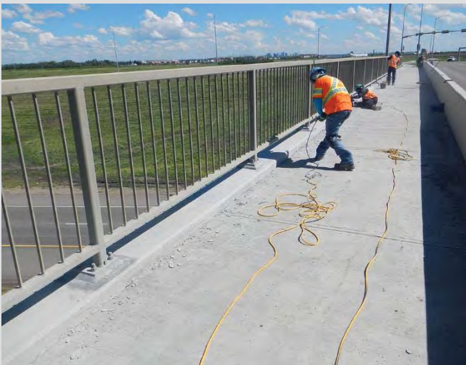
12.6 Sidewalk pedestrian rail. Horizontal and vertical alignment is important for the overall appearance.
