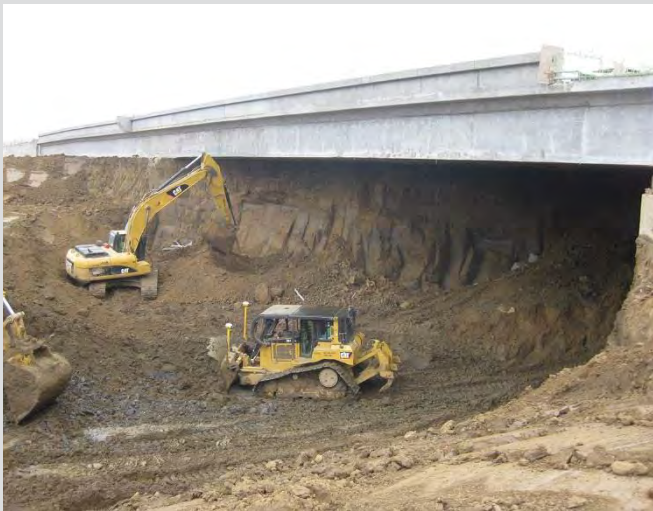
1.10 Cast-in-place concrete bridge constructed on existing grade. Excavation of roadway beneath, after superstructure is cast.
