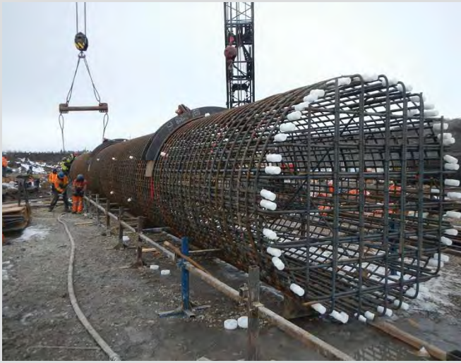
3.40 Large 3.0 m diameter pre-fabricated cage. Extra support / bracing used to retain shape and stability for lifting.
