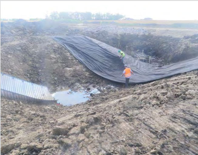
10.3 Crews placing filter fabric material prior to heavy rock riprap placement. Filter fabric keyed into top of slope.
