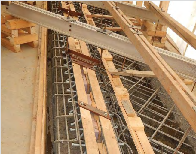
6.13 Deck joint installation. Deck joint gap set in accordance with the “Expansion Gap Setting Table” found in the design drawings. Erection angles left in place to maintain the required gap.
