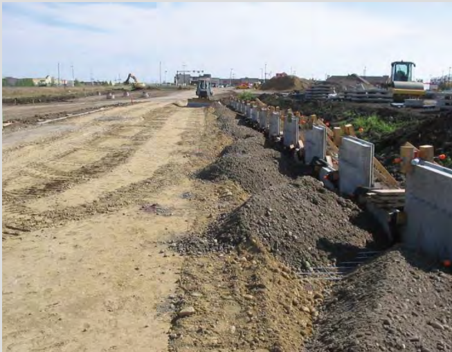
25.11 Two types of backfill material placed. Drainage layer backfill material placed within 1.5m of back face of wall.
