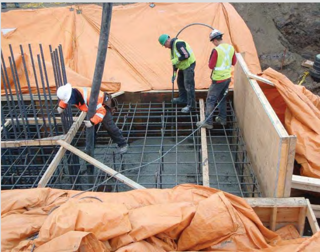
4.18 Substructure concrete placement. Long vibrator used to consolidate concrete for deep elements.
