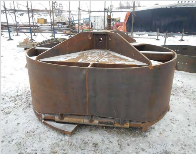
3.17 Large muck or slush bucket, used to clean out the bottom of wet or muddy holes prior to cage placement.
