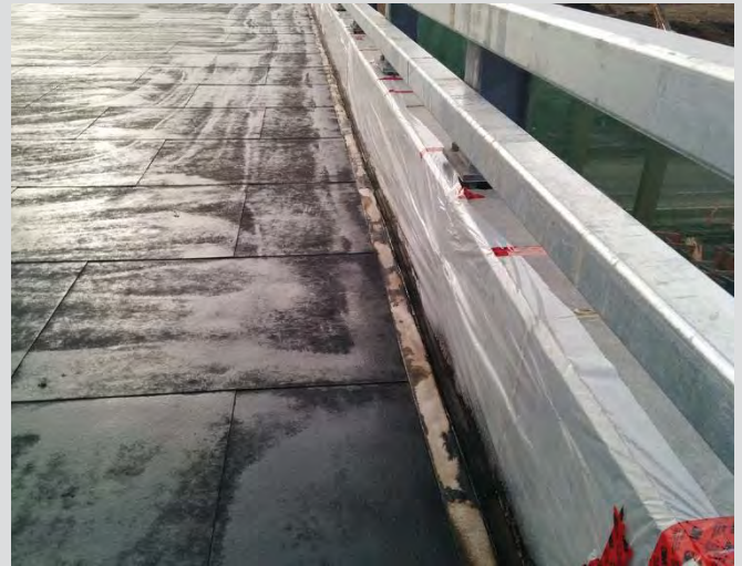
17.4 Wick drain and barriers protected from tack spray. Plastic strip placed over wick drain, and barriers covered with poly during spraying of tack coat.
