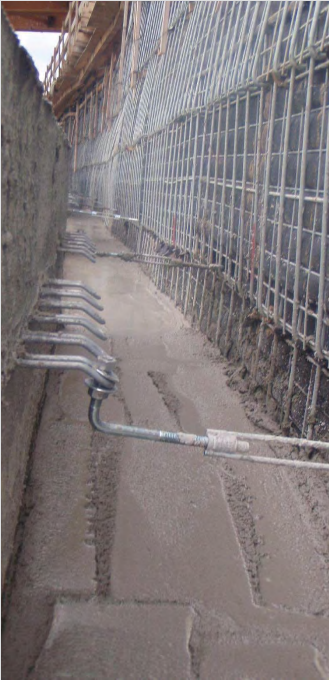
25.30 Space between 1 st and 2 nd stage. Panel anchorages shown.
