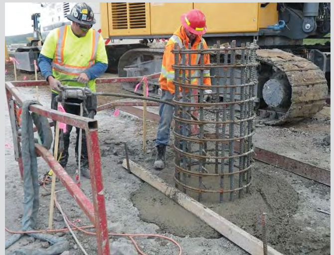
3.35 Vibrating top of pile. Efforts should be made to keep reinforcing steel free of paste.
