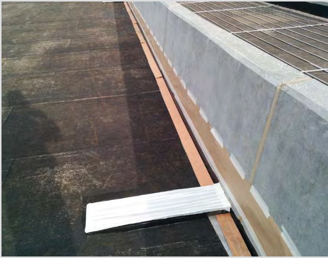
17.1 Protection of deck drain and barriers prior to tack coat and ACP placement.
