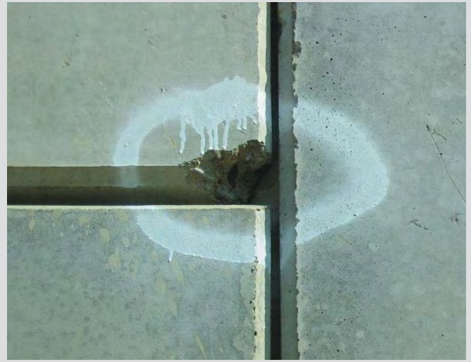
25.20 Panel damaged during erection.
