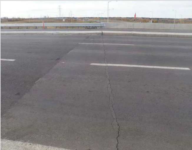
17.11 Cracking at approach slab transition.
