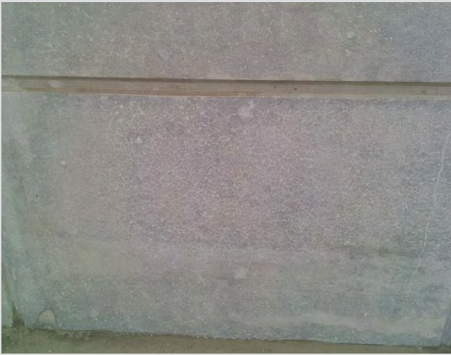
4.101 Crazing -type cracking seen on formed surfaces.
