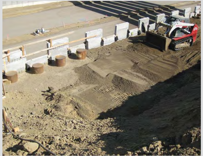
2.6 Skid steer loader used to spread 150 mm granular fill for MSE wall fill.
