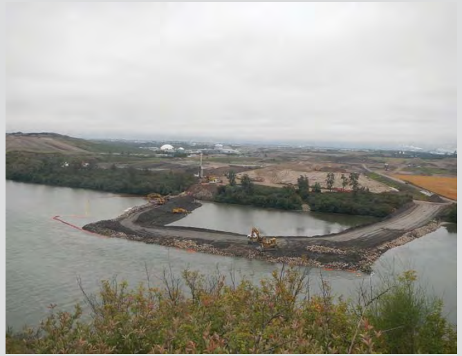
1.6 River berm construction. Perimeter placed first to isolate the work area. Riprap being placed for scour control.
