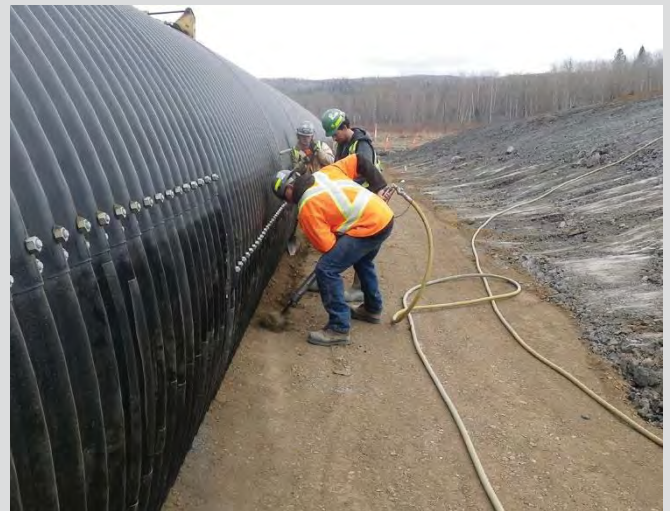
18.8 Compacting haunch area with pogo stick. Shovels and small equipment are also used to fill all corrugations.
