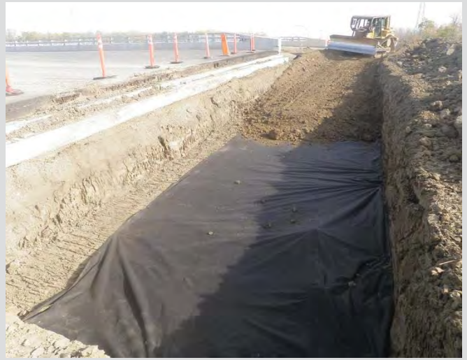
2.2 Soft soil at base of excavation removed and replaced with competent granular back fill.
