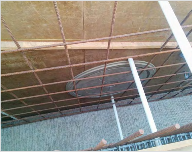
4.16 Wingwall formwork and plain steel reinforcement. Aesthetic enhancement motif cast into exterior face of wingwall.
