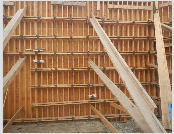
4.9 Formwork and bracing for wingwall. Full sheets of plywood used to reduce form lines.
