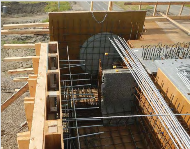
4.10 Abutment diaphragm formwork and reinforcing steel. Aesthetic enhancement motif cast into exterior face of diaphragm.
