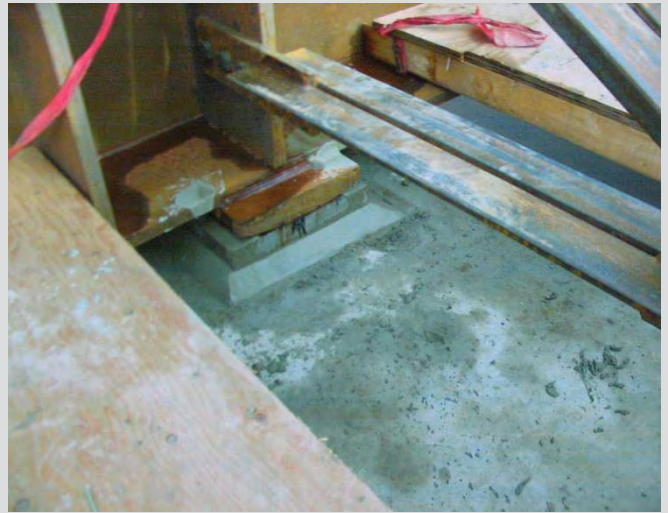
8.20 Grout pad constructed at 45 degree slope from abutment seat to bottom of base plate.
