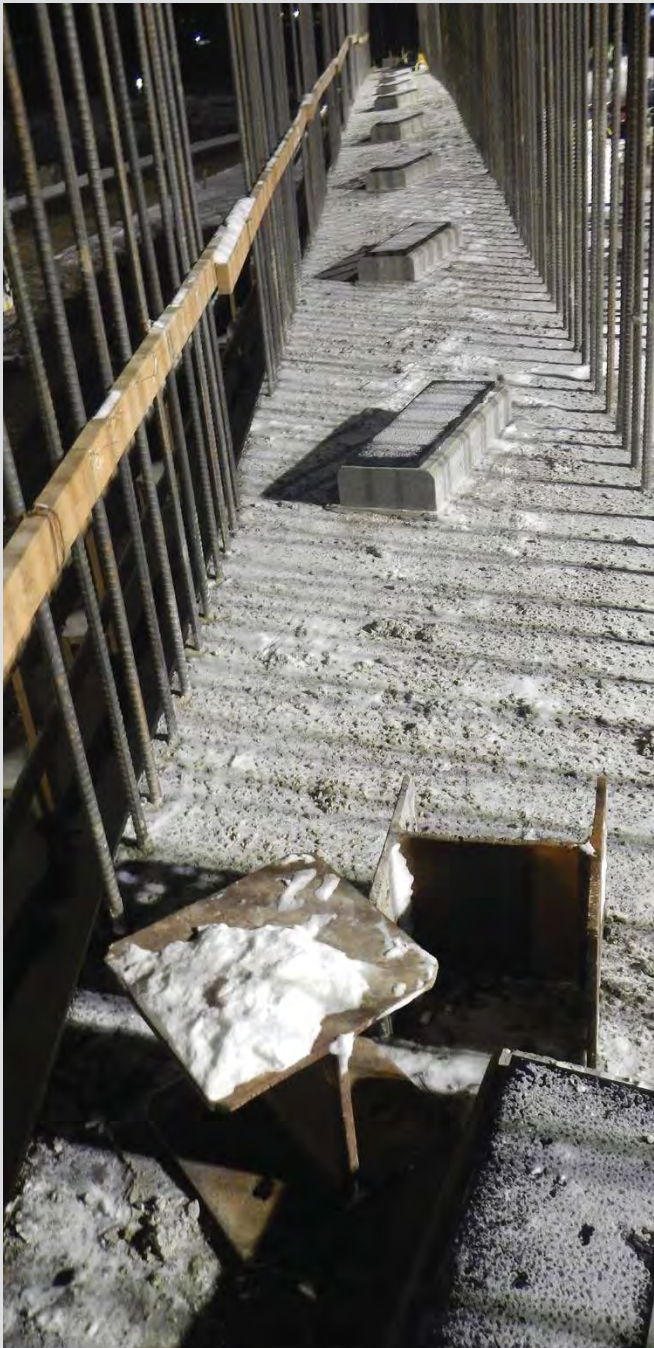
8.17 Concrete plinths on pier cap. Girder to be set on the plinths and cast with the diaphragm.
