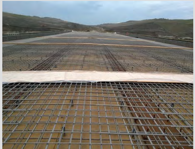
4.46 Deck reinforcing steel installed, tied, and chaired. Bulkheads constructed at planned termination of deck placement sections.
