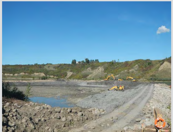
1.8 Berm construction and infill work. Pumping water from work area. Equipment access from top of berm.
