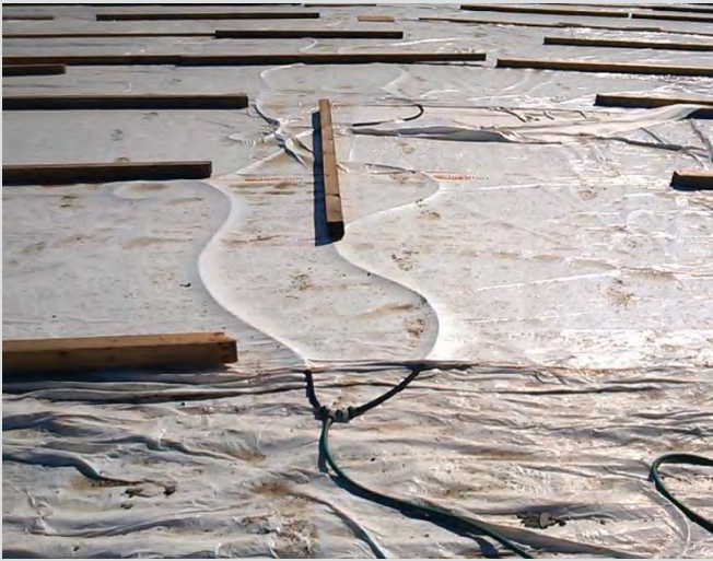
4.71 Soaker hoses are used at the crown to maintain wet filter fabric throughout the curing period.
