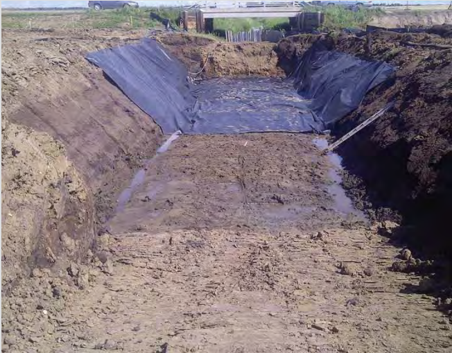
18.15 Excavation for culvert bed. Excavation crowned and sides trenched to control water.
