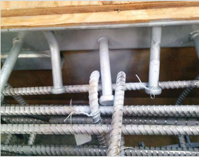
6.22 Damage to galvanized coating during transportation and/or installation. Metallizing repairs completed.
