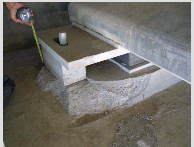
8.18 Damage to grout pad due to improperly set bearing.
