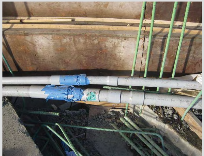
11.8 Poorly aligned connection at expansion joint.
