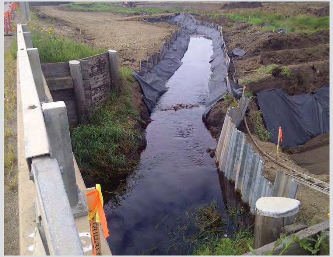
18.14 Temporary diversion for watercourse. Silt fence and filter fabric lining the temporary streambed.
