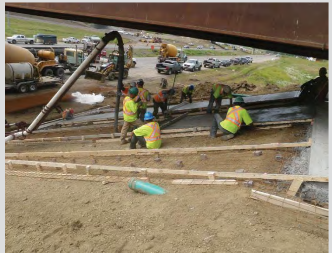
4.112 Pouring vertical courses in alternating sections. Care is required to avoid crushing chairs as pour progresses.
