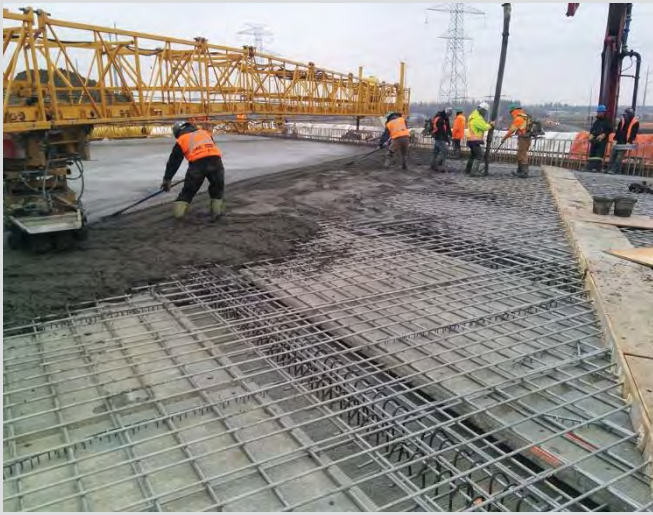
4.55 Bridge deck pour. Screeding closely following placement. Workers avoiding walking on screeded concrete.
