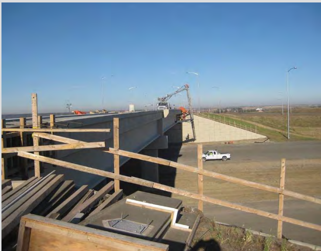
4.90 Concrete surface finishing of exterior faces of barriers. Workers using aerial lift truck to access work.
