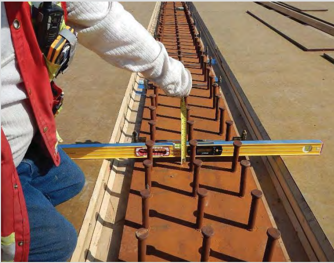
4.39 Prior to installation of reinforcing steel, it is important to check actual haunch values at all girder 10th points to confirm form position accuracy.
