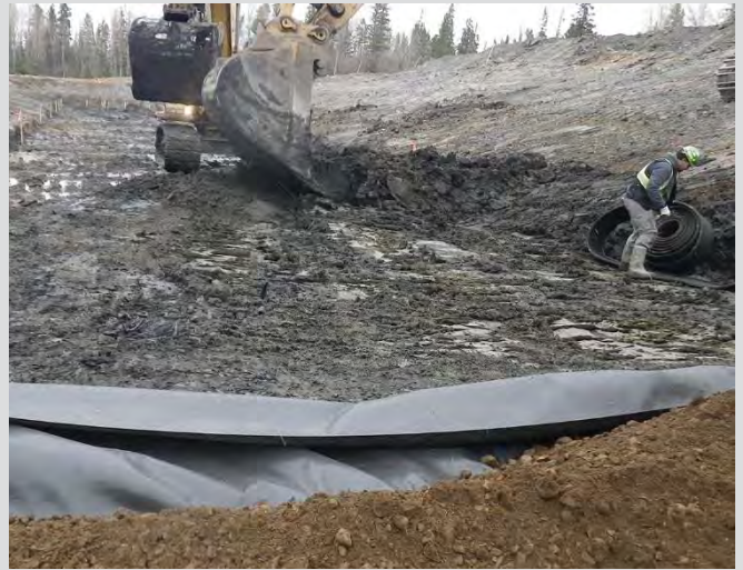
18.26 Soft conditions at culvert bed elevation.
