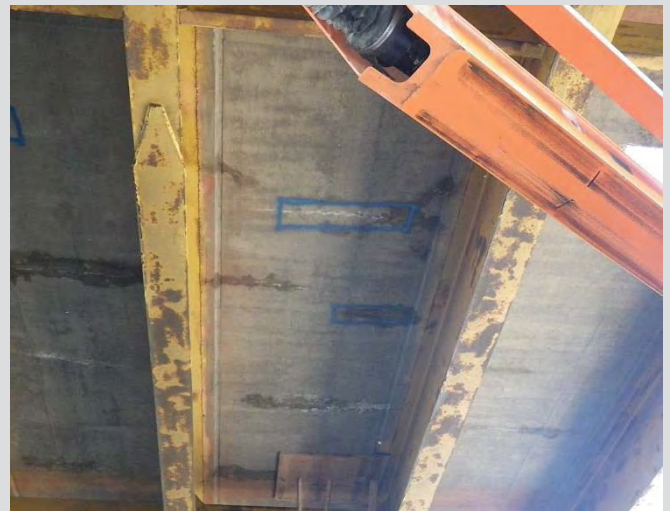
20.8 Full depth repairs are marked onto the deck soffit as well.
