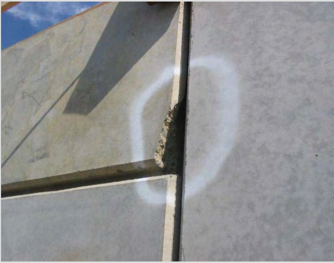
25.19 Panel damaged during erection.
