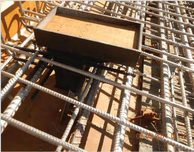
13.1 Polyurethane coated and galvanized deck drain.
