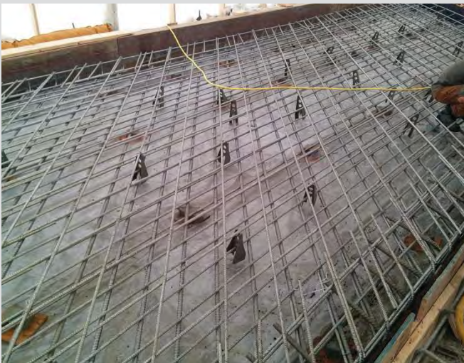
4.73 Approach slab reinforcing steel. Plastic chairs used to separate reinforcing mats. Reinforcing steel placed on skew with deck.
