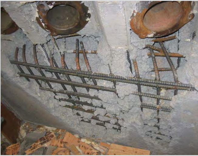
7.40 Severe honeycombing on pier cap due to congestion at post tensioning tendon heads.
