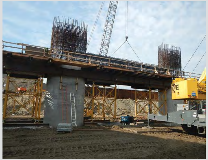
4.13 Pier strut shoring towers and scaffolding. Pre-fabricated reinforcing steel cage installed by crane.
