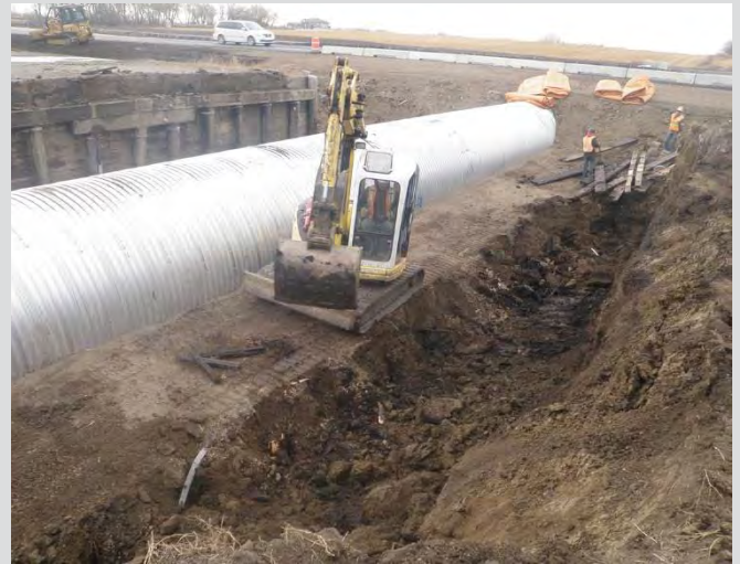
21.4 Demolition of substructure. Piles are removed or cut to specified elevation below streambed.
