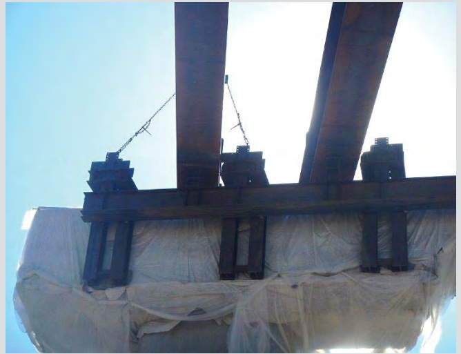
6.6 Temporary bracing, tie downs secured to pier and girder. Diaphragm installation completed prior to release.
