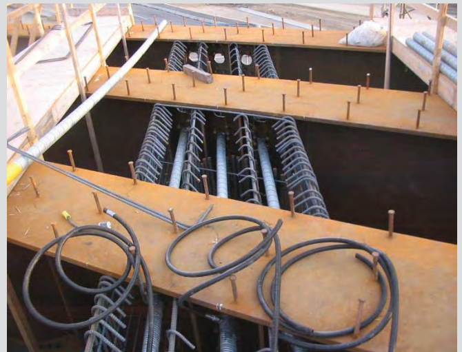
7.20 Post tensioning tendons in pier cap. Survey at every 1.0 m to confirm proper tendon profile.
