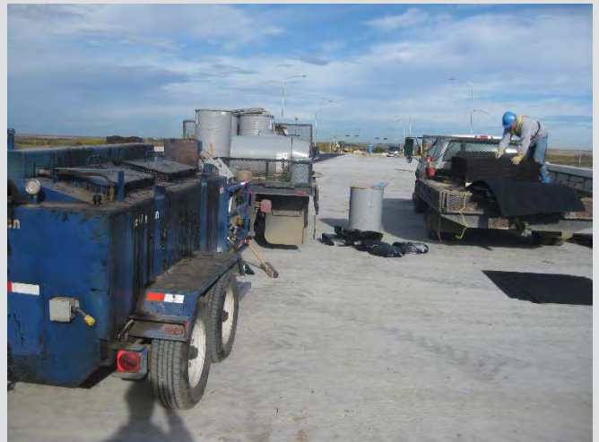
16.4 Waterproofing equipment and materials. Heating and mixing kettle on site. Workers unloading protection board.
