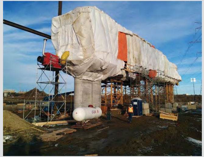
4.24 Scaffolding and shoring towers for straddlebent pier beam. Heating and hoarding for cold weather concreting in place.
