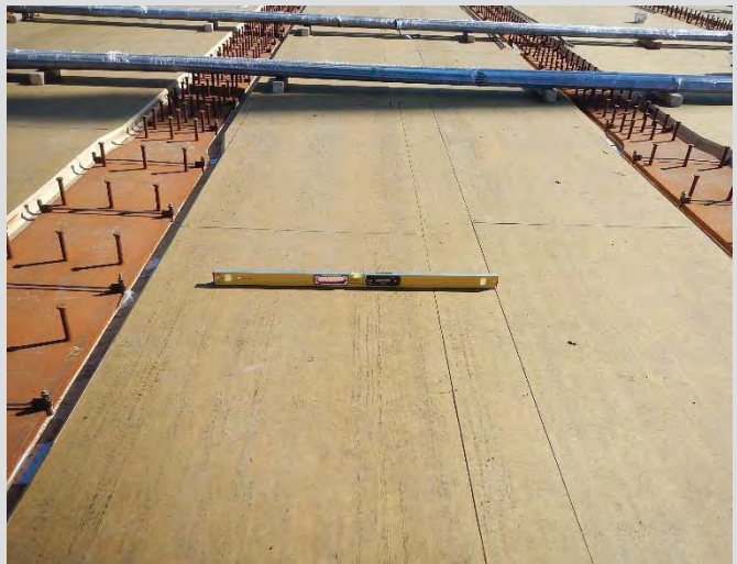
4.38 Prior to installation of reinforcing steel, it is important to check form cross-fall to confirm form position accuracy.
