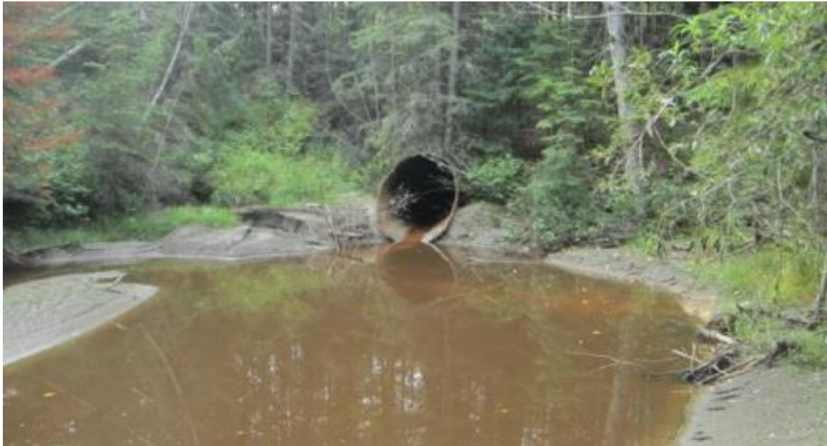
Photo No. 5b (Taken by AT in 2018) – Erosion and debris around culvert outlet; culvert outlet heaved by about 300 mm above the creek bed
