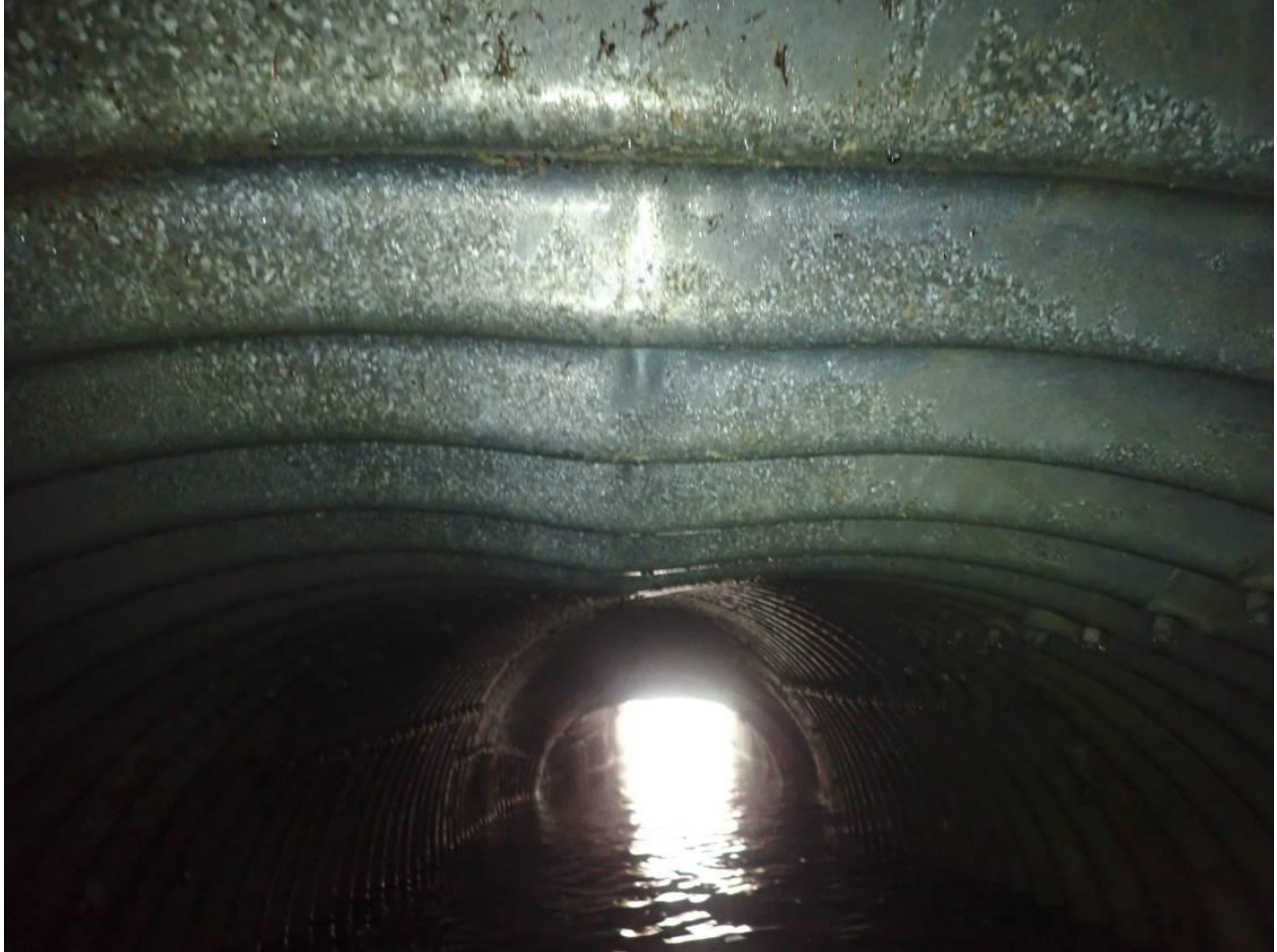
Photo No. 9 – Looking inside CSP Culvert outlet; note reverse curvature in the roof (Photograph was taken by AT during bridge culvert inspection completed on June 3, 2020). This is approximately 27 to 30 m from the culvert outlet location.
