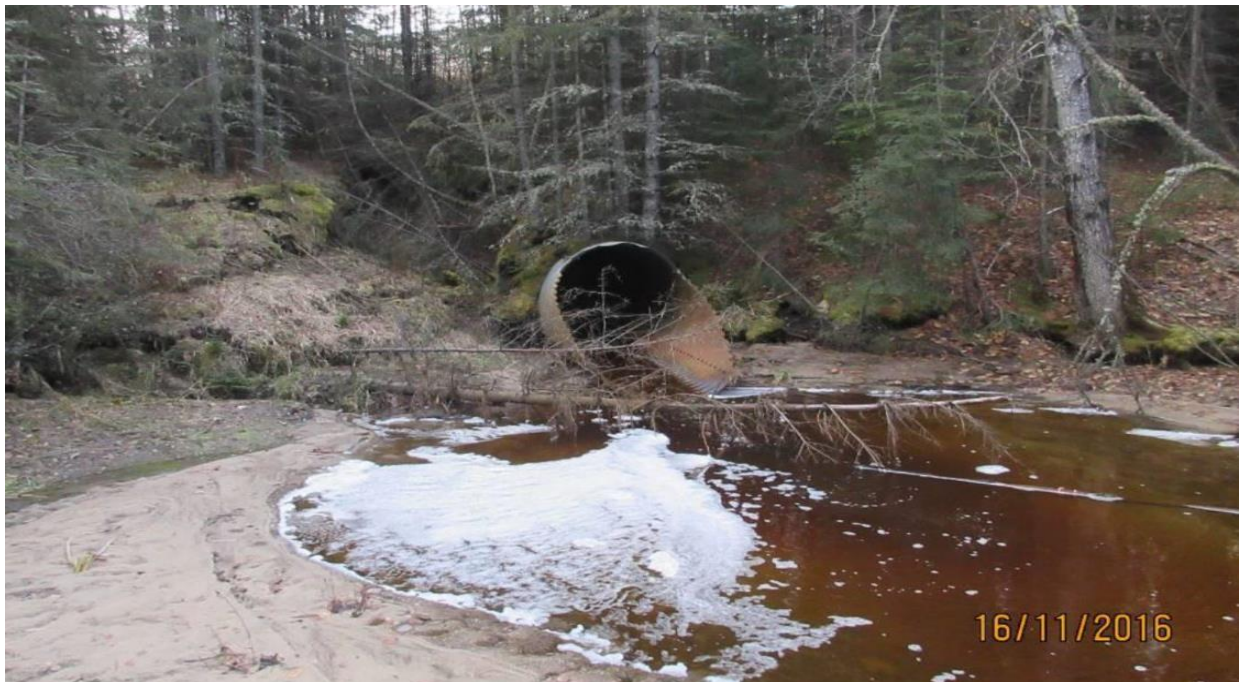
Photo No. 5a (Taken by AT in 2016) – Erosion and debris at the culvert outlet; note the absence of riprap at the culvert outlet location
