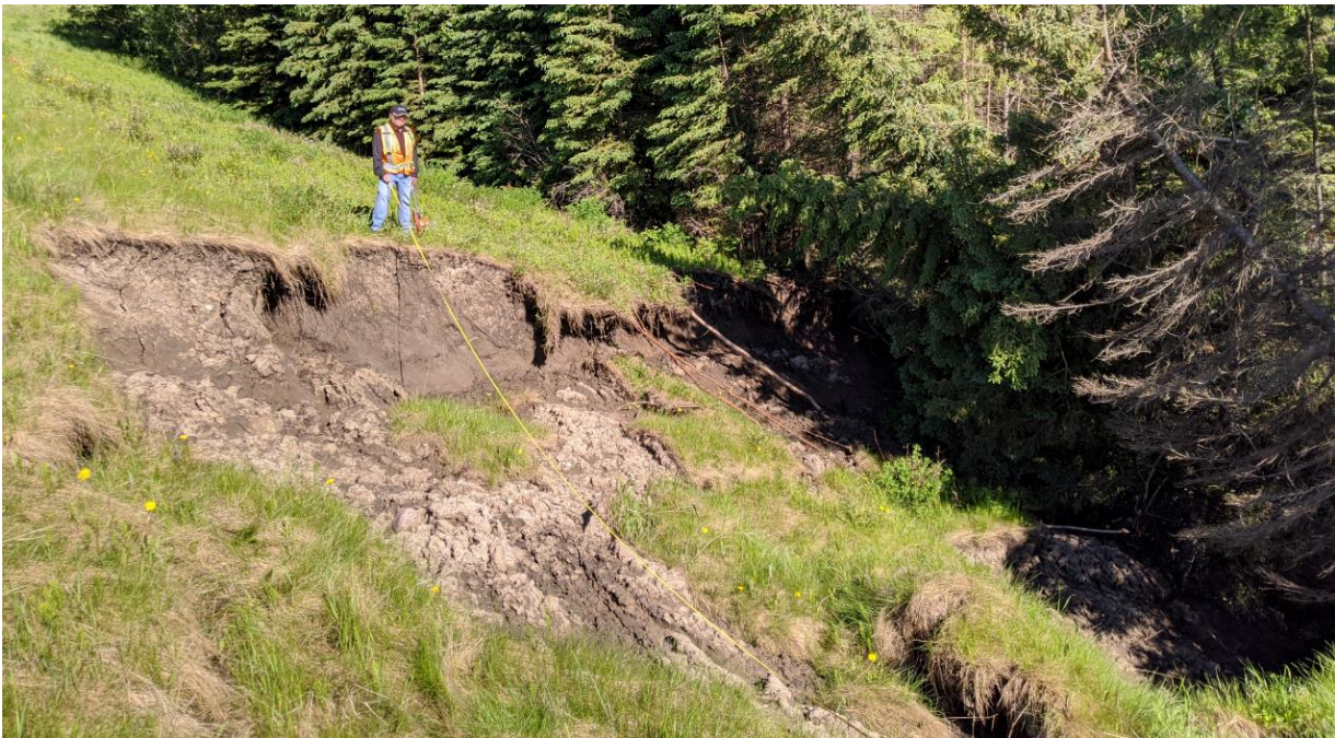
Photo No. 2 – Looking west at the north embankment landslide's head scarp and western flank; note the presence of fallen and tilting trees, and seepage along the western flank; landslide mass was noted to be wet at the time of the inspection.
