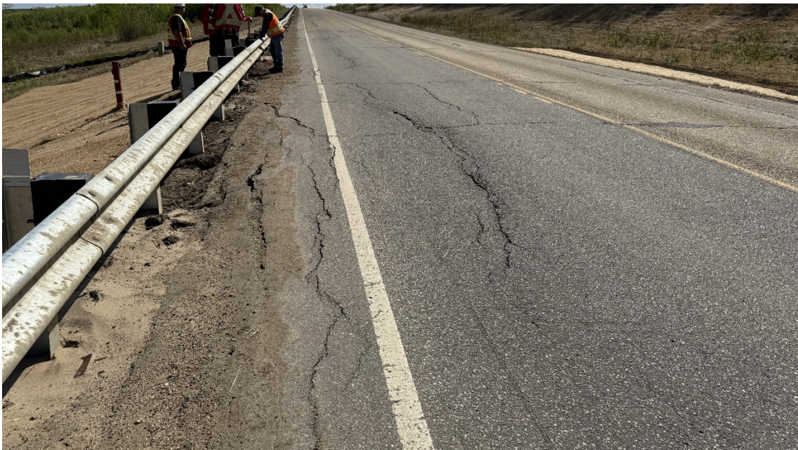
Photo 5. Looking east at the most severe area of pavement distress within the slide. The dips and cracks have not shown substantial change since construction of the pile wall in 2024.
