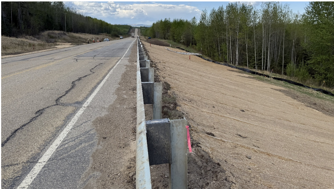
Photo 2. Looking west at the flank of the landslide area and the west edge of the 2021 ACP patch.
