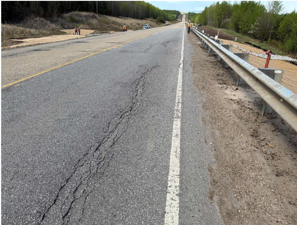
Photo 4. Looking west at longitudinal cracks on the highway.
