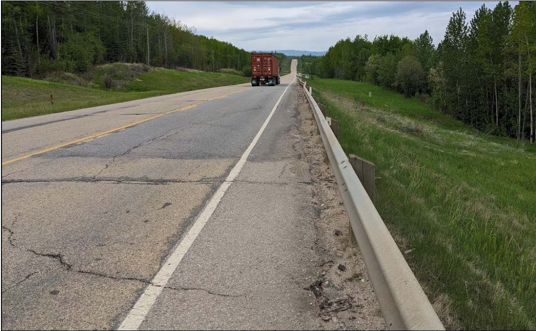
Photo 3A (2024 Inspection). Looking west at the edge of the 2021 ACP patch. Reflective cracks are visible through the ACP patch.
