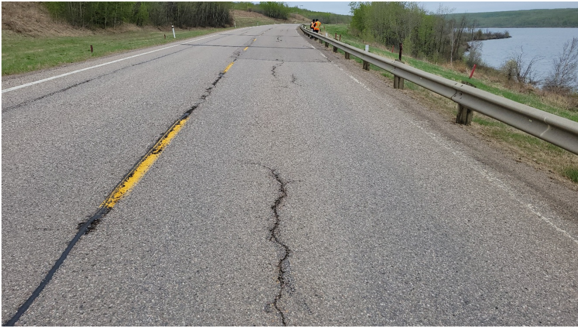
Photo 3. Looking south at reflective cracks through north 2017 ACP patch.
