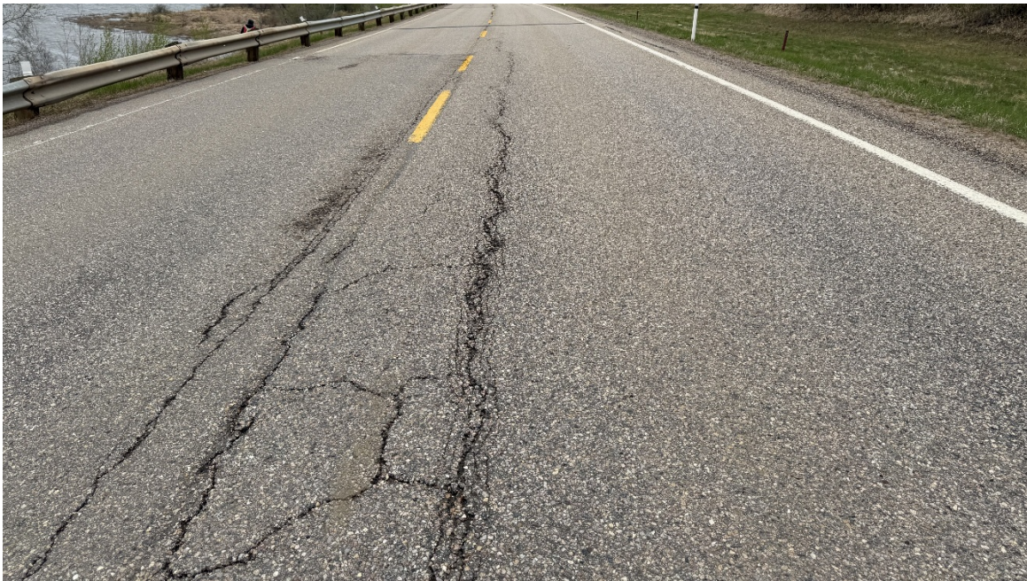
Photo 2. Looking north at reflective cracks in the highway surface at the NC102 pile wall location. Cracks are 10-80 mm wide, with a 10-20 mm drop.
