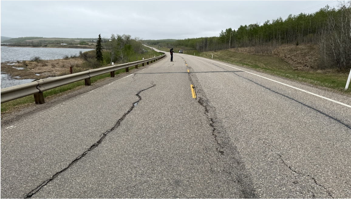
Photo 5. Looking north at reflective cracks near north end of NC102 pile wall. Reflective crack in middle of southbound lane is up to 100 mm wide with 30 mm drop. Centerline crack is up to 150 mm wide with a 30 mm drop.
