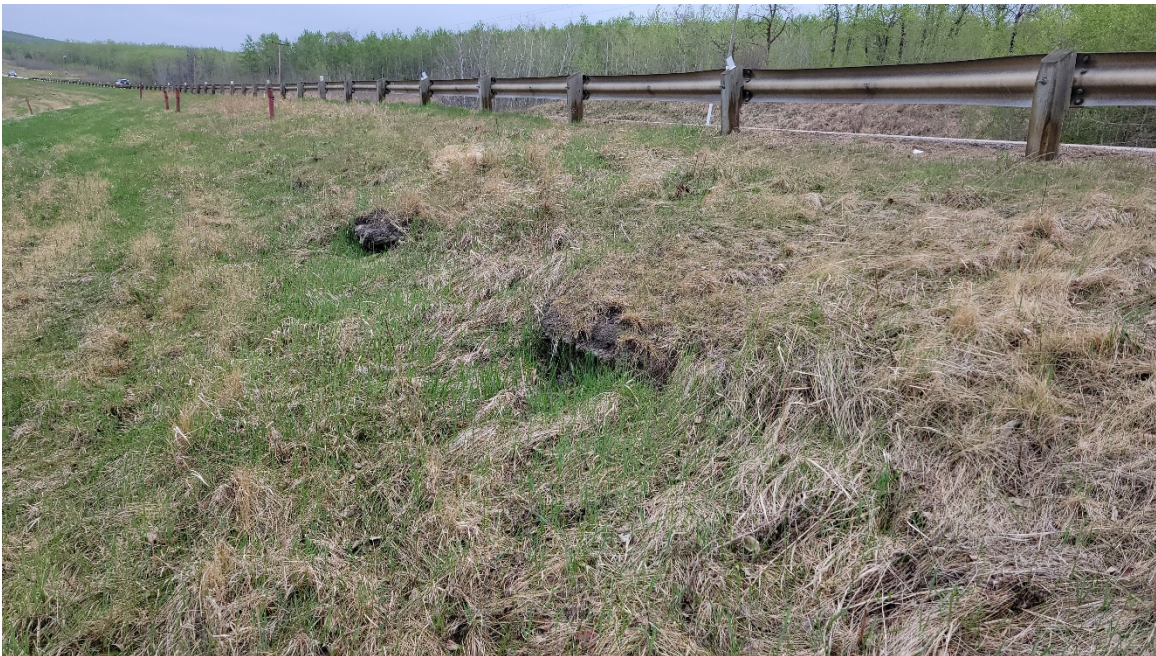
Photo 8. Looking at the tops of exposed concrete piles. The cracks in front of the piles are 300 mm deep.
