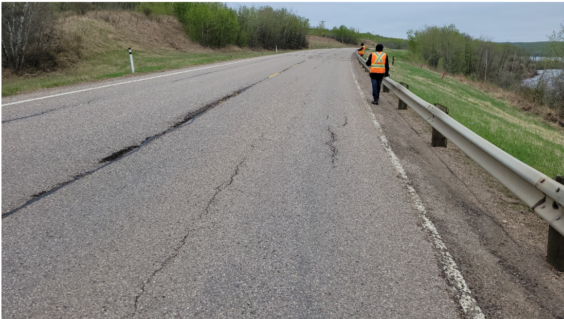
Photo 6. Looking south at 5 to 20 mm wide reflective cracks with no drop on the southbound lane, up to 150 mm wide and 30 mm deep along centerline.
