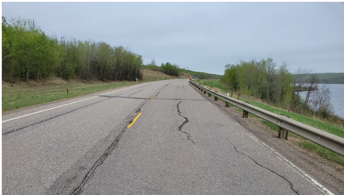
Photo 4. Looking south at reflective cracks in north ACP patch. Reflective crack in middle of southbound lane is 10-70 mm wide with a 30 mm drop.
