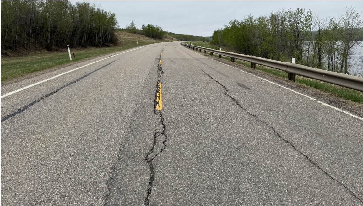
Photo 7. Looking south at 60 to 100 mm wide reflective cracks with up to 5 mm drop.
