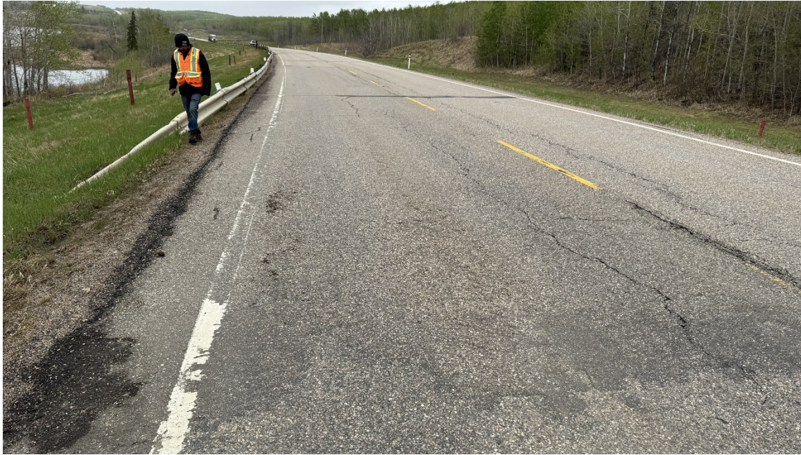
Photo 1. Looking north at the 2017 ACP patch placed on the highway surface at the NC102 pile wall location; no visible dip on highway surface.
