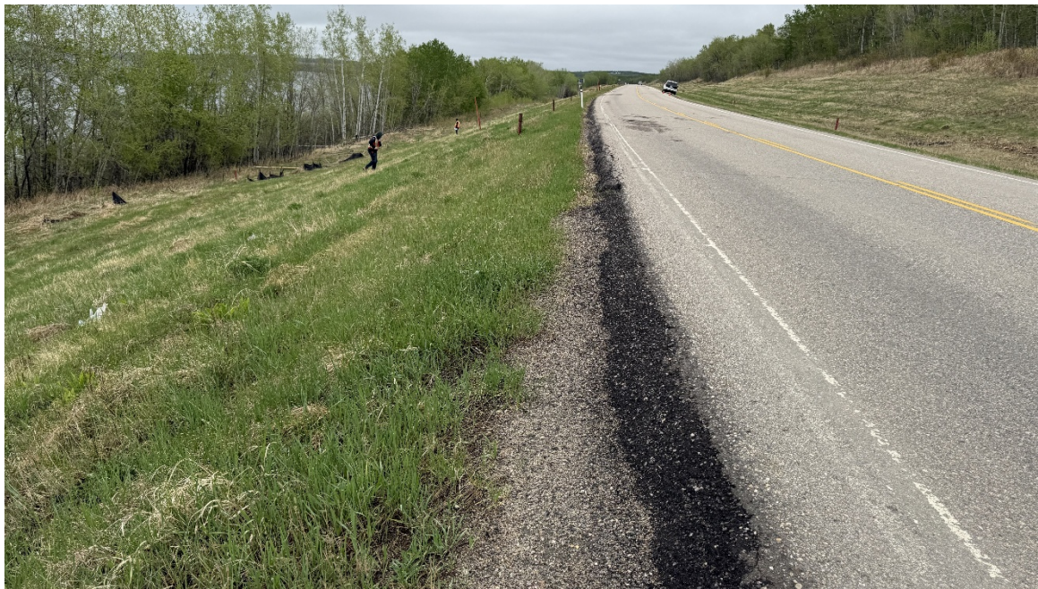
Photo 4. Looking north at sharp drop at shoulder of pavement on the southbound lane.
