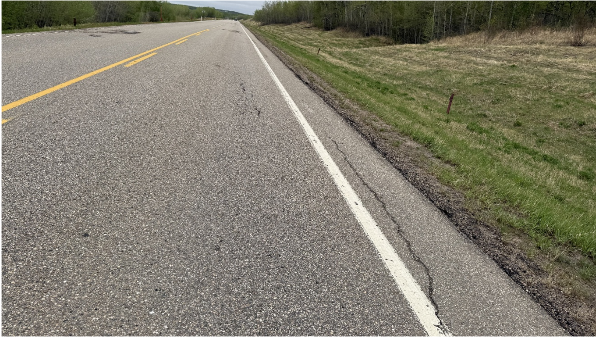
Photo 7. Looking north at reflective cracks, 10 to 60 mm wide with no drop, in the northbound lane.
