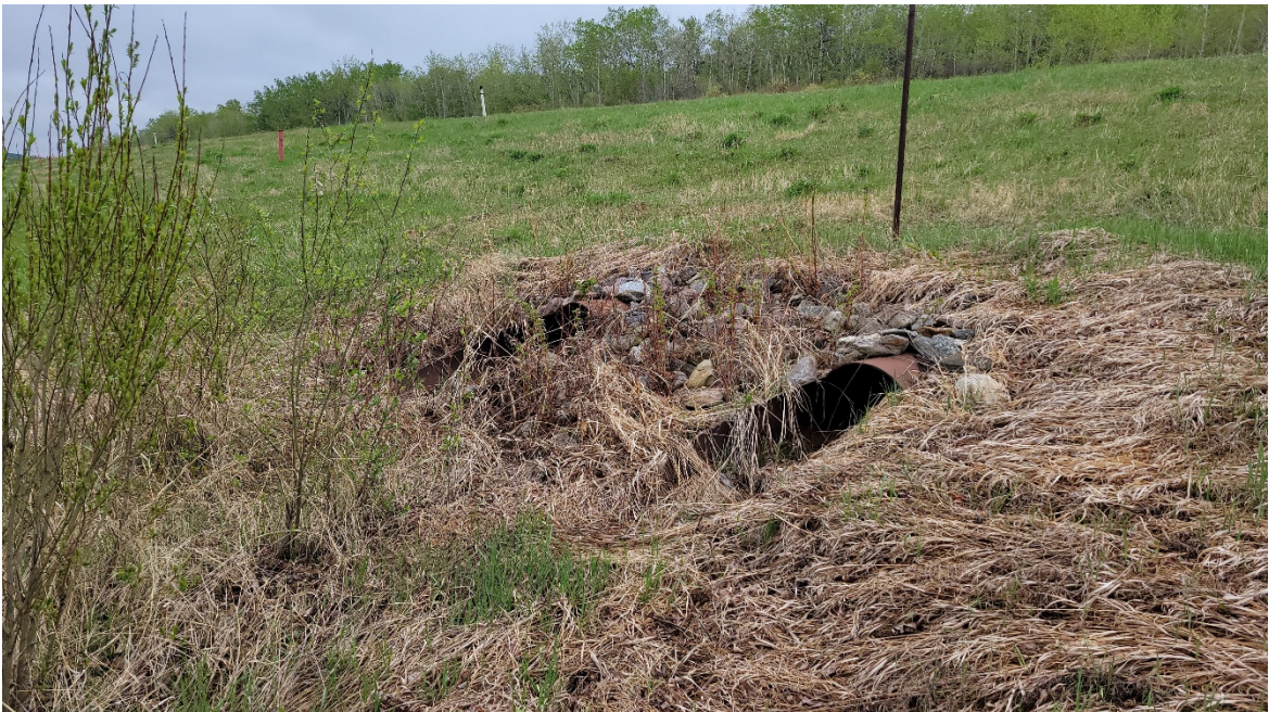
Photo 2. Looking northeast at the twin culvert outlets. 10-20 mm of sediment has accumulated at the outlets of the culverts since the 2023 inspection.
