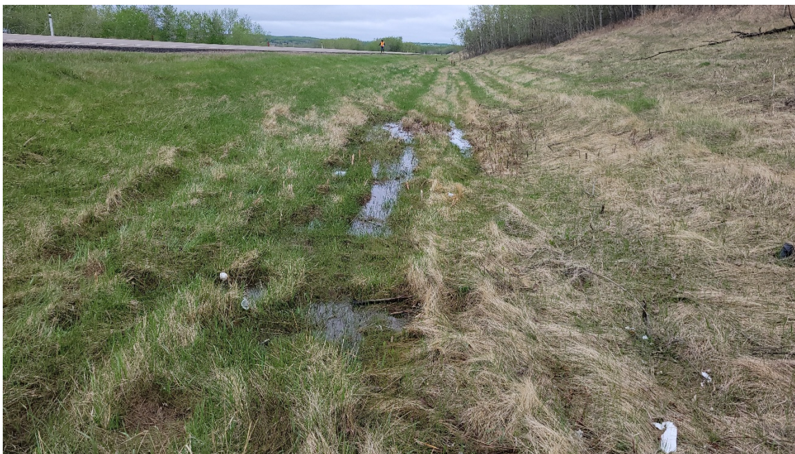
Photo 9. Looking north at ponding water in the east highway ditch. |
