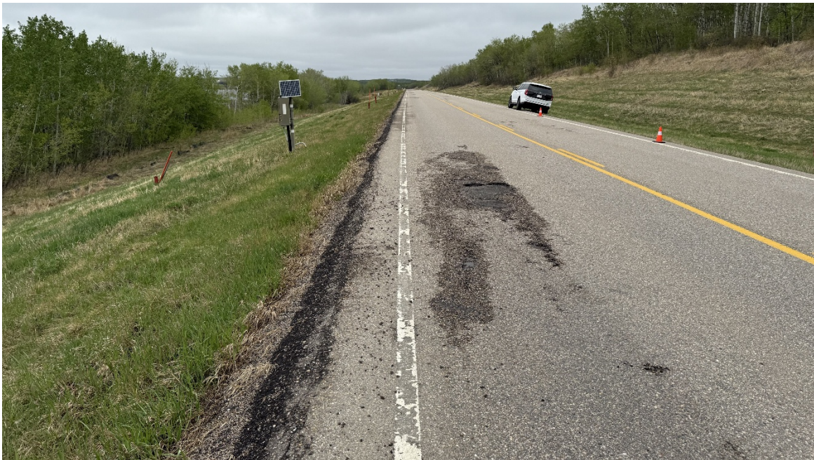
Photo 6. Looking at datalogger DT1 installed at the pile P146 location in the NC104 pile wall extension. New pothole with segregation developed in 2025.
