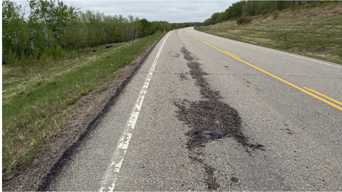
Photo 1. Looking north at highway surface from the south end of site. Segregation and raveling of pavement have worsened since the 2023 inspection. Some cold mix asphalt was placed in 2025.
