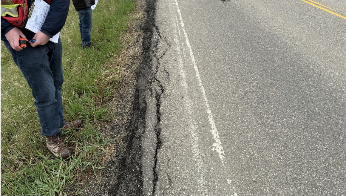
Photo 5. Pavement stress cracks noted on southbound lane shoulder near south end of NC104 pile wall extension. Cracks were 20-50 mm wide with a 10-20 mm drop.
