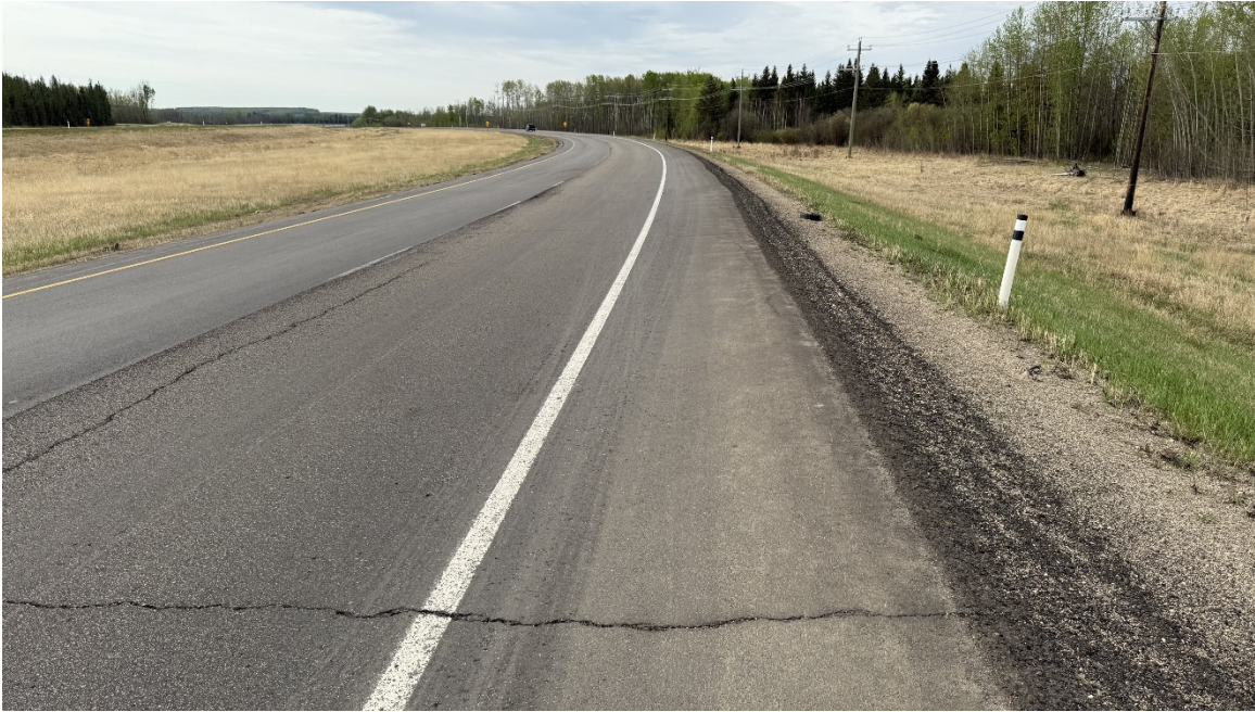
Photo 11. Looking south at middle section of the NC08-2 landslide. Reflective cracks 5-10 mm wide are visible in the recent ACP overlay.
