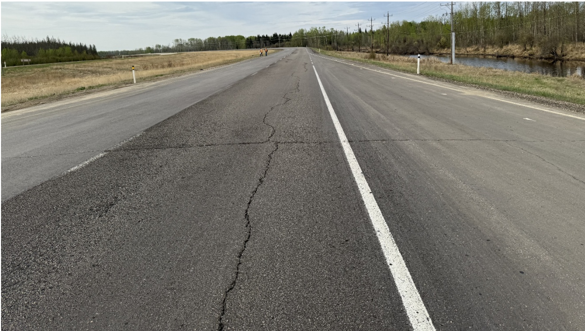
Photo 6. Looking south at highway within the limits of the area repaired in 1997 (previously known as NC08-1). Highway was overlaid in September 2024, but reflective cracks (10-100 mm wide, no drop) are visible through the new ACP.
