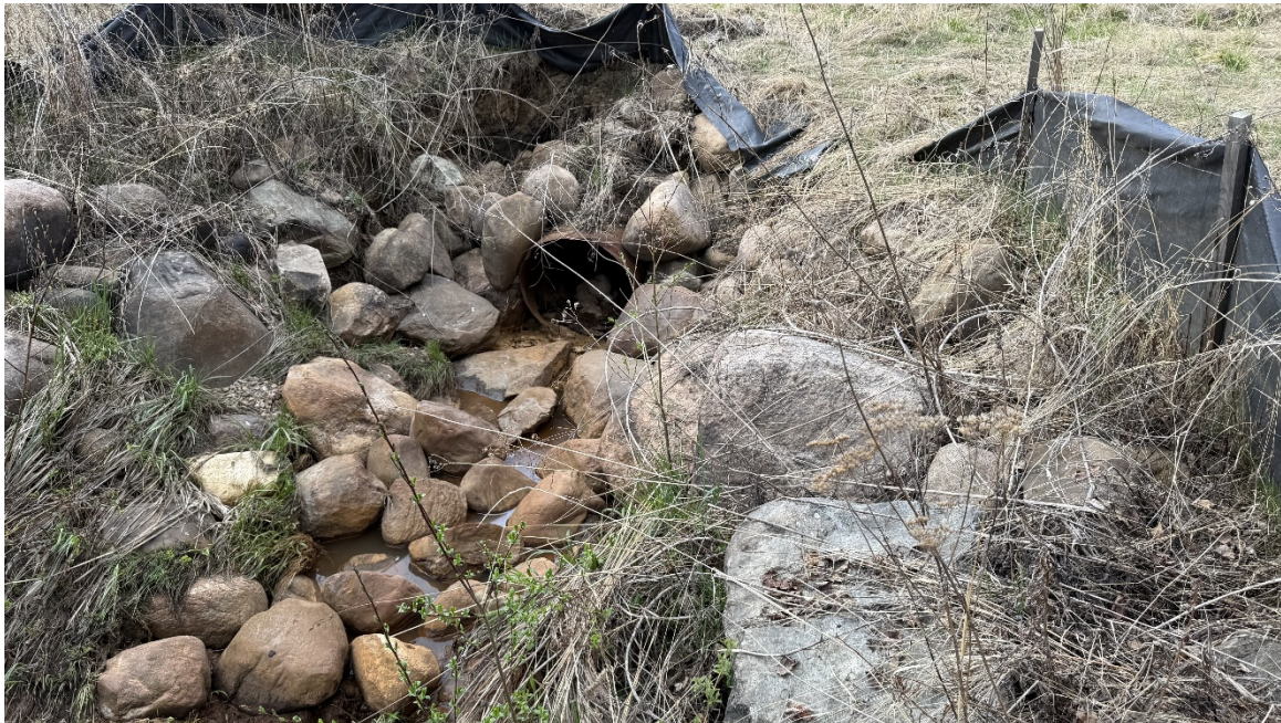
Photo 4. Steady water flow from Culvert C1 outlet (though noticeably less than during 2024 inspection). Bottom of culvert barrel is severely corroded at outlet.
