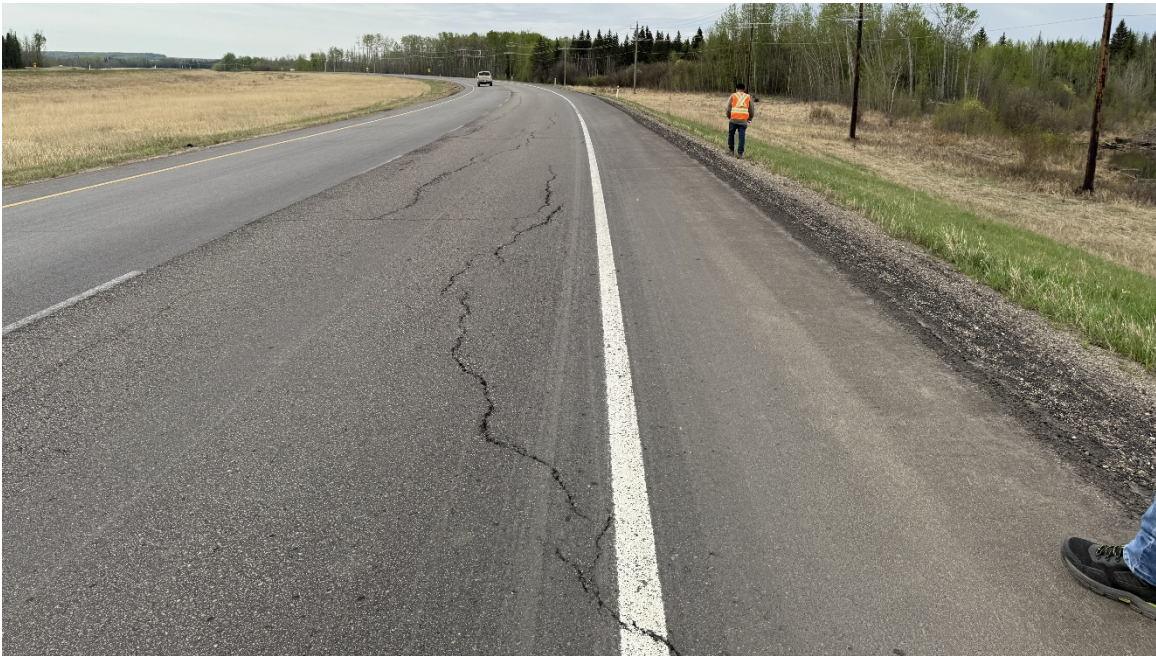
Photo 10. Looking at the northern flank of the new landslide (NC08-2). Previous ACP patch is no longer visible (new ACP overlay completed September 2024). Reflective cracks 10-20 mm wide are visible in the ACP overlay.
