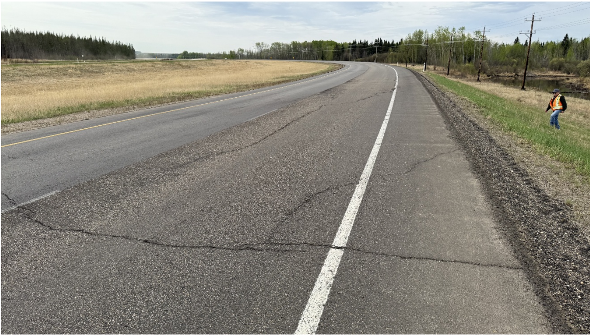
Photo 9. Looking south at the southern flank cracks of the NC08-1 repaired landslide.
