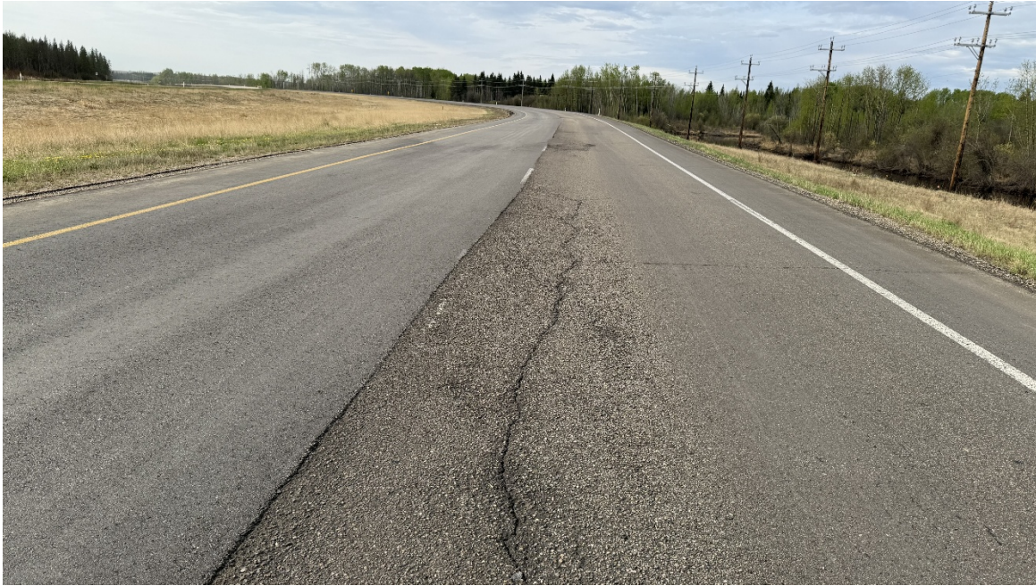
Photo 7. Looking south at highway within the limits of the NC08-1 repaired area. Reflective cracks are visible through the ACP overlay area.
