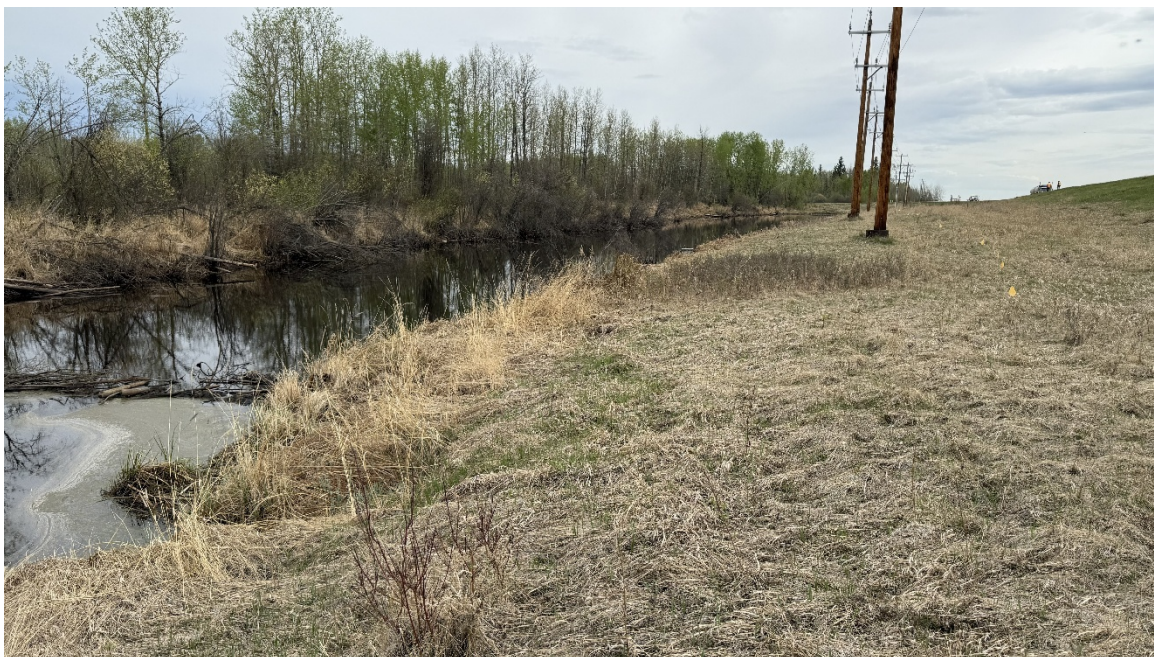
Photo 13. Looking north at landslide toe bulge. Beaver Dam 3 is visible at the left of the photo.
