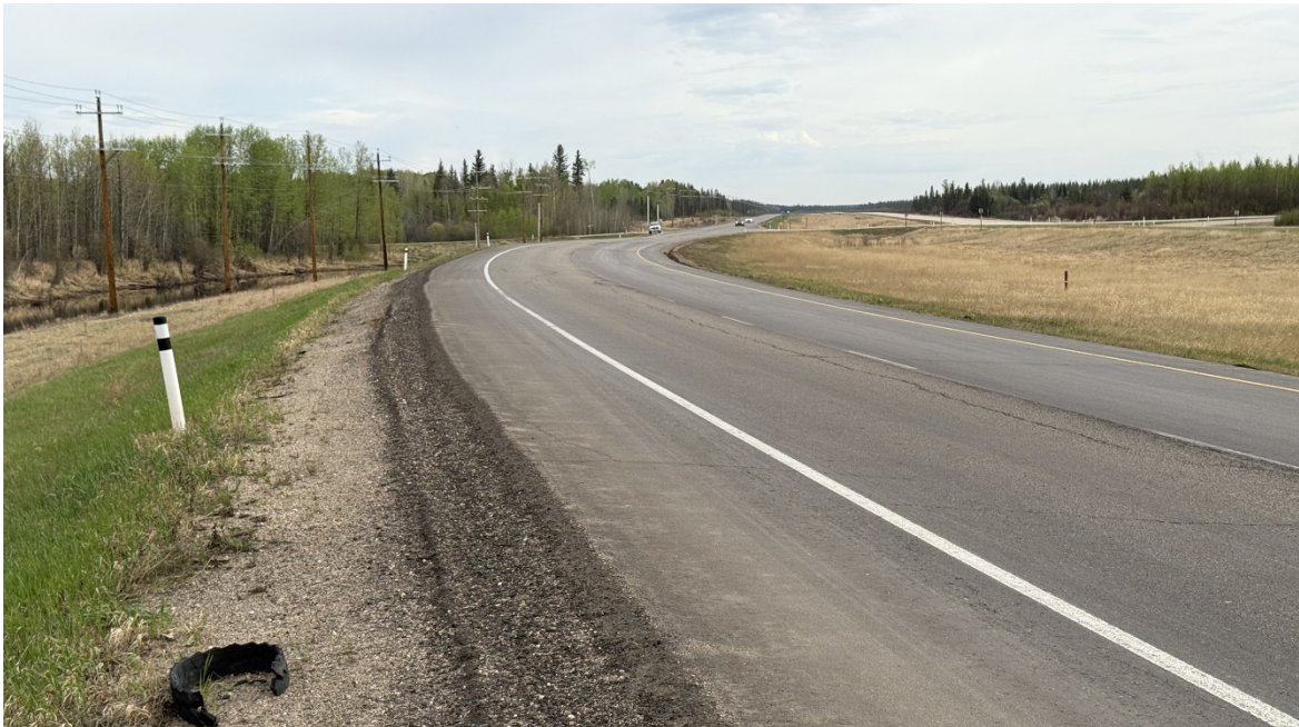
Photo 12. Looking north at southern flank of NC08-2 landslide. Hairline cracks are visible through the recent ACP overlay.
