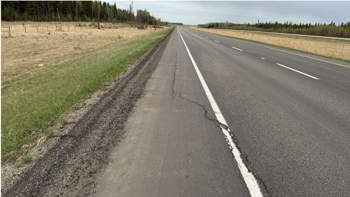
Photo 6A. Looking north at the diagonal crack appearing through the 2024 ACP overlay north of the landslide north flank. Crack is 10-20 mm wide with no drop.
