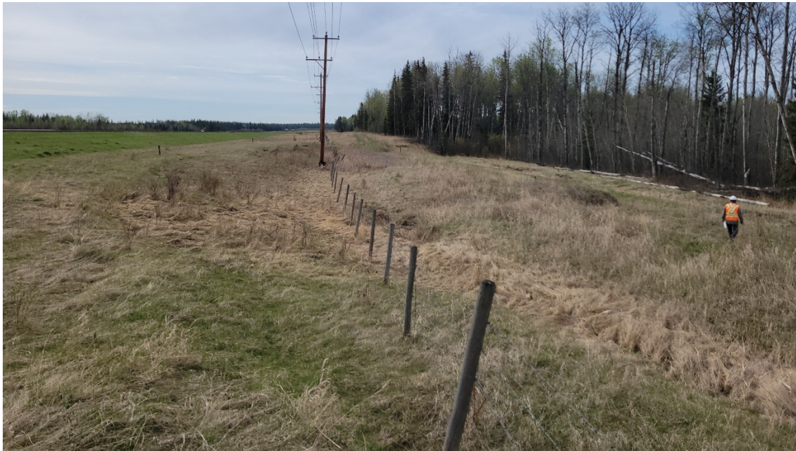
Photo 1. Looking south at head scarp crack of upper landslide block
