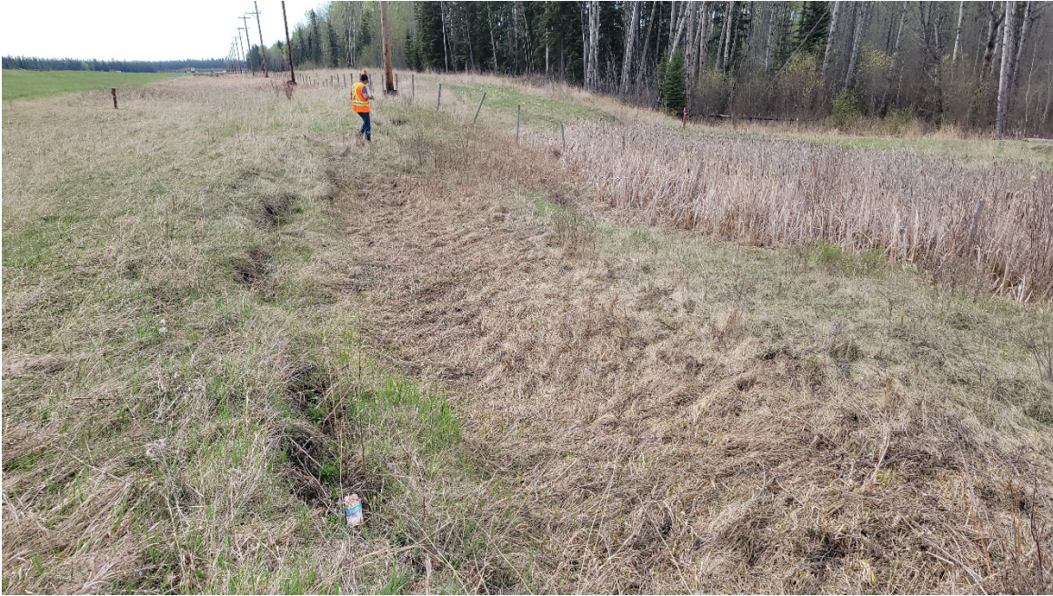
Photo 3. Looking south towards the southern flank of the landslide (700 mm wide cracks, up to 1.1 m drop). Water is ponding along the ditch between the trail and the fence (note the cat tails in this area).
