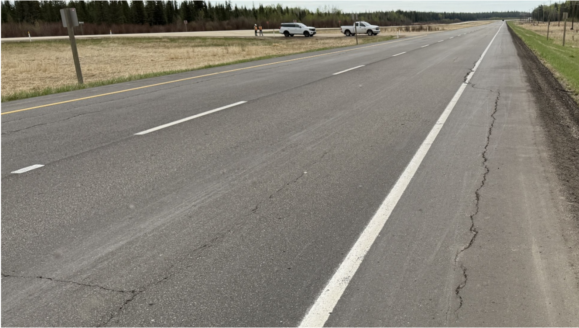
Photo 6B. Looking south at diagonal crack appearing through the 2024 ACP overlay north of the landslide north flank. Crack is 10-20 mm wide with no drop).
