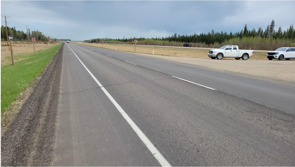
Photo 5. Looking north at highway southbound lanes. Landslide is currently not impacting the highway surface; head scarp crack is about 6.5 m from the edge of pavement (same as 2023 inspection).
