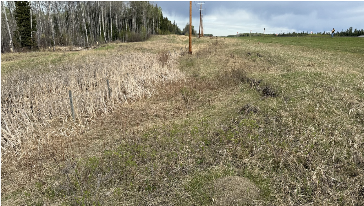
Photo 4. Looking north at the southern flank of upper and lower landslide blocks; note standing water within the flank and lateral shifting of fence. Landslide is well vegetated.
