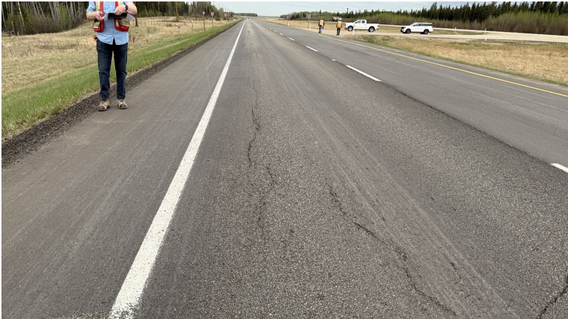
Photo 7. Looking north at cracking in southbound lane near landslide southern flank. Cracks are 5-10 mm wide with no drop.
