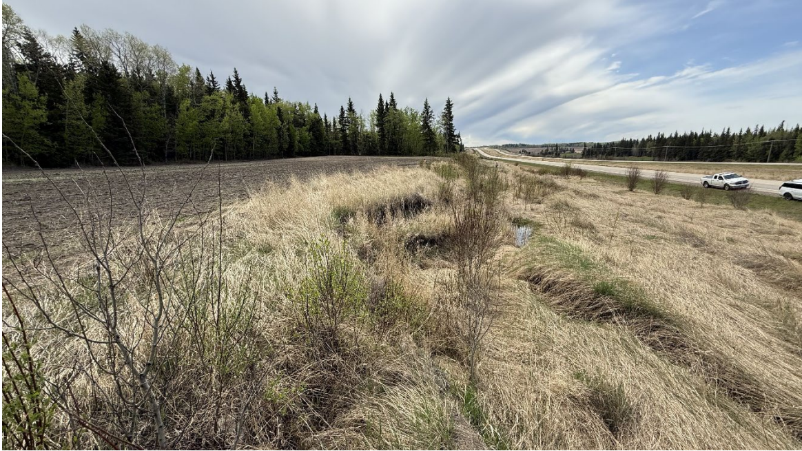
Photo 9. NC091-2: Looking south at a scarp crack developed within the crest of the backslope.
