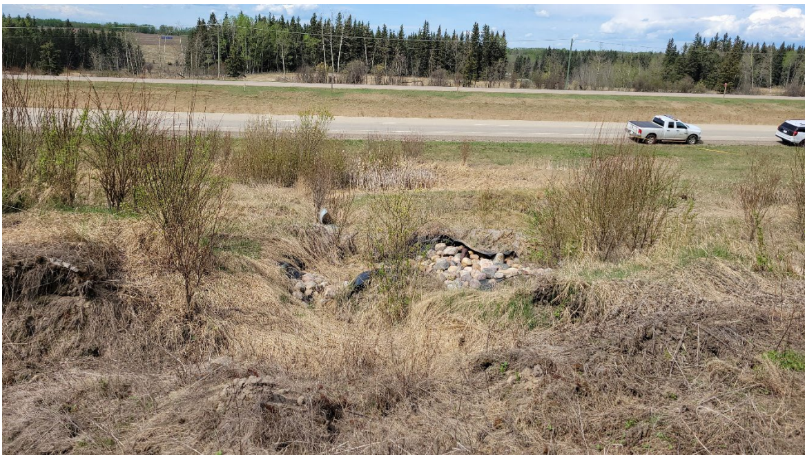
Photo 12. NC091-2: Looking west at the failed riprap apron and half-pipe culvert.
