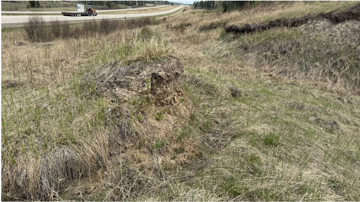
Photo 5. NC091-1: Looking northwest at graben feature developed in the middle of the landslide mass.
