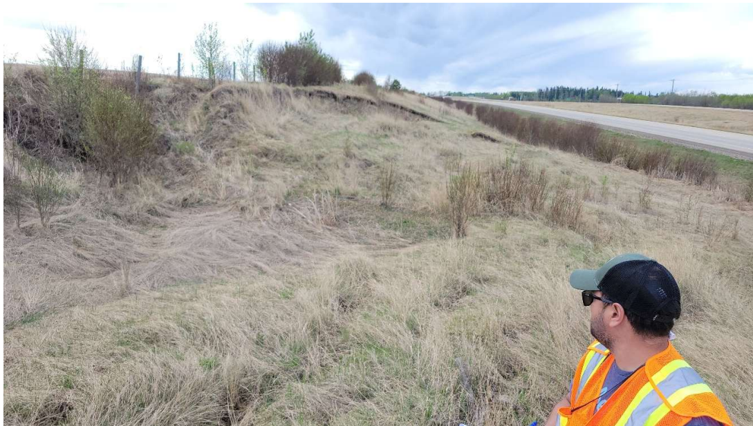
Photo 4. NC091-1: Looking south at landslide mass. The retrogression of the backscarp crack into the farmer's field is visible on the left of the photo. Eight barbed if it got wire posts were hanging in 2025.
