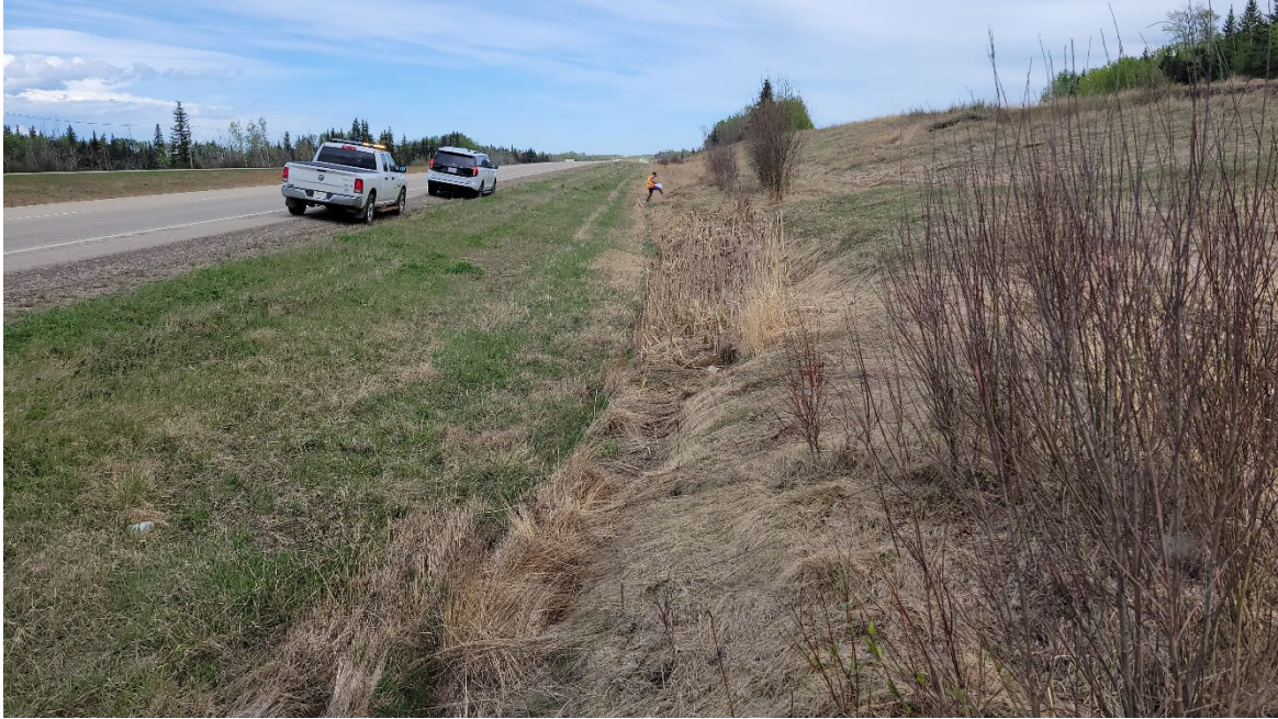
Photo 7. NC091-2: Looking north near the southern flank of the landslide; note the presence of a distinct toe roll in the ditch.
