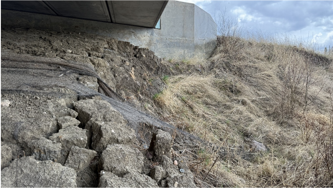
Photo 7. Looking southwest at slump no. 2 flank. There is a 0.65 m drop from the original fill height at the abutment (shown as the soil staining in the photo).
