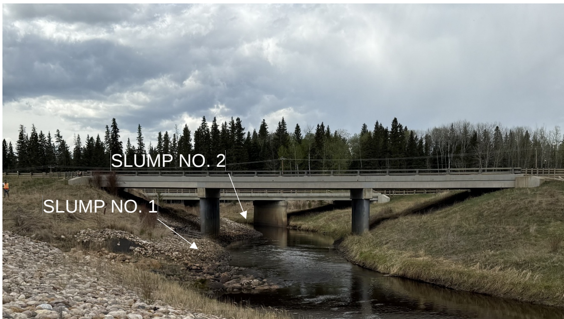
Photo 4. Slumping within the riverbank to the east of the Hwy (slump no. 1) and to the west of the Hwy (slump no. 2). Note distinct toe rolls in the river channel.
