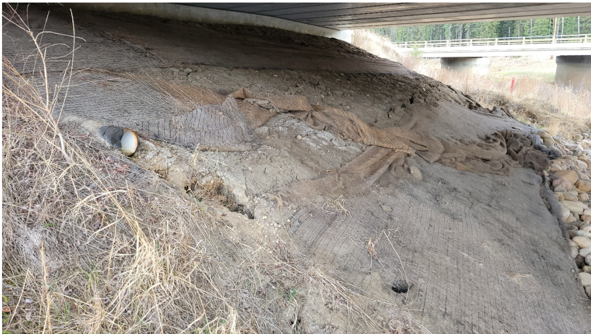
Photo 6. Looking at crack on headslope extending to the subdrain on the east side of the bridge. Crack is 5 mm wide at the subdrain and 700 mm at 10 m west of the subdrain.
