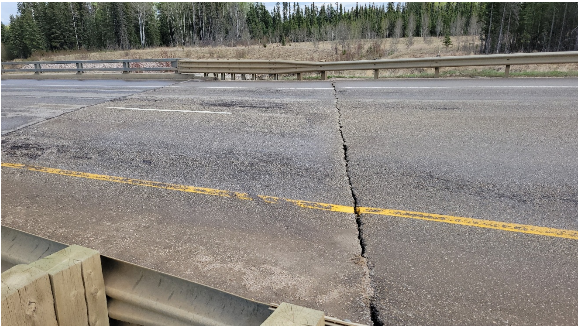
Photo 8. Dip (25 mm to 30 mm) at the bridge south approach slab. Crack is 40-70 mm wide.
