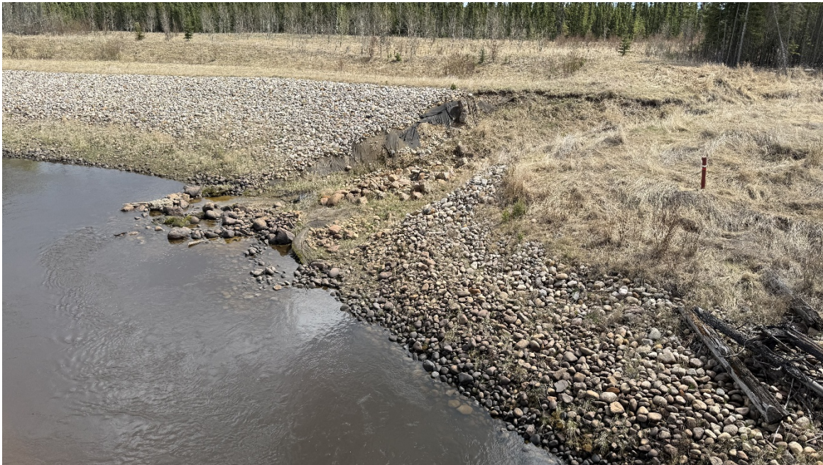
Photo 3. Looking southeast at mouth of the severe erosion channel.
