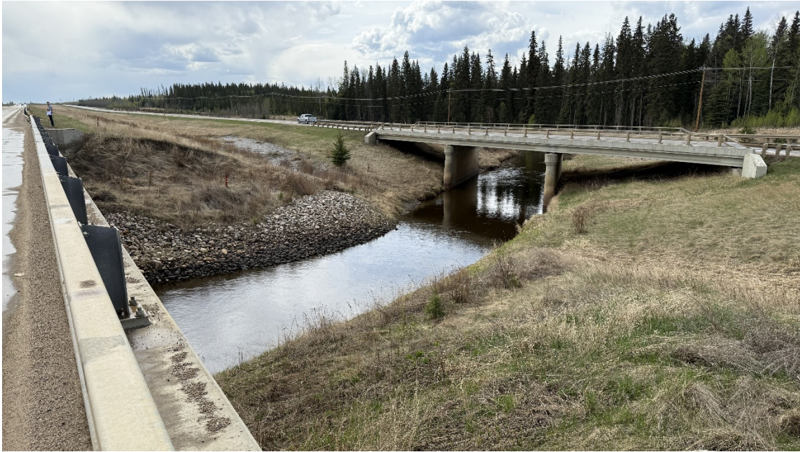
Photo 5. Looking southwest at slump no. 2 area. Slump area is well vegetated.
