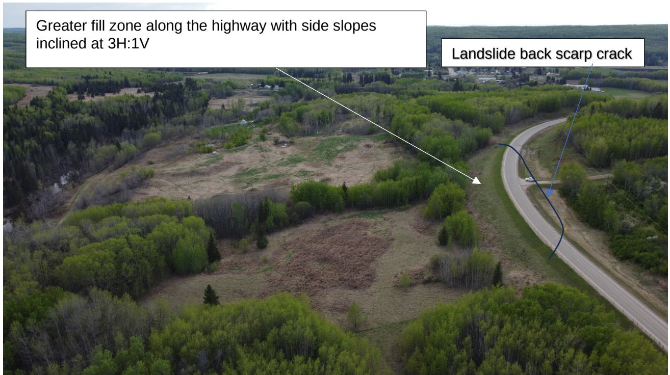
Photo 11 (drone shot). Looking west from beyond the eastern limits of the landslide. Little Pine Creek is visible on the left side of the photo. Hummocky terrain is visible downslope of the highway. Note fill section along the highway notably higher within landslide area.
