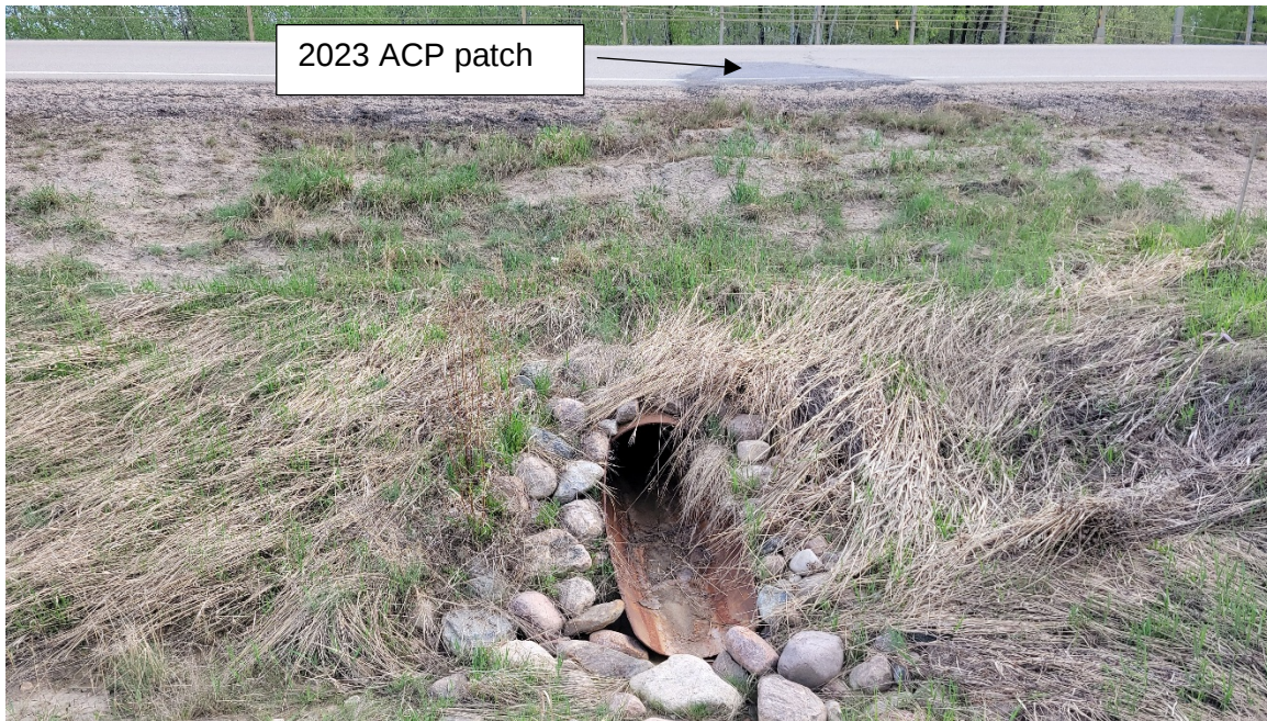
Photo 7. Looking south at the inlet of culvert C3 – No flow noted in 2025. The 1.9 m wide ACP patch on the highway surface dropped by 30 mm.
