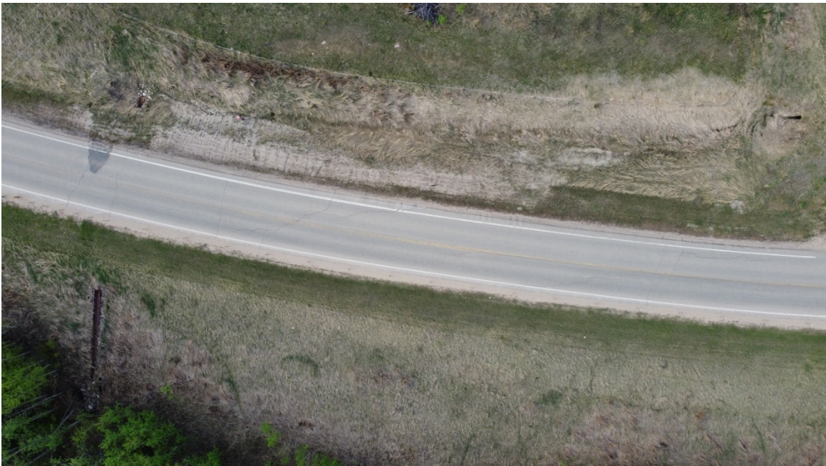
Photo 12 (drone shot). Highway west of access road. Erosion on the ditch slope is visible. Inlet of culvert C3, sinkhole area and ACP patch, and C3 culvert outlet and half pipe extension is visible on the left of the photo.
