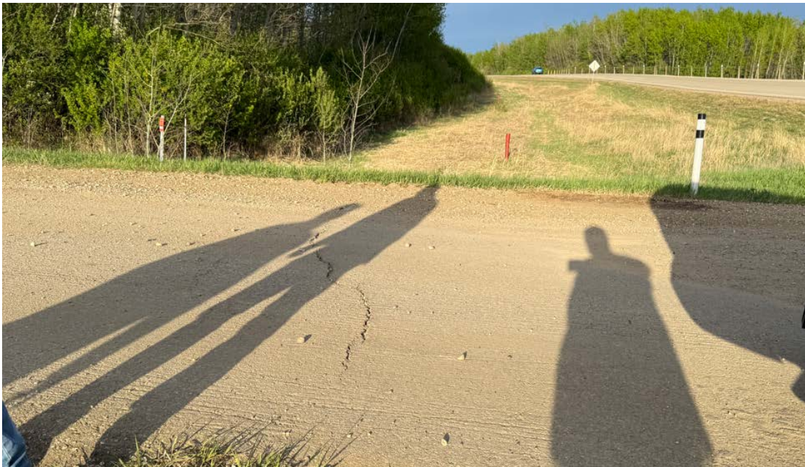
Photo 14. Possible backscarp crack 30 mm wide, no drop
