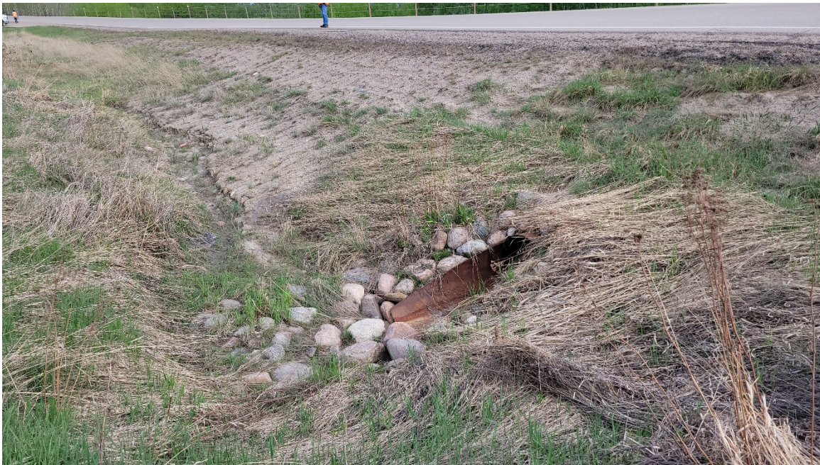
Photo 8. C3 inlet; side slope still is bare of vegetation; erosion developing upstream of the inlet within the ditch.
