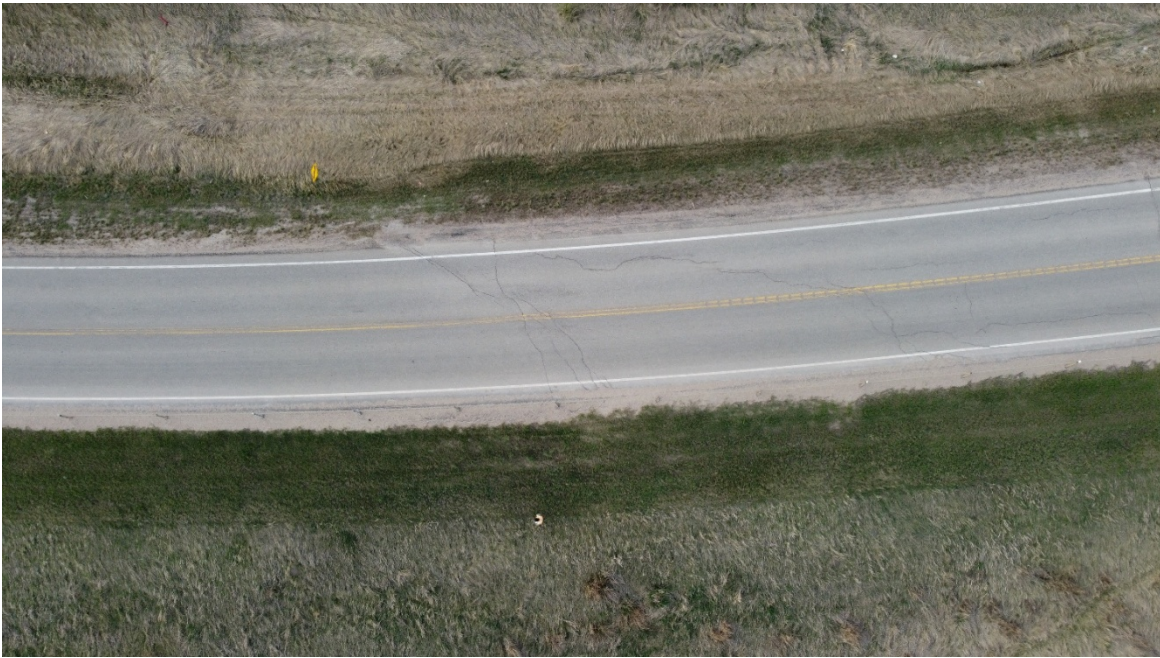
Photo 13 (drone shot). Highway east of access road showing the eastern flank of the highway and cracking pattern in the ACP.
