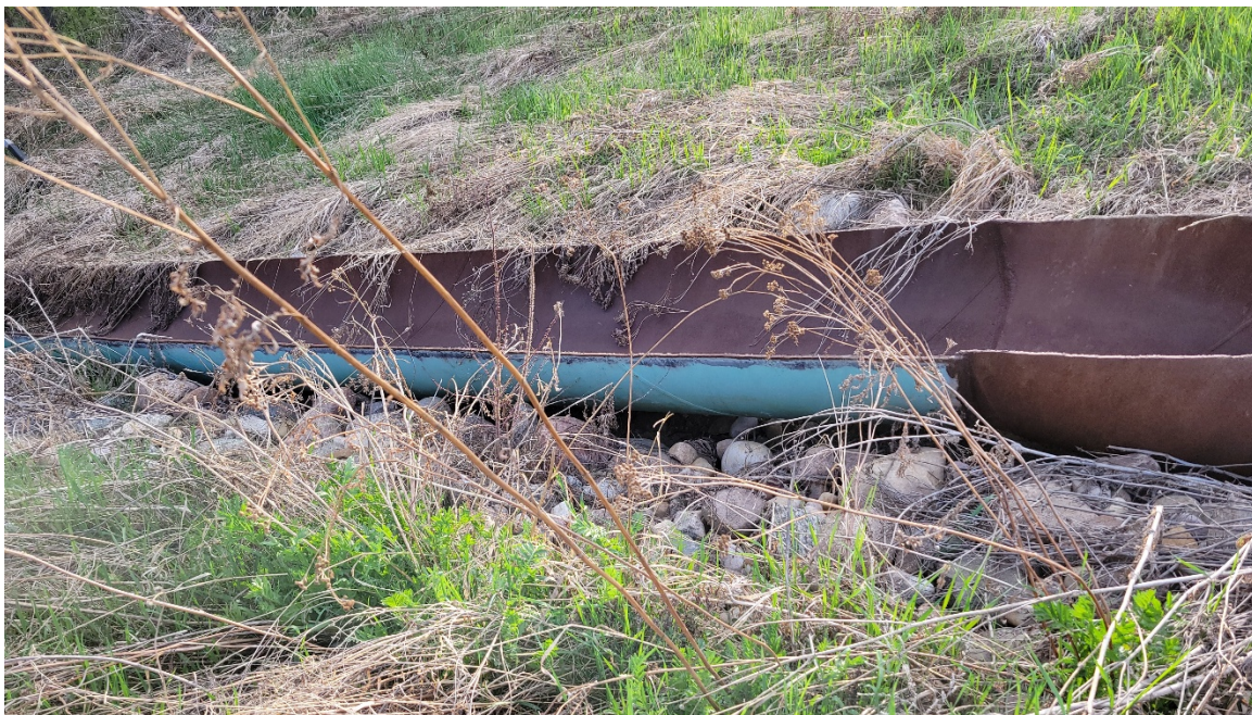
Photo 10. Outlet of culvert C3, installed in 2021. There is a void below the half pipe extension piece.
