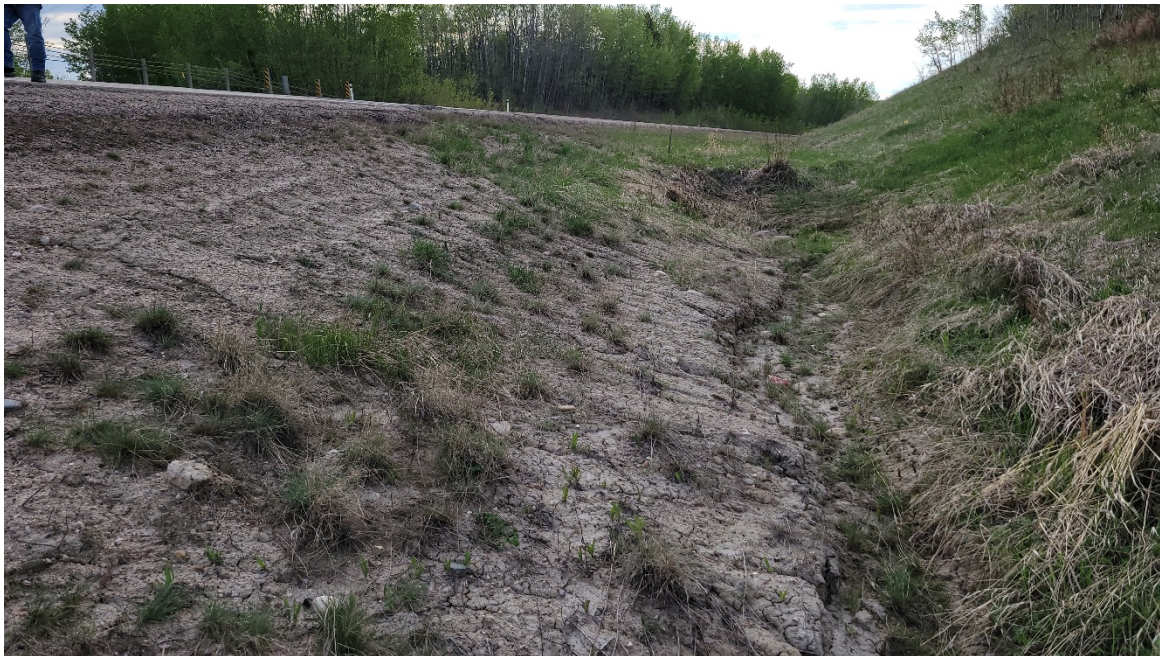
Photo 6. Looking west at the section of the north ditch regraded in 2019; side slopes and sections of the ditch bottom are still bare of vegetation; note the presence of erosion rills along the side slope and a deep erosion gully in the ditch.
