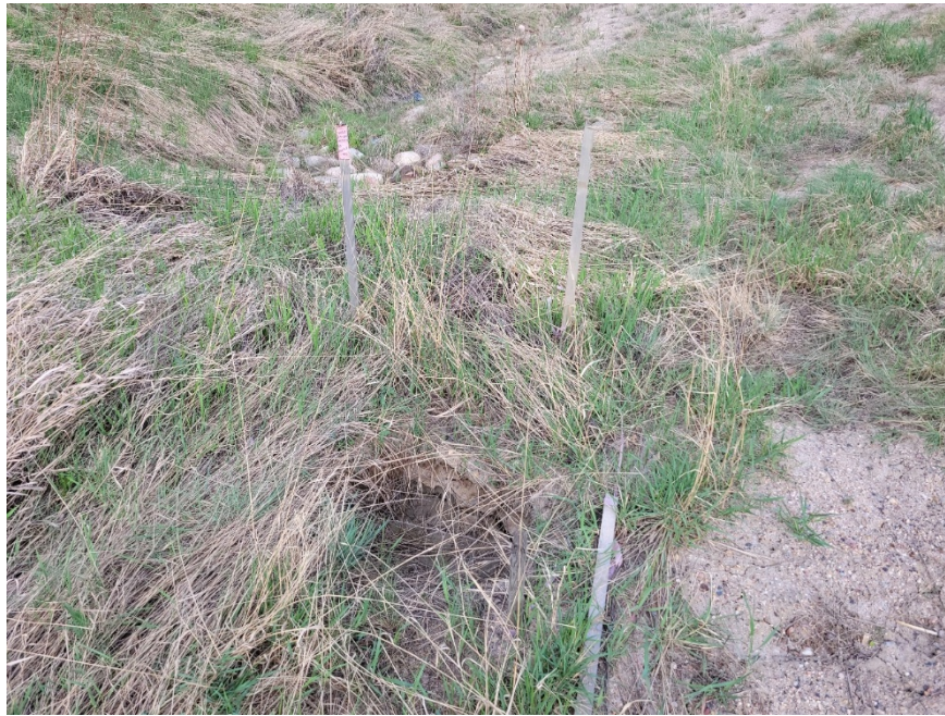
Photo 9. Sinkhole (800 mm long x 500 mm wide x 400 mm deep) west of the C3 culvert inlet.
