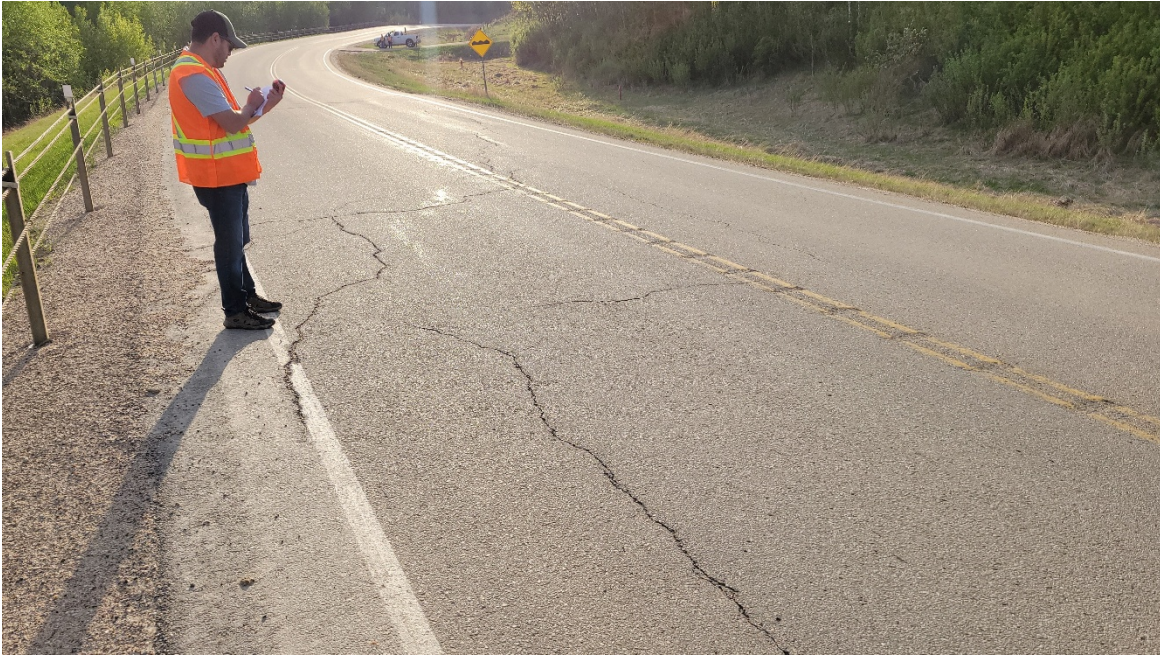
Photo 5. Looking northwest at diagonal cracks about 15 m east of the landslide eastern flank (up to 50 mm wide with 20 mm drop).
