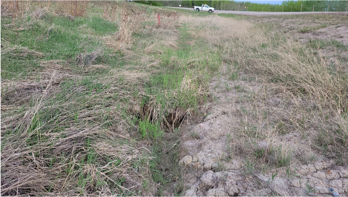
Photo 1. Looking east at a sinkhole that has developed at the start of the erosion gully in the highway north ditch. The sinkhole is 1300 mm wide, 500 mm long and 600 mm deep.
