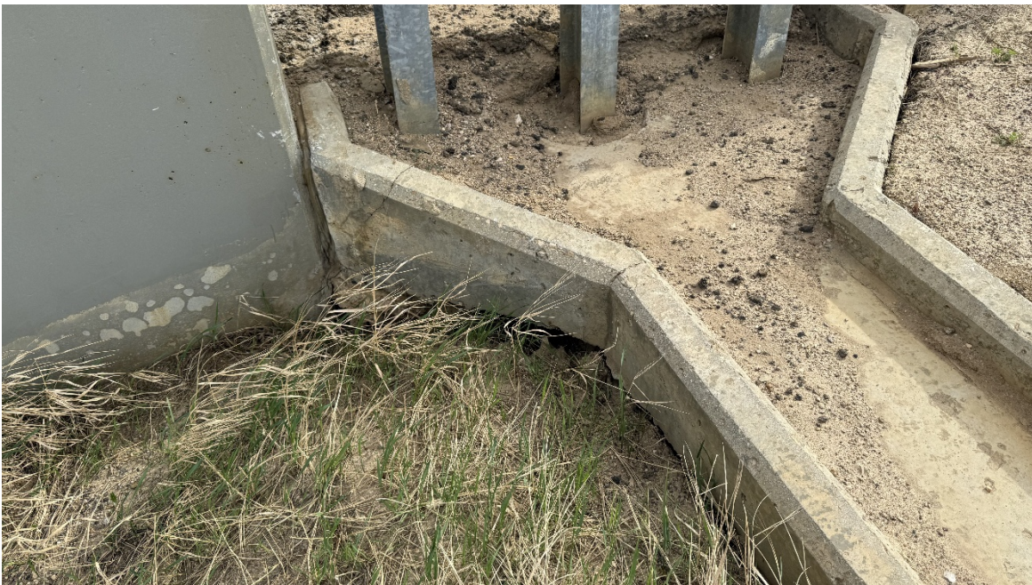
Photo 4. View of drain trough. A flexible filler was placed in 2024 to seal the 50 mm wide separation gap between the northwest wing wall and the drain trough. However, there is a gap beneath the drain trough in response to fill settlement (up to 100 mm wide and 150 mm deep).
