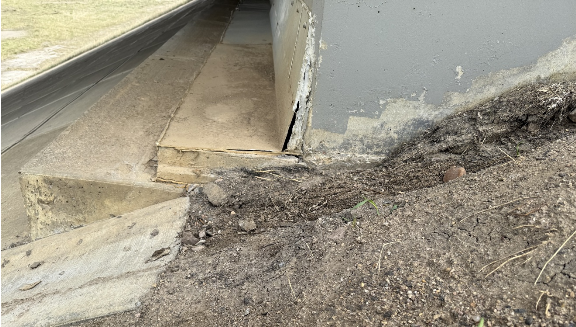
Photo 5. Looking south at north end of abutment seat. Grout was placed between the 2023 and 2024 inspections to fill a void that had developed under the abutment seat.
