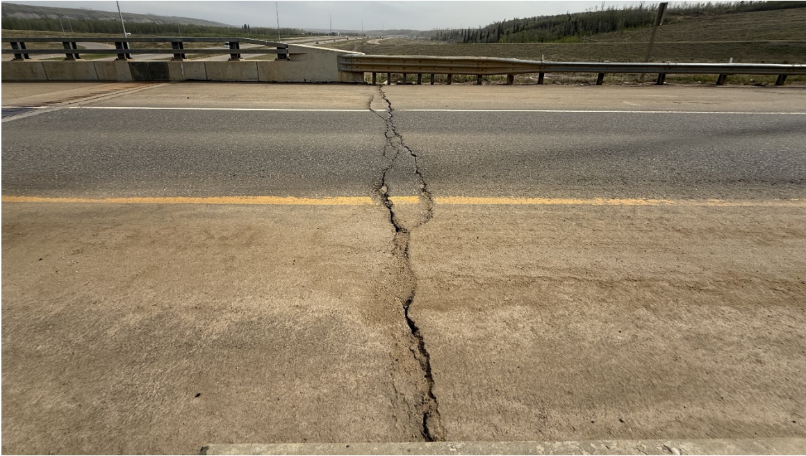
Photo 3. Looking south at the eastbound lane. Cracks are up to 40 mm wide and 30 mm deep.
