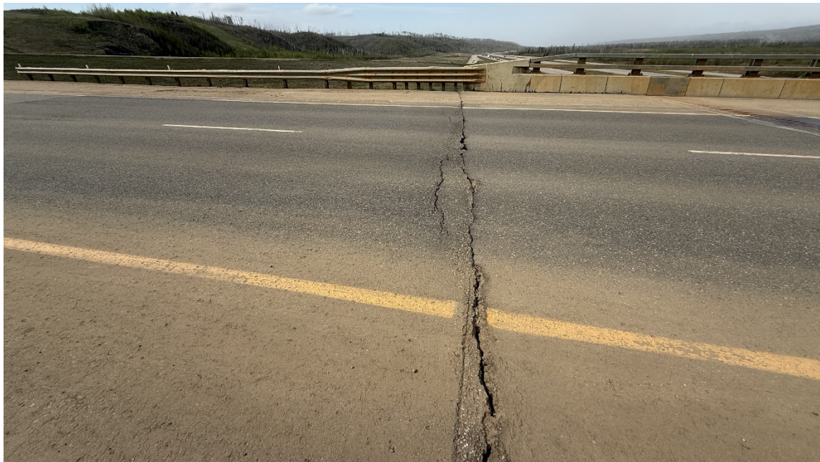
Photo 2. Looking north at same crack from Photo 1
