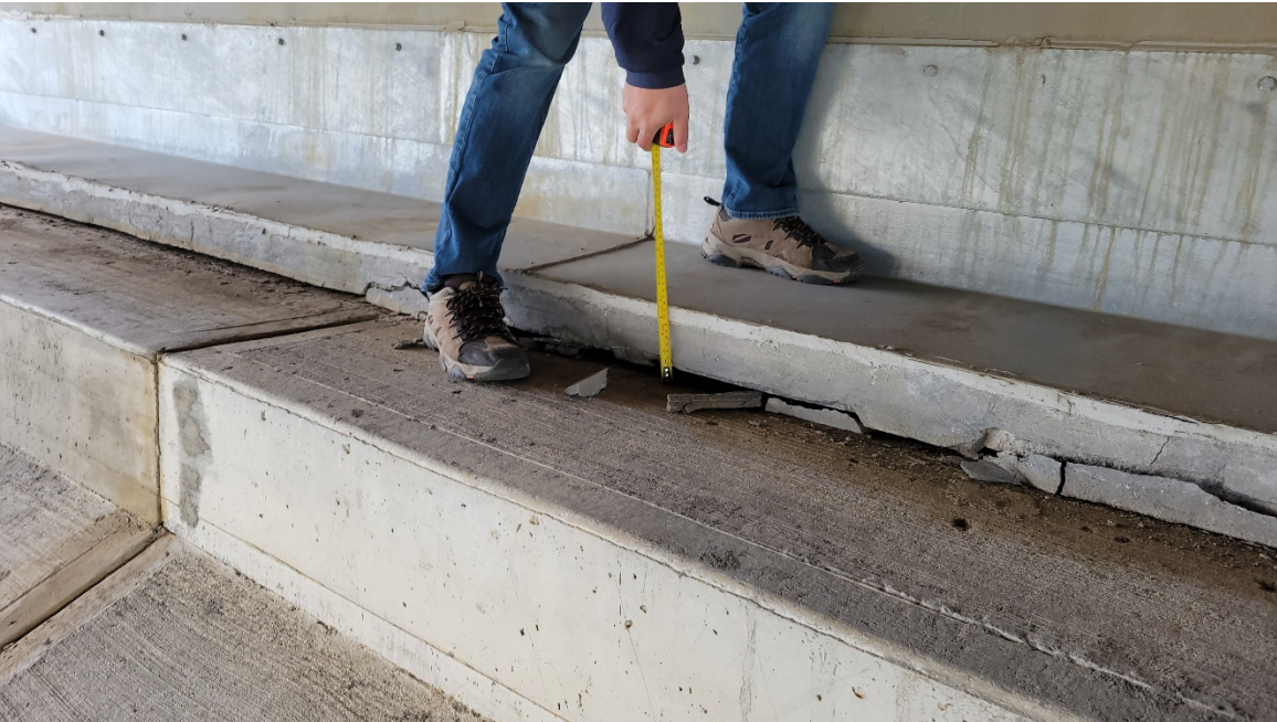
Photo 6. Gap of up to 30 mm has developed between abutment seat and grout fill that was placed between 2024 and 2025 inspections.
