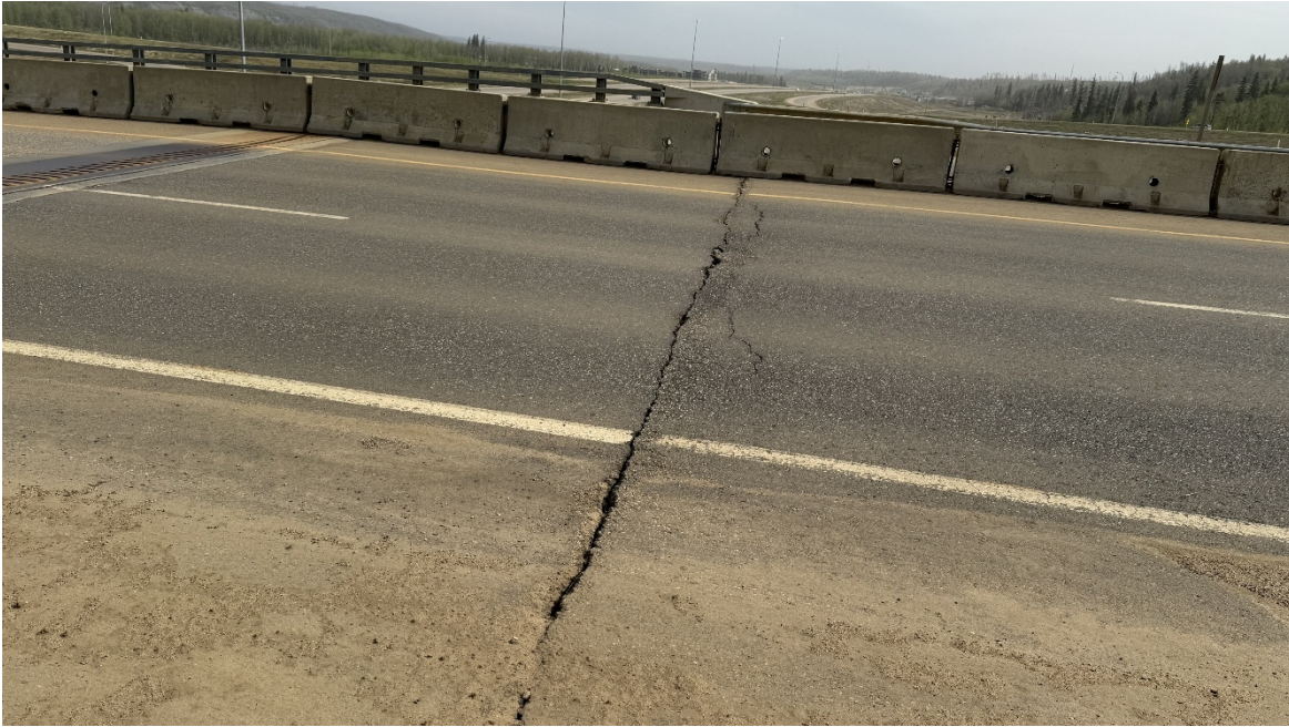
Photo 1. Looking south at the crack developed across the westbound lanes towards the median. The main crack is 30 to 70 mm wide and 30 to 200 mm deep. The cracks are across both traffic lane directions and have formed between the approach slab and the pavement, about 6 m west of the west abutment fingerplate. Fatigue cracking is visible west of the main crack.
