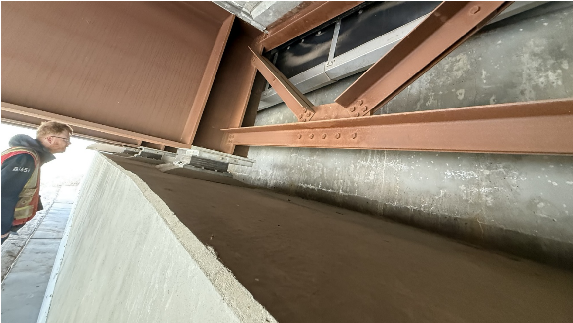
Photo 7. Bridge bearings appear to be maxed out.
