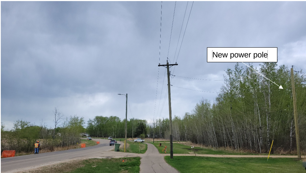
Photo 6. Looking north from the east side of the highway at Power Pole No. 2, which has a much less pronounced tilt since the anchor pole has been removed. Note the new power pole installed after the 2024 inspection.
