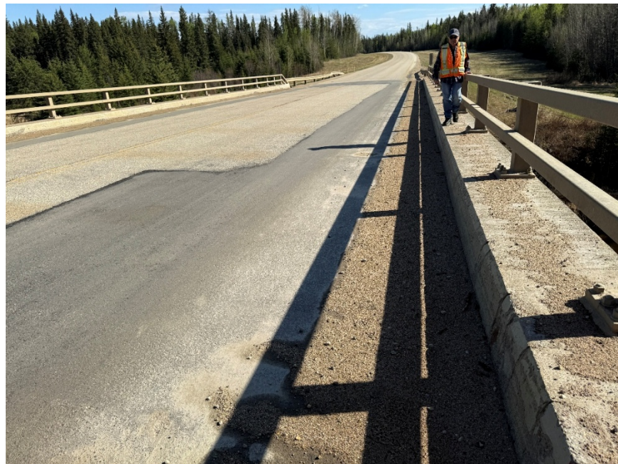
Photo 6. Patched area of previously failed pavement on bridge deck (looking south)
