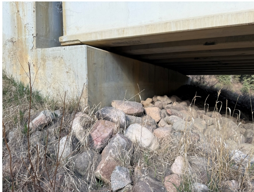
Photo 2. North Abutment (looking east) showing riprap placed by TEC in 2021; The riprap top surface appears to have dropped for a distance of about 10 m along the face of the abutment seat and the riprap along this zone shifted laterally towards the river.
