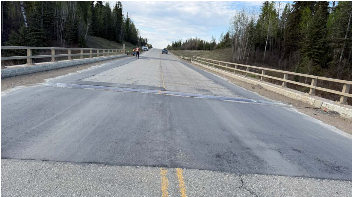
Photo 12. Looking north at the overall bridge deck surface condition. Note new ACP patch placed in 2024.
