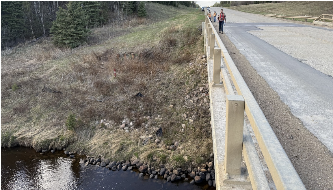
Photo 1. Landslide area viewed from bridge (looking north).
