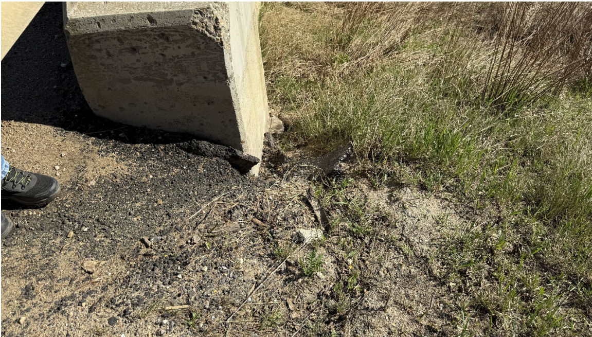
Photo 9. Void that had formed between the highway side slope and the top edge of the NE wingwall has been filled with ACP since the 2024 inspection.
