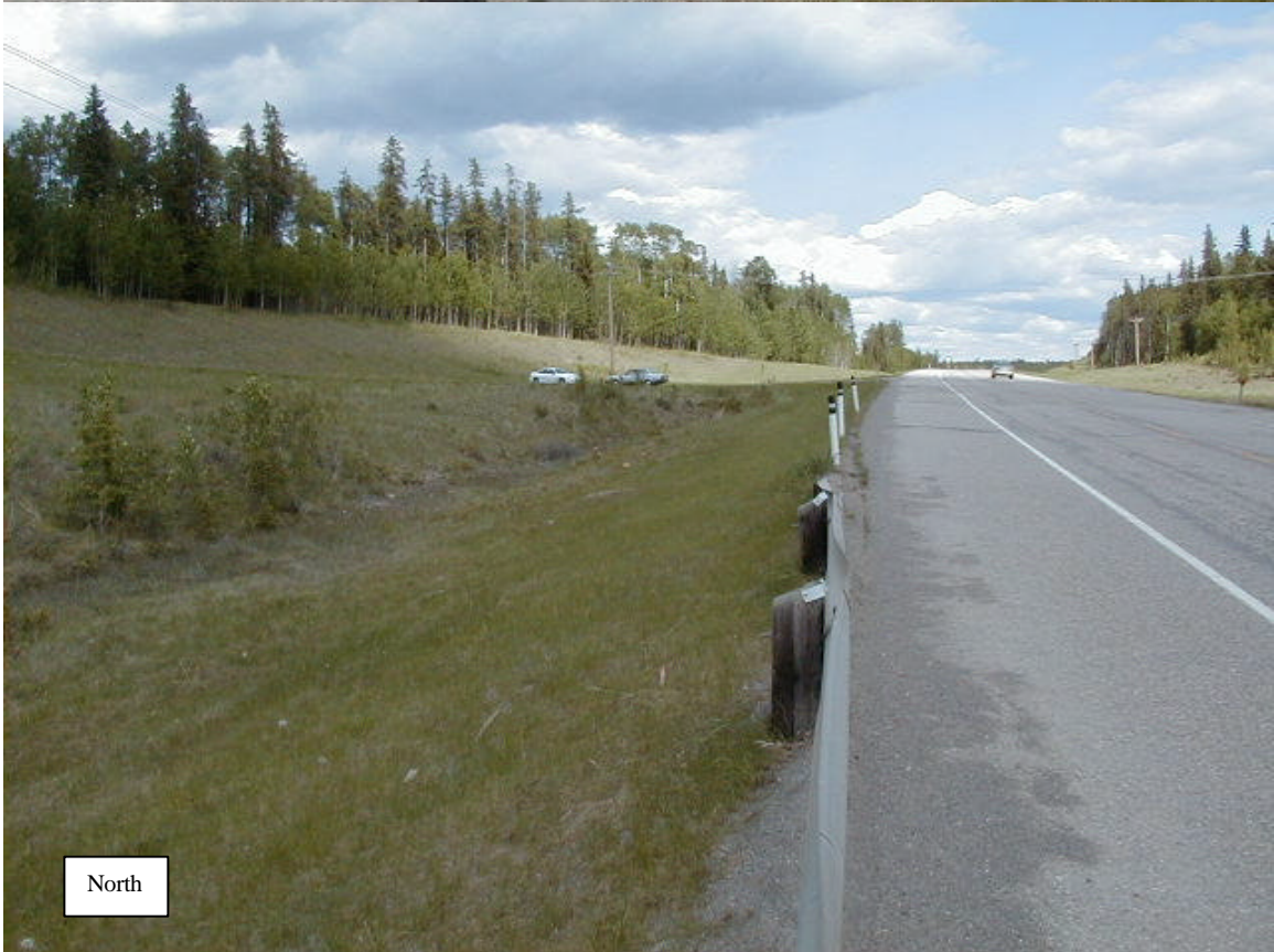
Standing water in north ditch
