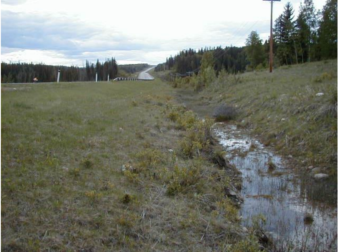
Standing water in north ditch
