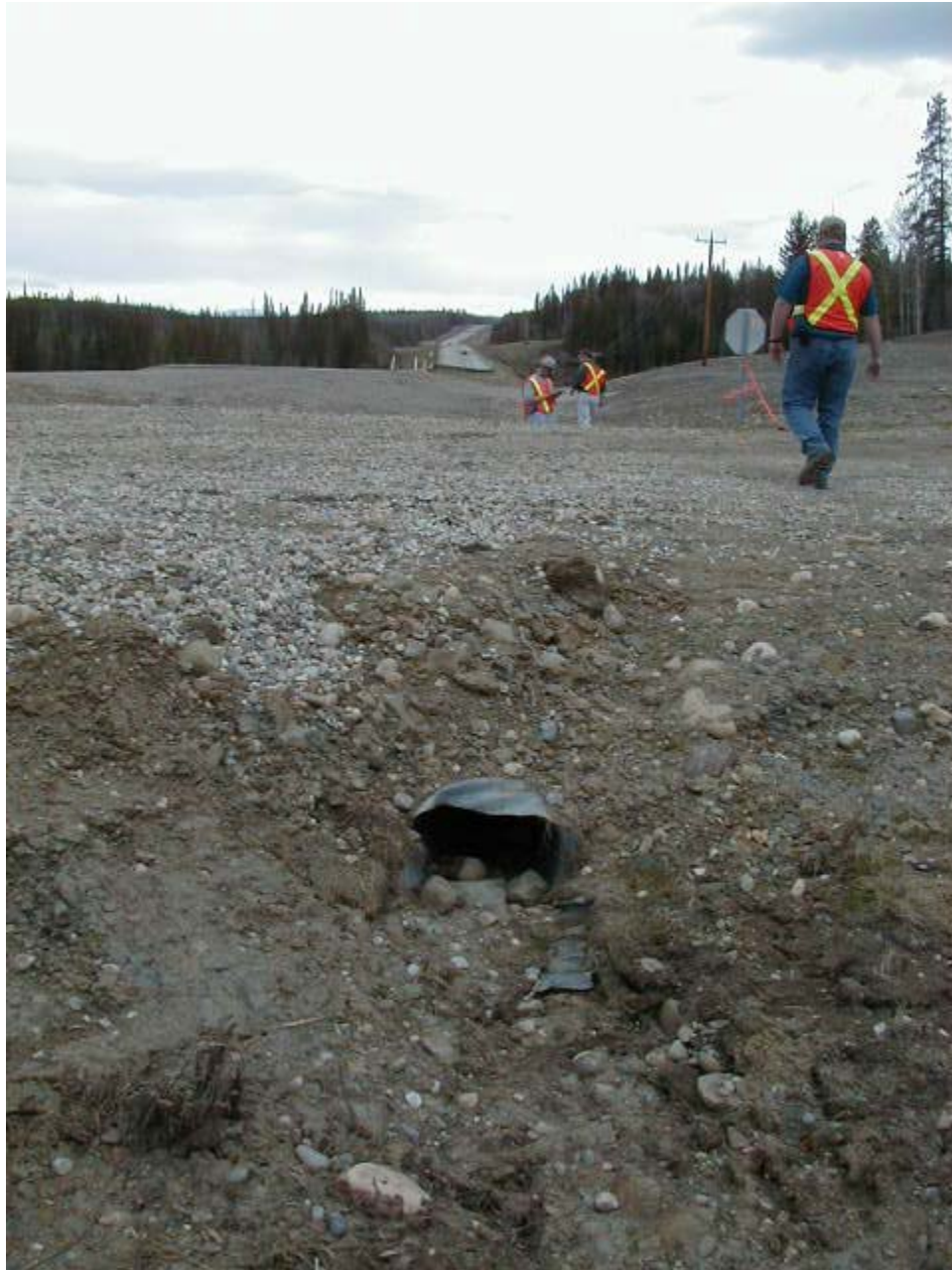
Looking west along north ditch from east of access road. Note partial blockage of culvert.
