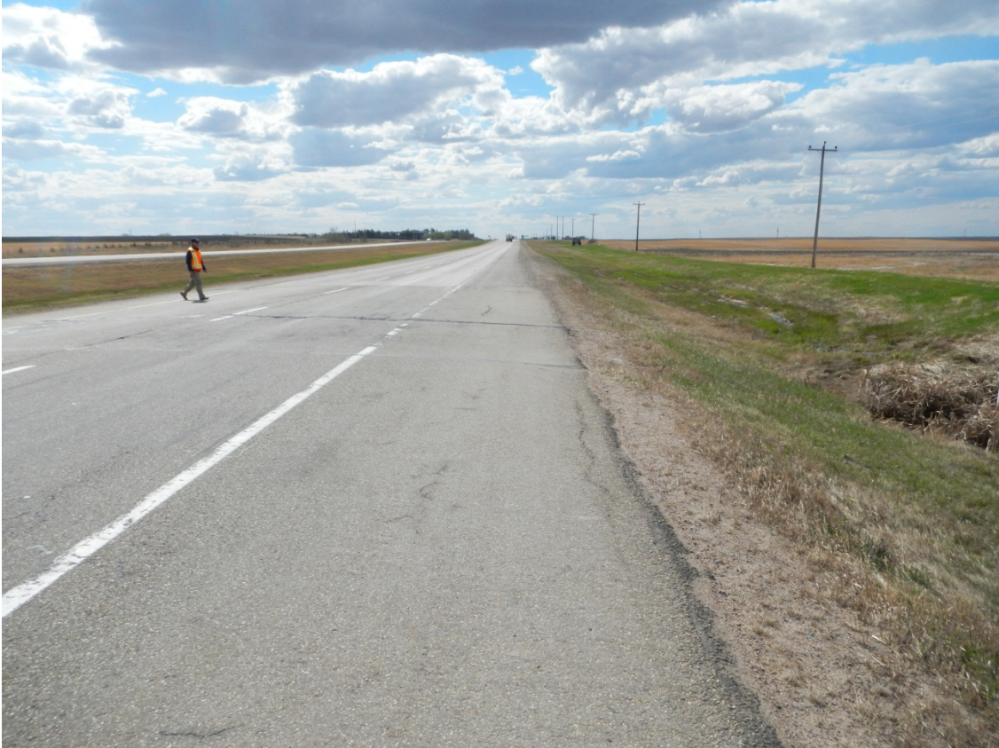
Ponded water north of highway
