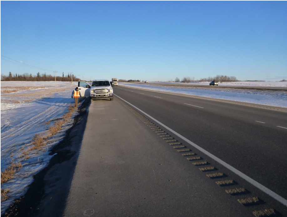
Photo 1 Location of repaired lateral cracking along the highway above the culvert backfill. Photo taken on February 28, 2018 looking east.
