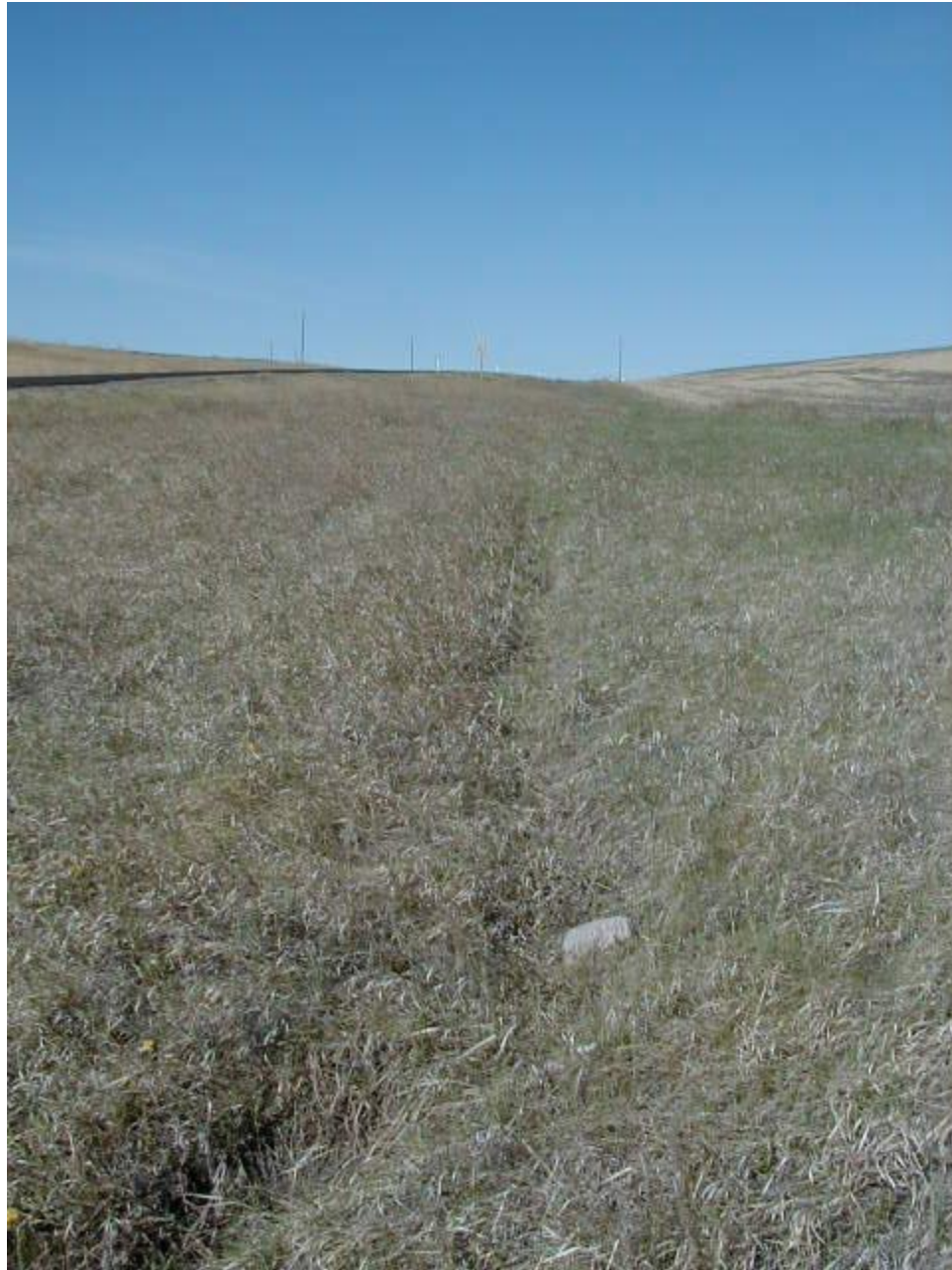
Looking west at small erosion channel forming on north side of highway
