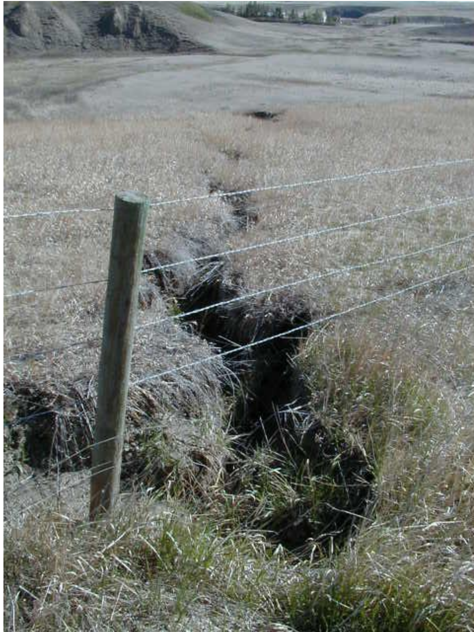
Looking north at erosion channel leading to large gully down to the toe of the embankment
