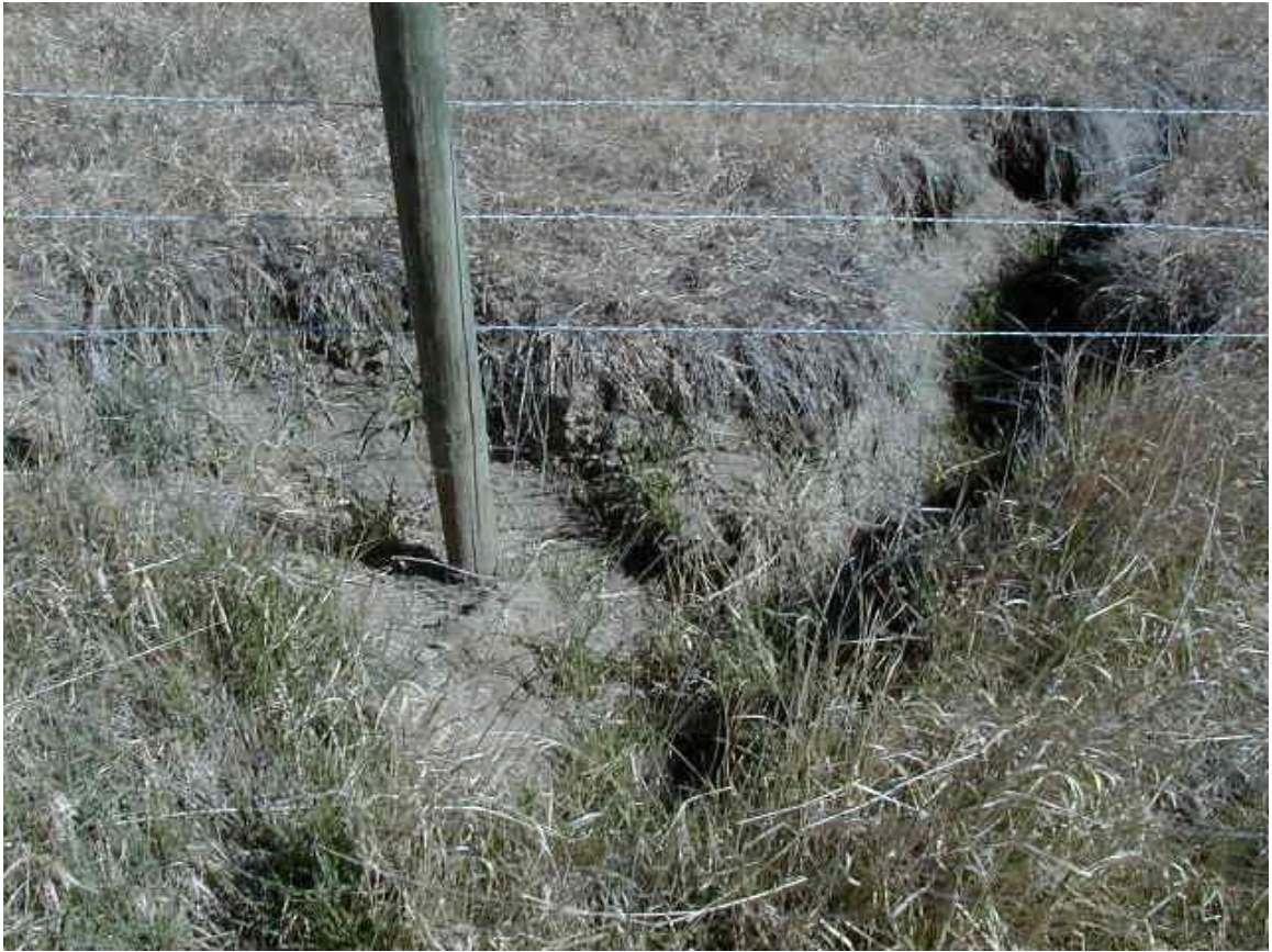
Erosion channel at fenceline
