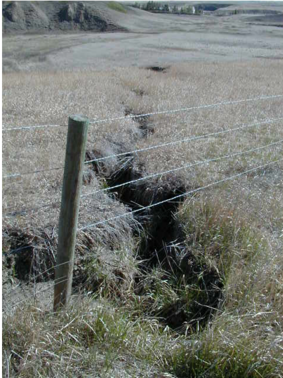
Looking north at erosion channel leading to large gully down to the toe of the embankment
