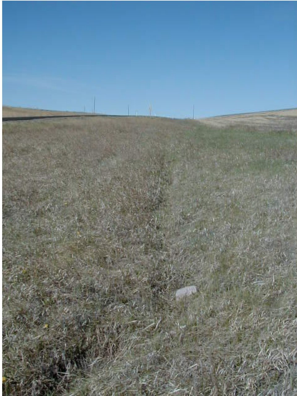
Looking west at small erosion channel forming on north side of highway
