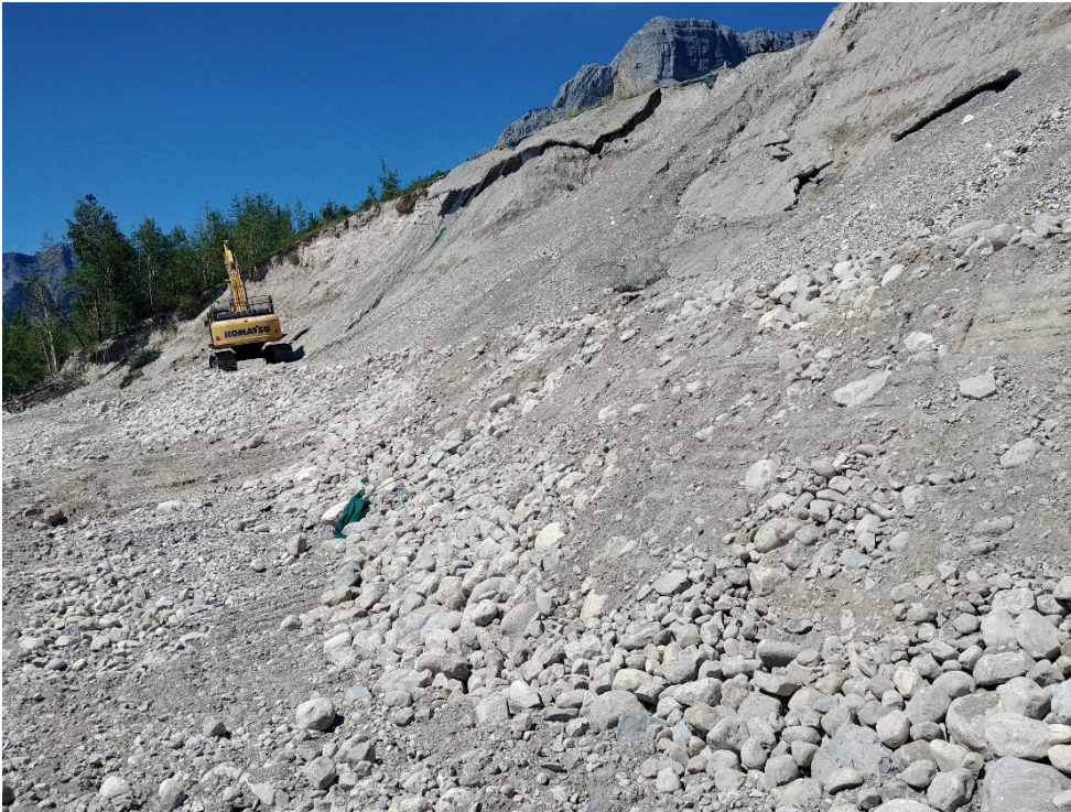
Photo 7 Close-up view of the finished temporary berm slope comprising cobbles, gravel, and sand from the beach. Photo taken July 22, 2019 looking northwest.
