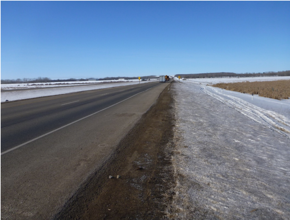
Photo 5 Location of frost heave site (east section). White posts indicate drain outlets. Photo taken on February 28, 2018 looking west.
