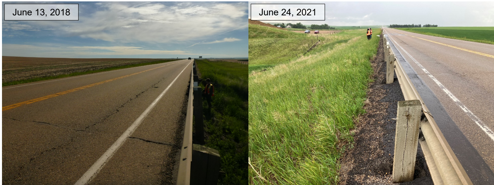
Photo 2 Longitudinal cracking in the eastbound lane before and after repairs were completed. Photos taken June 13, 2018 and June 24, 2021 looking northeast and southwest, respectively.
