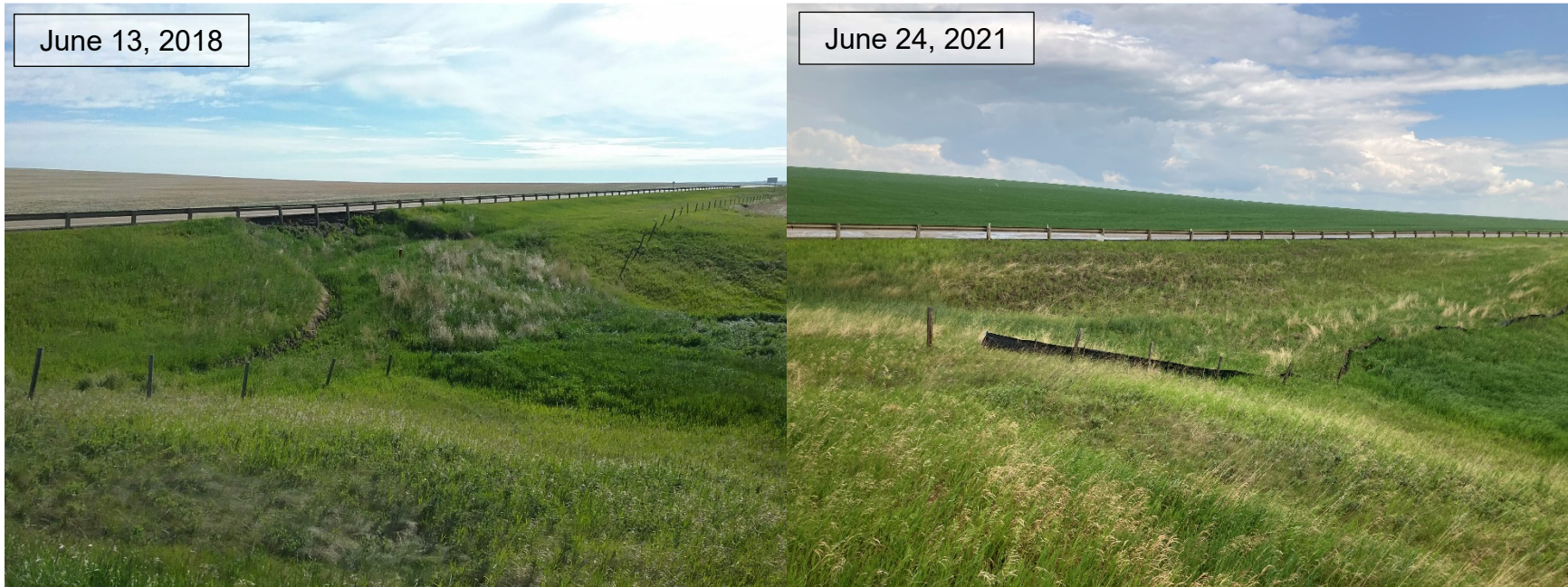
Photo 1 An overview of the C070W slide area, before and after repairs were completed. Photo taken June 13, 2018 and June 24, 2021 looking northeast.
