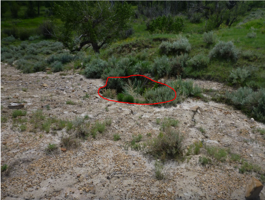
Photo 6 Large sinkhole (red outline) at the toe of the south slope below highway at C058-III (waypoint 691) has not expanded since 2018 inspection. Photo taken July 10, 2019 looking south.
