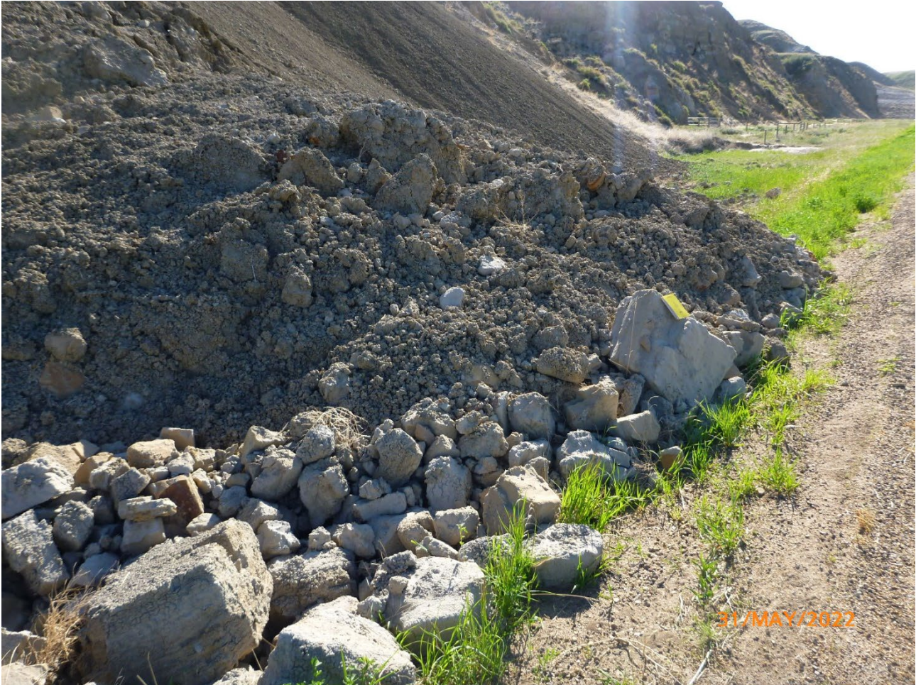
Photo 3 Failed material accumulated in the ditch. Photo taken May 31, 2022, facing east.
