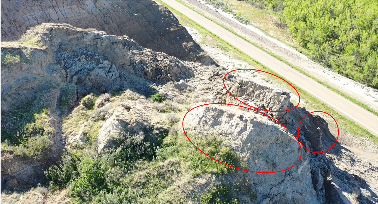
Photo 7 Oblique photo behind the three weathered rock blocks. Photo taken from the UAV on May 31, 2022, facing south.
