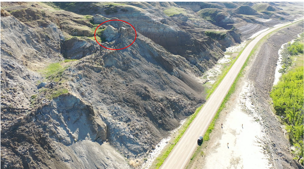
Photo 8 Oblique photo of the three rock blocks on the east side of the slope. Photo taken from the UAV on May 31, 2022, facing east.
