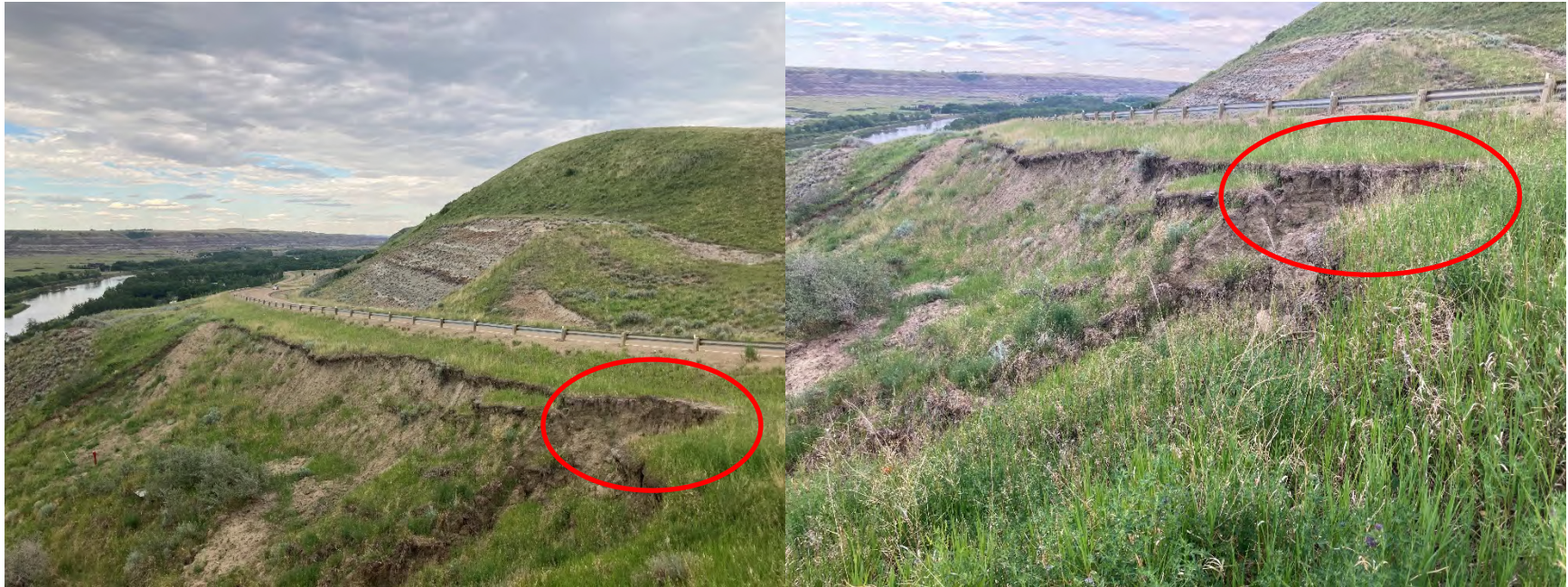
Photo 4 The headscarp of the C017-III slide is approximately 1.5 m to 2.0 m in height. The area of the headscarp that has retrogressed towards the highway since 2020 is indicated by red circles. Photos taken June 23, 2021 looking southeast.
