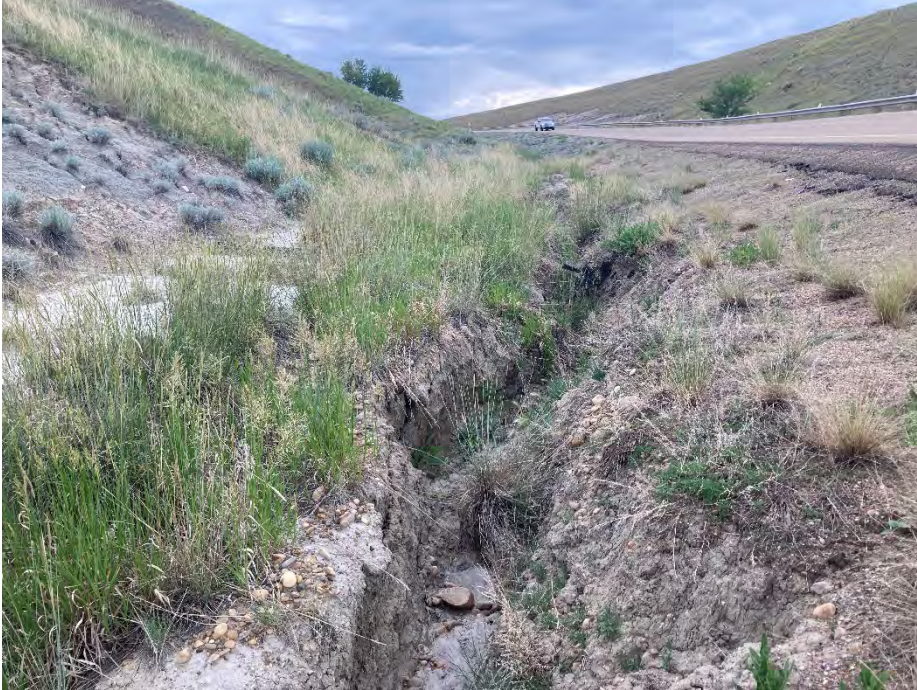
Photo 5 Gully erosion in the ditch south of Hwy 575 has expanded slightly since 2020. Photo taken June 13, 2021 facing north.
