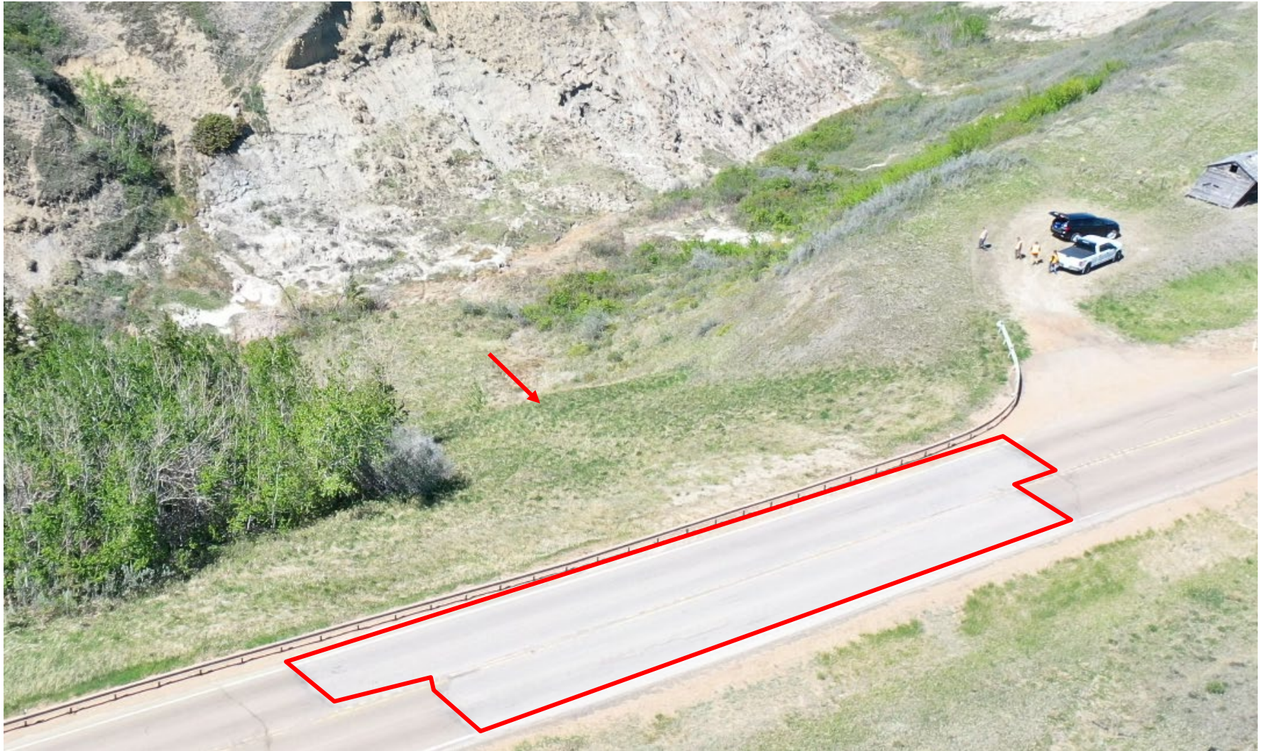
Photo 2 Aerial photo of the C019 site from the upslope (south) side of Hwy 575:04, showing the failing geogrid reinforced lower slide (indicated by red arrow) and pavement patch (indicated by red polyline). Photo taken May 30, 2022, facing north.
