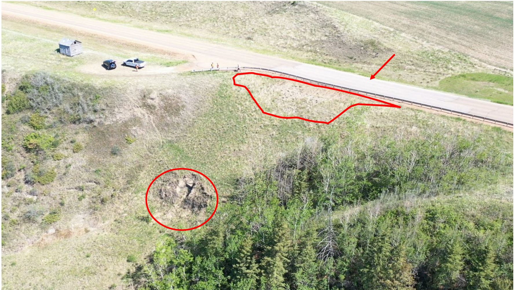
Photo 1 Oblique view of the C019 site, indicating poor vegetation cover at the top of the highway embankment (indicated by red polyline), the failing geogrid reinforced lower slide completed in late-2010 or early-2011 (indicated by red circle), and previous pavement patch (indicated by red arrow). Photo taken May 30, 2022, facing southeast.
