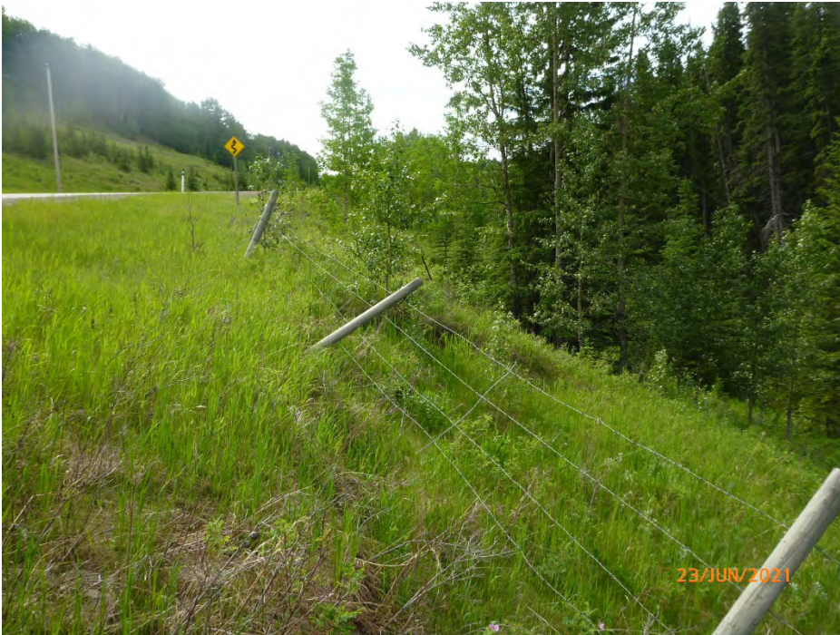
Photo 2 Fence downslope of Slide Area No. 4 has tipped over (roadway remains unaffected). Photo taken June 23, 2021 facing east.
