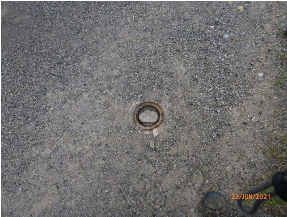
Photo 4 Flush-mounted headbox is missing its cap and require replacement. Photo taken June 23, 2021.
