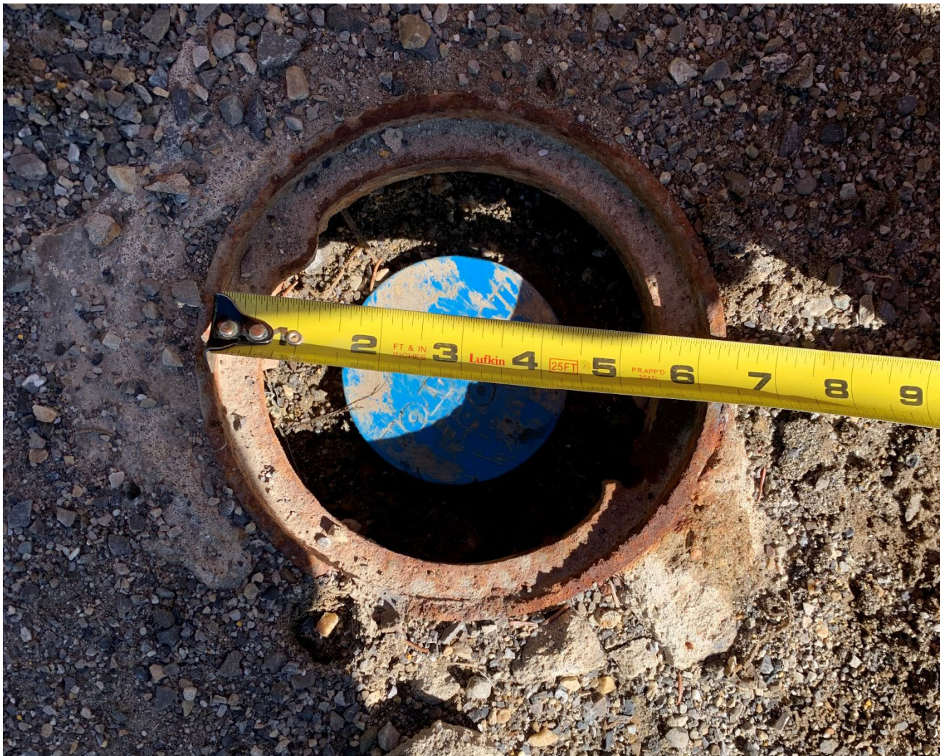
Photo 1 Flush-mounted casing protector installed in the south shoulder of Hwy 579:02 to protect the SI05-07. Photo taken June 15, 2021.
