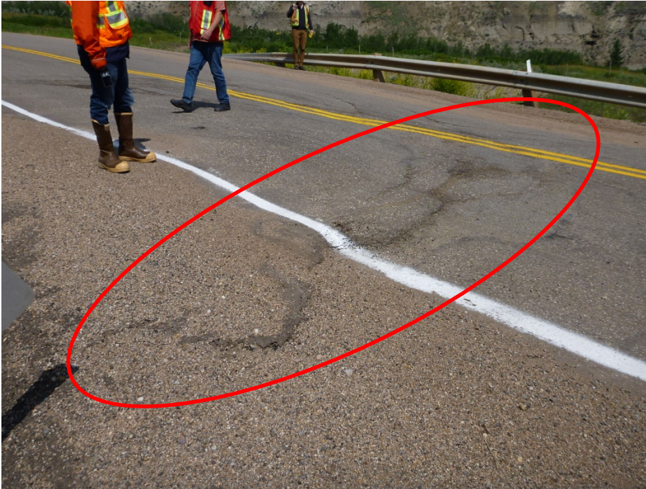
Photo 3 Close-up view of toe roll in pavement (red circle) caused by heavy trucks braking in the eastbound lane as they approach the C065-I site. Photo taken July 11, 2019 looking northwest.
