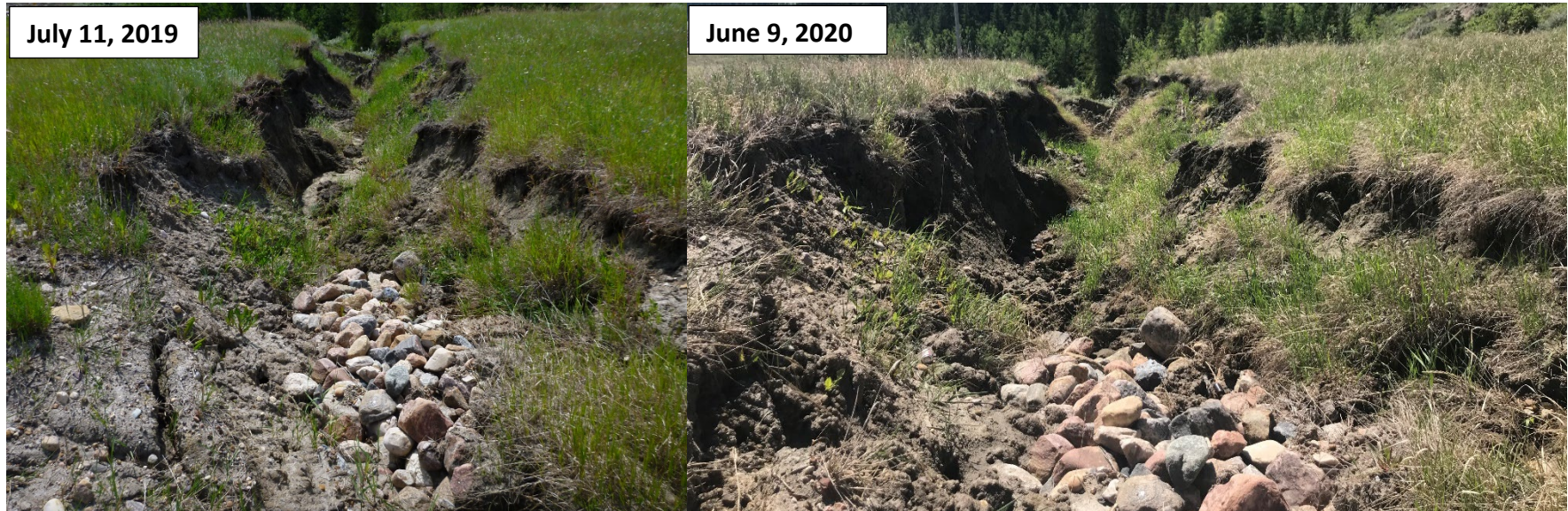
Photo 1 Comparison photo of the existing erosion gully on the south side (eastbound lane) of the highway, approximately 600 m west of the bridge. Gully appears to have expanded since 2019. Photos taken looking south.
