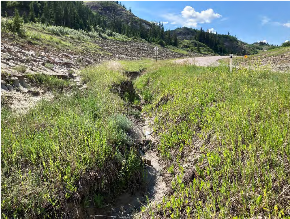
Photo 2 Continued erosion in the ditch south of Highway 590, upstream of the 1200 mm diameter CSP culvert. Photo taken June 24, 2021 facing west.
