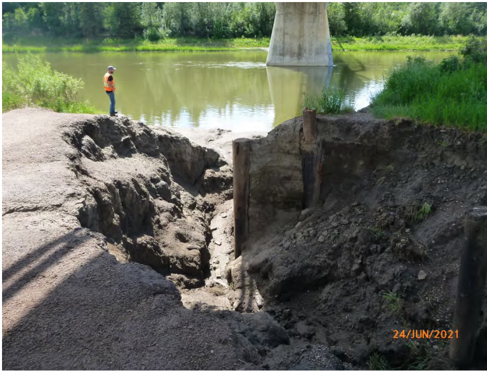
Photo 4 Erosion gully at the east abutment is larger than during the 2020 inspection. Photo taken June 24, 2021 facing west.
