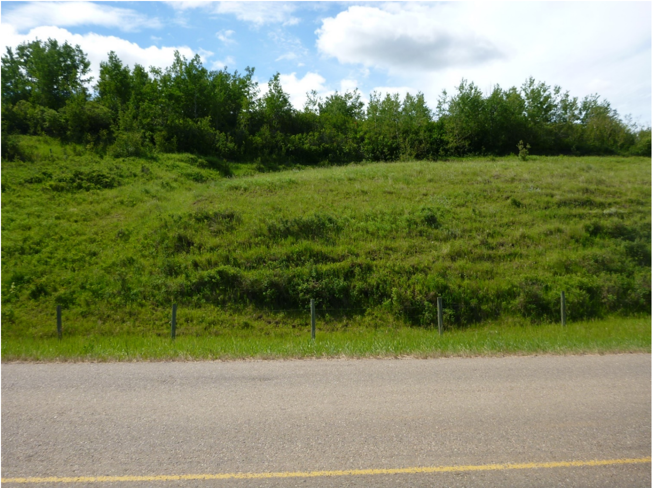
Photo 3 Slope movement in the slope south of Hwy 619:06. Photo taken June 24, 2020 facing south.
