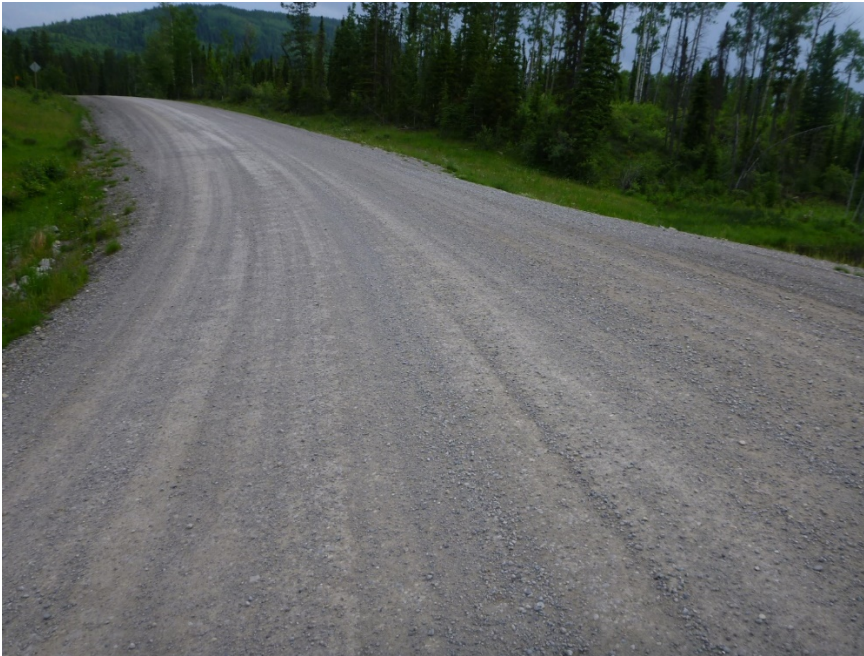
Photo 3 Super elevation reestablished in roadway at C037-II from grading operations since repair was completed in 2016. Photo taken July 9, 2019 looking south.
