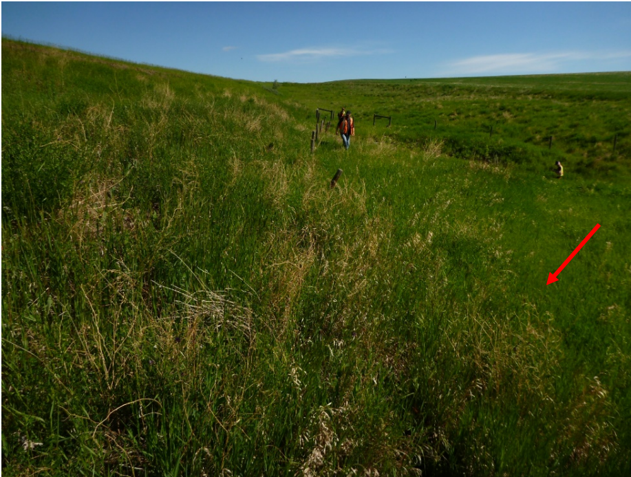
Photo 5 Area where the toe roll has extended beyond the fence line by approximately 3 m as indicated by the red arrow. Photo taken June 13, 2018 looking north.
