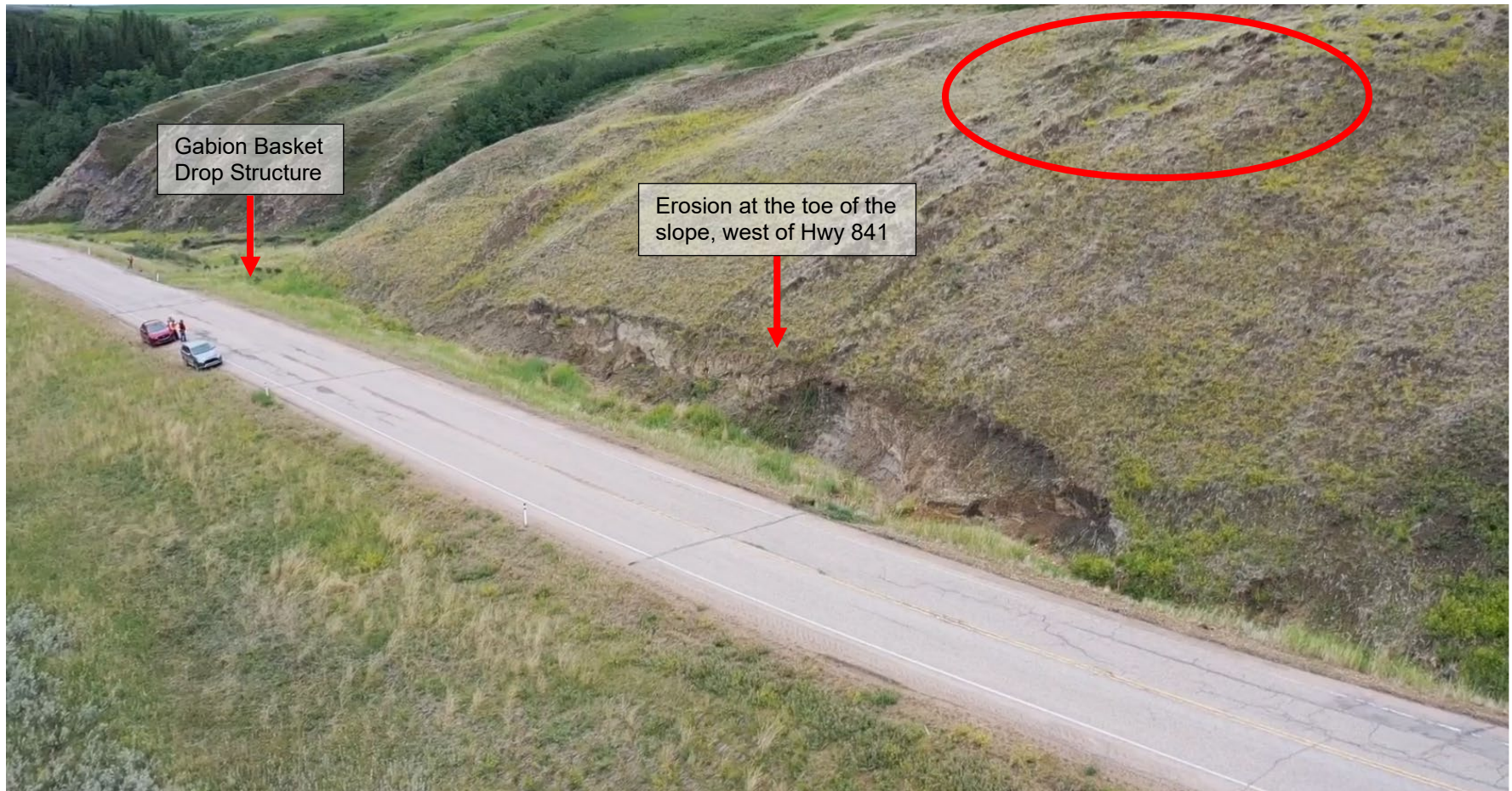
Photo 7 Gabion basket drop structure and ongoing erosion occurring at the toe of the slope, on the west side (southbound) of Hwy 841. Red circle indicates slope instability on private land influenced by oversteepening at toe of slope due to ditch erosion. Photo taken June 24, 2021 facing west.
