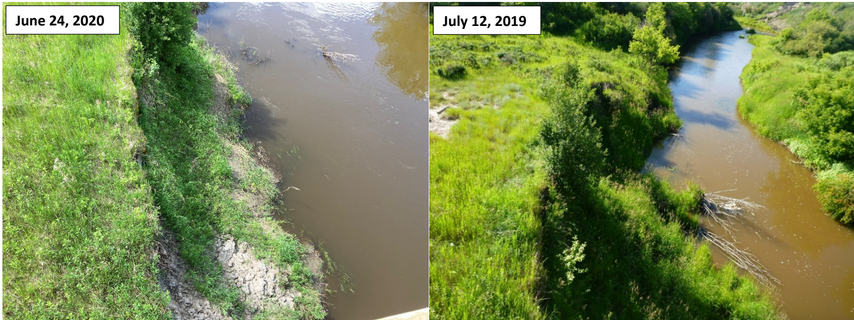
Photo 5 Slide on the south embankment of the Battle River (Photo from 2019 inspection included for comparison). Photo taken June 24, 2020 looking west.
