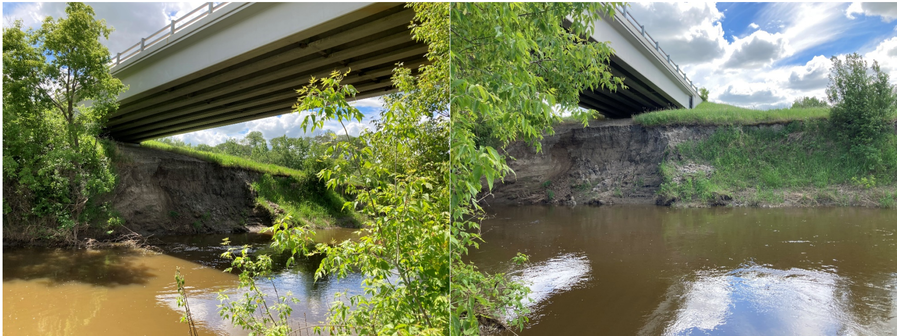
Photo 6 Unstable south abutment riverbank directly below bridge deck. Photo taken June 24, 2020 from the east and west side of the bridge, respectively.
