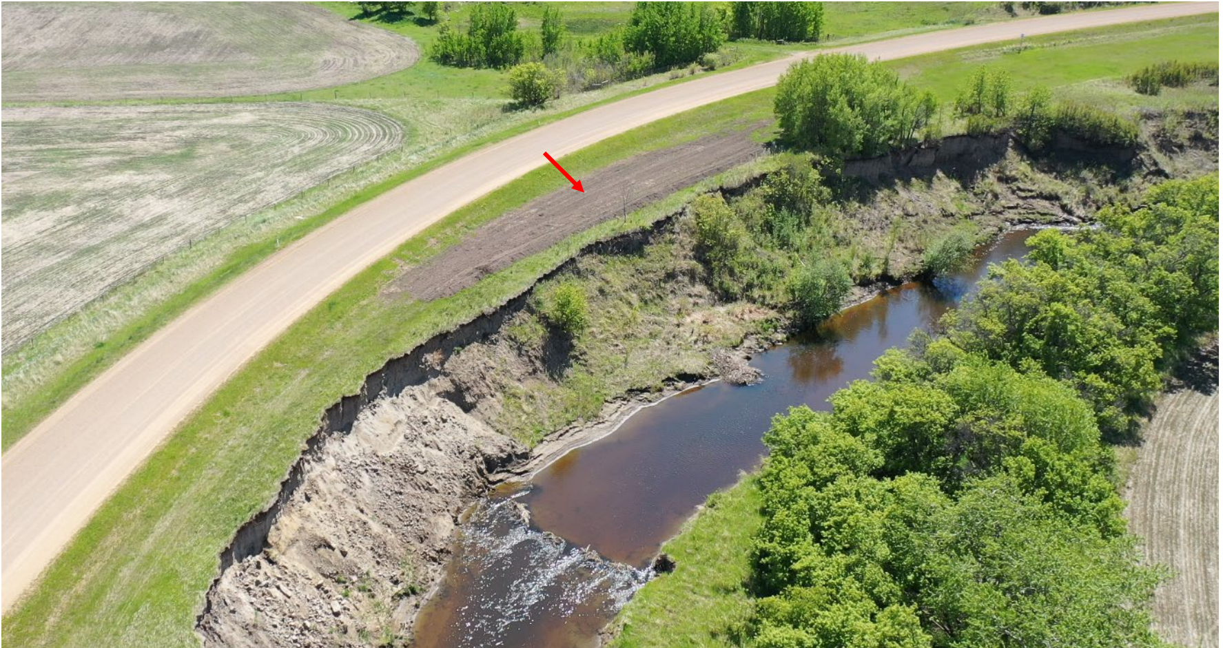
Photo 6 A length of the ditch near the southwest extent of the C055-II site where a berm was built to divert flow away from the eroding bank. Photo taken May 31, 2022.
