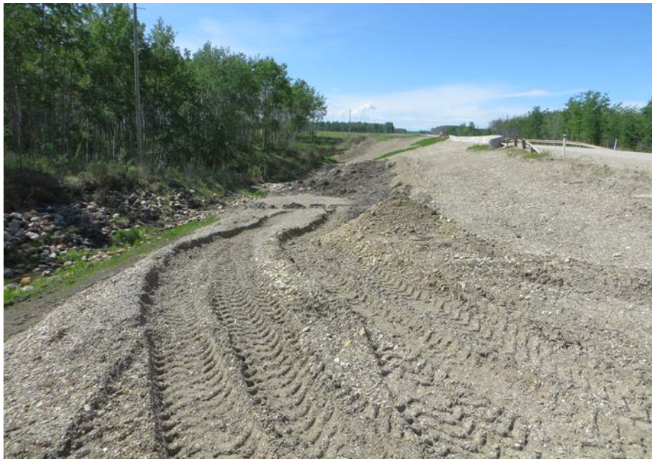
Photo 2 – Looking west along the south highway embankment slide area from the east end (construction on-going).
