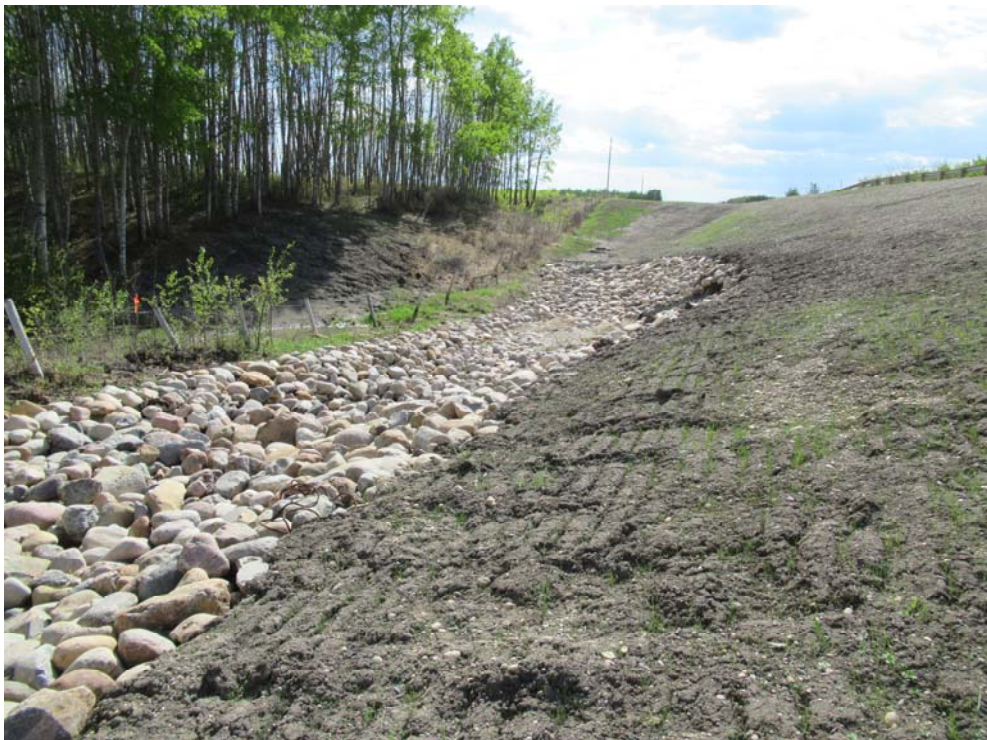
Photo 4 – Looking west along the toe of the repaired south highway embankment, and re-constructed riprap channel leading to the culvert inlet.
