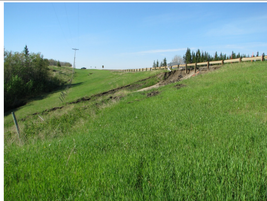
Photo 13. Looking along the east side of the road near 26+800. Three guardrail posts are now hanging
