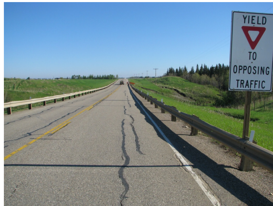
Photo 12. Looking northwards along the east side of the highway near 26+890. Backscarp has encroached into the northbound lane with traffic having to cross centerline to avoid.
