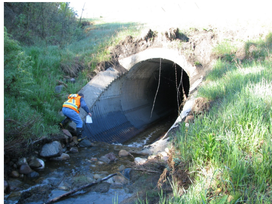
Photo 10. Looking southwest at culvert inlet. Slide material and barbed wire from fence originally situated about 23 m upslope of the culvert is now draped over the pipe.
