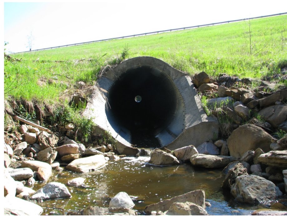
Photo 5. Outlet (west end) of the multi-plate culvert under the highway. No significant change since 2009.
