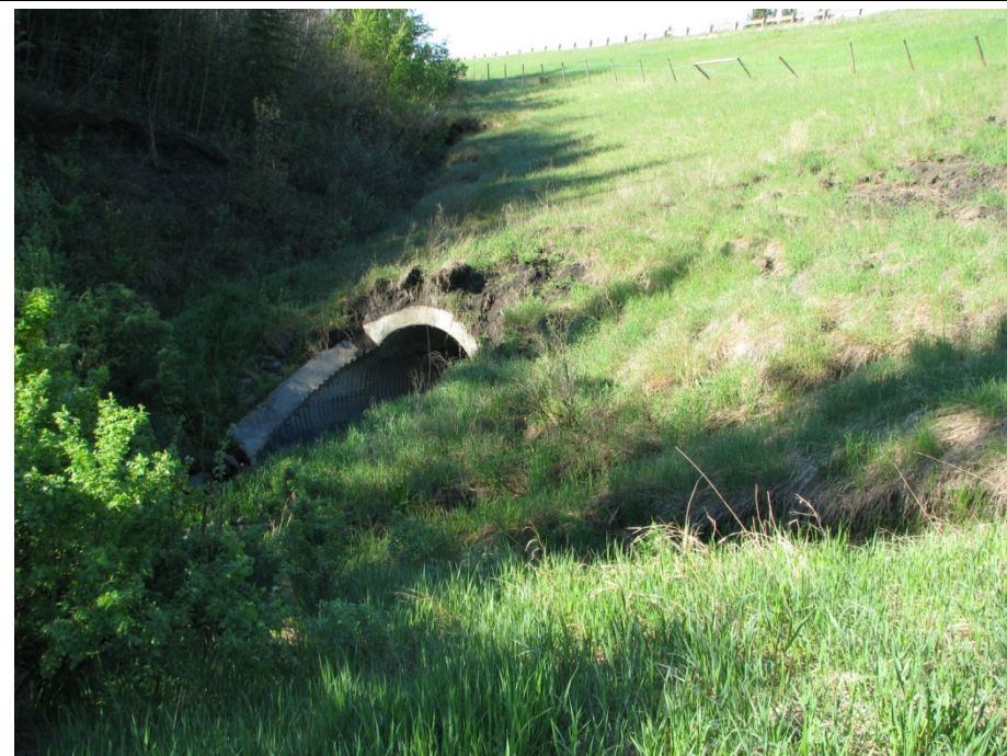
Photo 11. Looking southwest at toe of slide area. Slide debris continues to move gradually downslope towards the culvert inlet.
