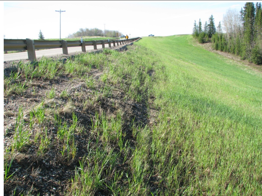
Photo 4. Looking south along the west side of the road. Winter highway salt is likely impeding vegetation growth below the shoulder.
