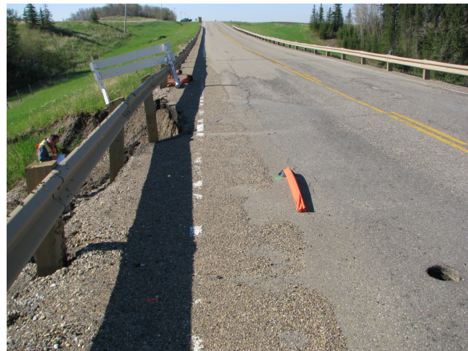
Photo 14. Looking southwards along the road near 26+800 at backscarp of east side slide which is encroaching about 0.7 m beyond the guardrail. Pavement cracks have grown in the middle of the northbound lane since 2012. Thurber test hole TH12-1 from September 2012 investigation can be seen in lower left corner.
