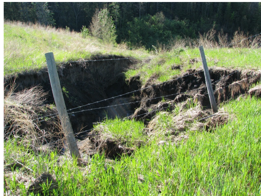
Photo 8. Ditch gullying at upper portion of the ditch at the NE corner of the site has extended further north and west than observed in 2012.
