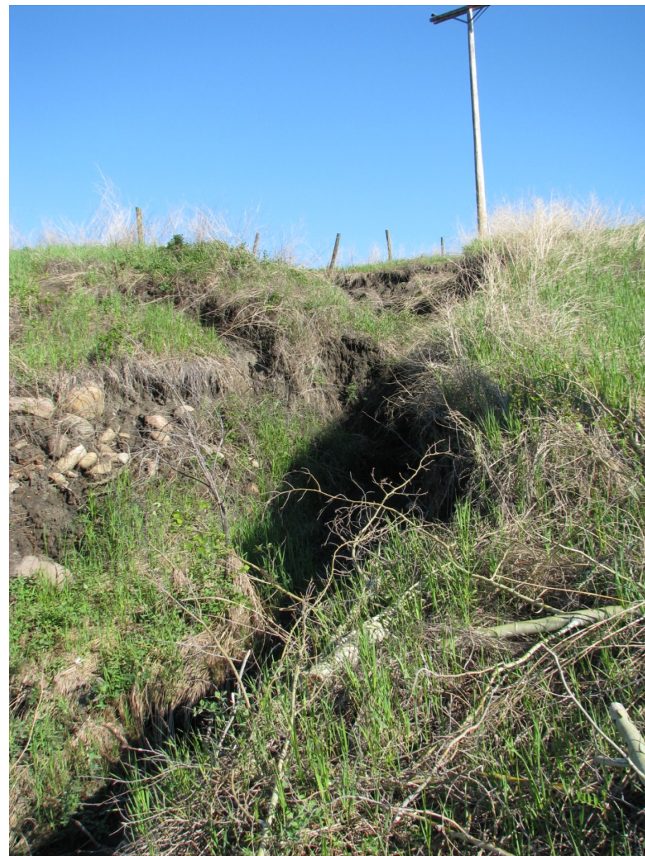
Photo 7. Middle portion of the ditch in the NE corner of the site has worsened since 2012 with the gully sidewalls failing and falling into the bottom.
