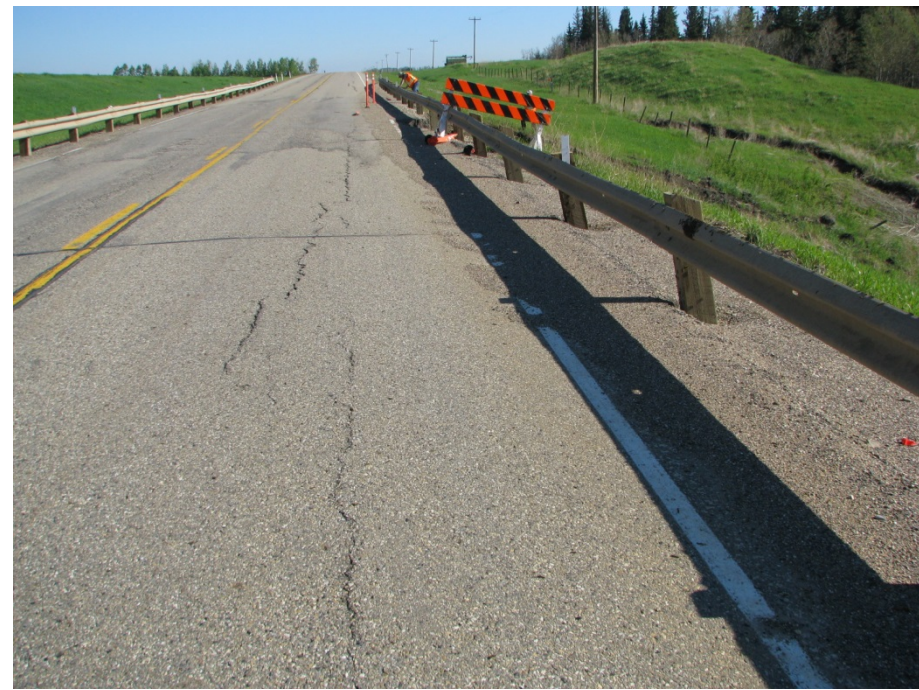
Photo 15. Asphalt cracking extends south of patched area.
