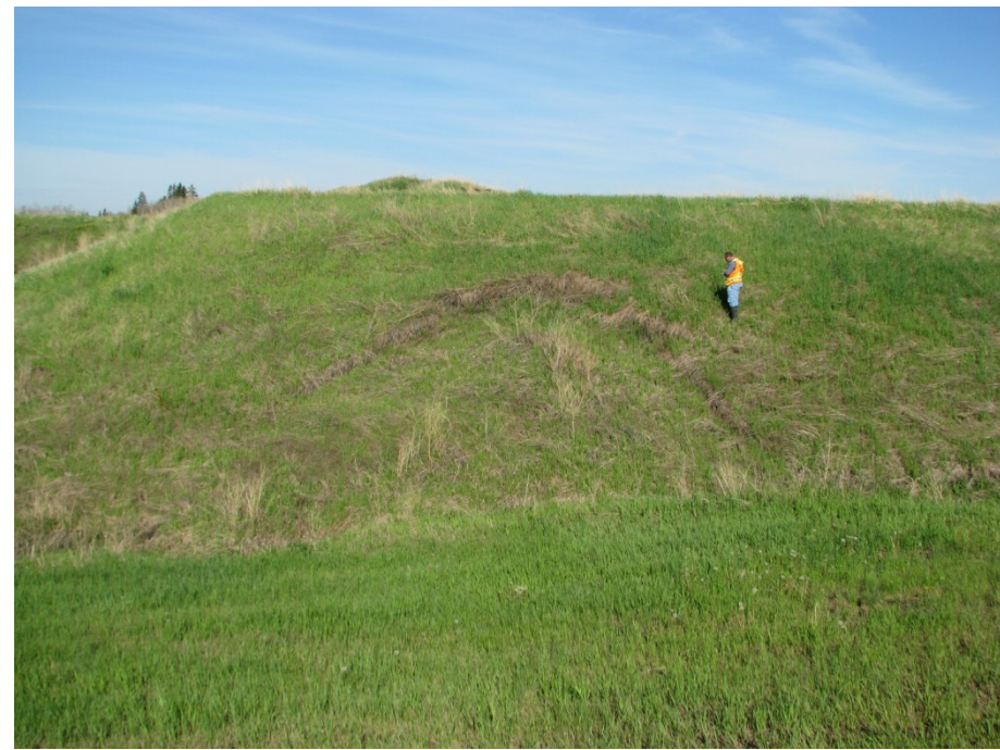
Photo 2. Slump in the NW corner of the site. No significant change since 2012.
