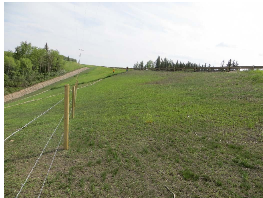
Photo 10. Looking south from northeast ditch at new type A fence and main landslide repair in highway sideslope. The failed rea was excavated in the fall of 2013 and backfilled with pit run gravel with a subdrain placed at the base extending into the centerline culvert inlet rip bowl. The disturbed area was then capped with clay, topsoiled and seeded in June 2014.
