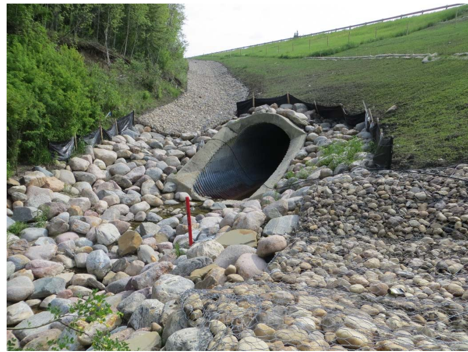
Photo 12. Looking southwest at the highway centerline culvert inlet. The landslide debris had buried the culvert inlet in 2013. The culvert clay cap was exposed and the rip rap replaced and enhanced to accommodate the gabion mattress tie-in overlaps from the northeast and southeast ditches.
