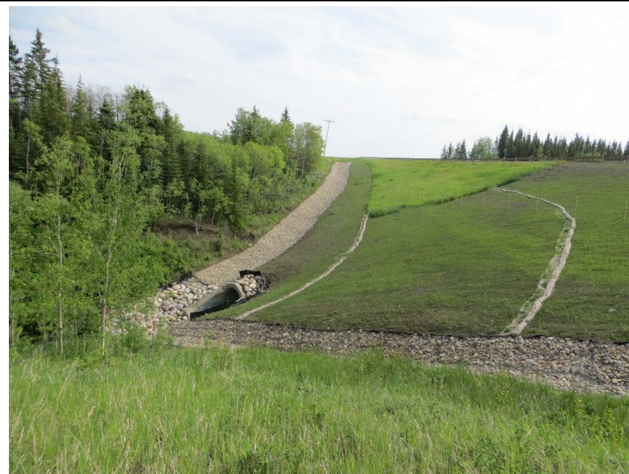
Photo 11. Looking southwest at culvert inlet. Two biodegradable sediment control devices were placed diagonally across the repaired sideslope to shed the water gradually towards the gabion mattresses. Vegetation along the constructed sideslope is relatively sparse when compared to the existing grass of the undisturbed sideslope in the background.
