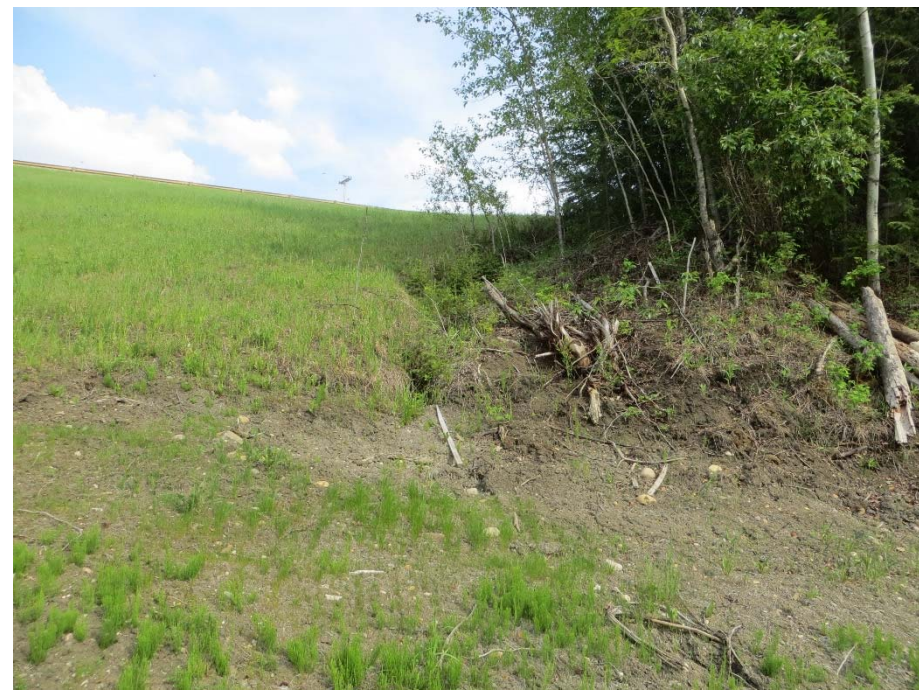
Photo 7. Looking southeast at small erosion rills along the downstream end of the ditch in the SW corner of the site. No significant change since 2014.
