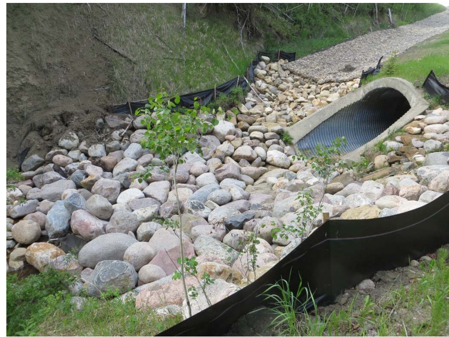
Photo 6. Looking north at outlet (west end) of the multi-plate culvert under the highway. Enhancements to the rip rap armouring were performed in June 2014 and northwest ditch gabion mattress was launched in the rip rap.
