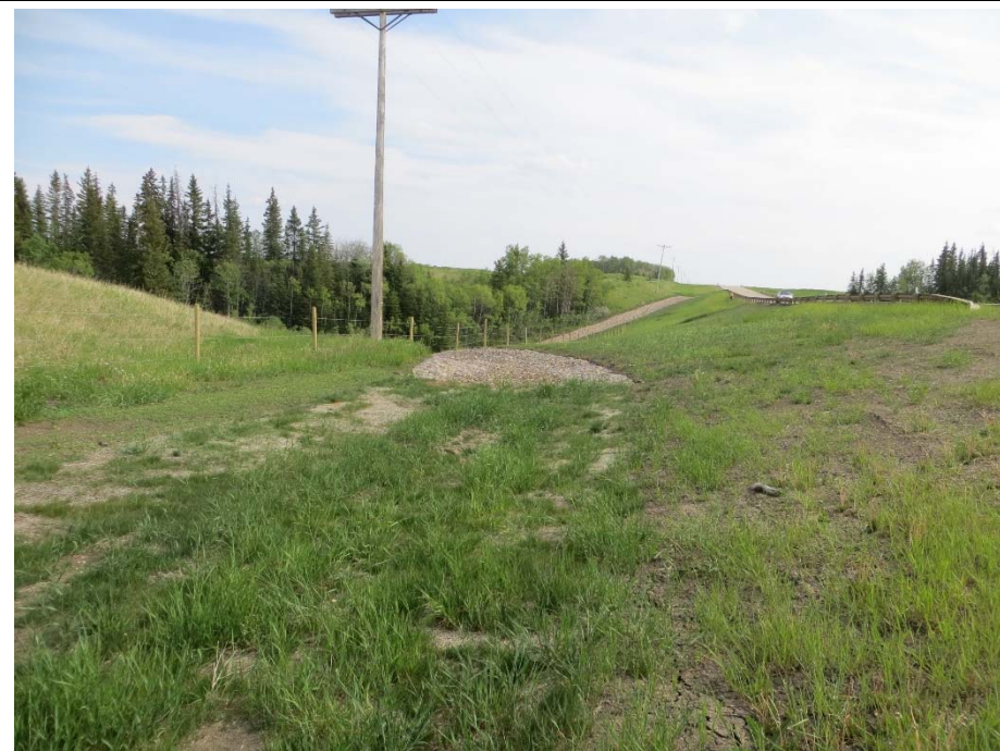
Photo 8. Looking south at RECP and gabion mattresses installed in June 2014 along the ditch bottom. Vegetation is sparse upslope towards the highway.
