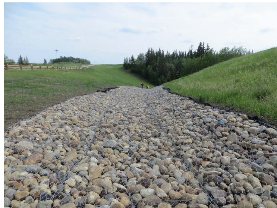
Photo 2. Looking south at gabion mattress placed in 2014 in NW corner of the site in ditch along the cut/fill contact.
