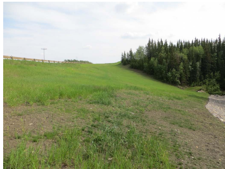
Photo 5. Looking south along the west side of the highway. Vegetation is sparse above the gabion mattresses.
