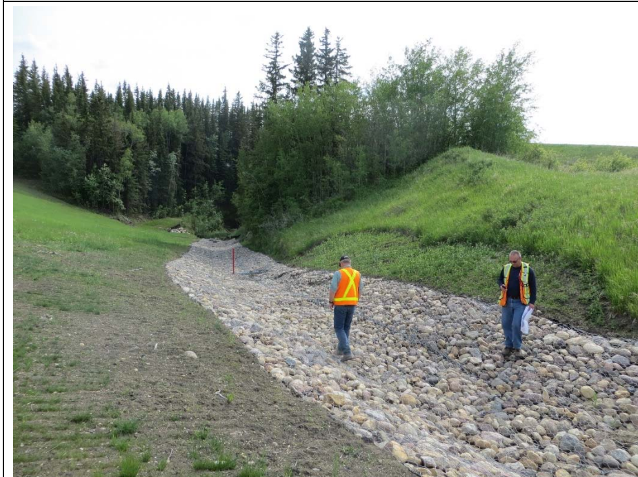
Photo 4. Looking southwest at a backslope failure above the northwest ditch that was repaired in June 2014 using the same method as the failure shown in Photo 3. Vegetation is sparse along the east side of the gabion mattress.
