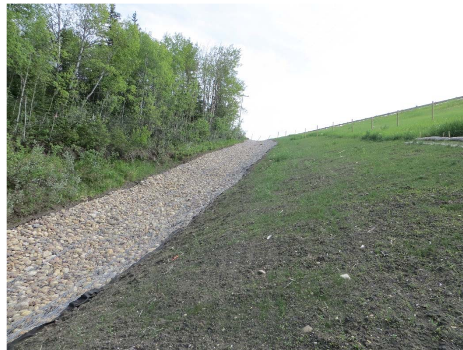
Photo 13. Looking southwest along the southeast ditch gabion mattress. Vegetation is sparse in the disturbed area along the highway sideslope (to the left of the mattresses).
