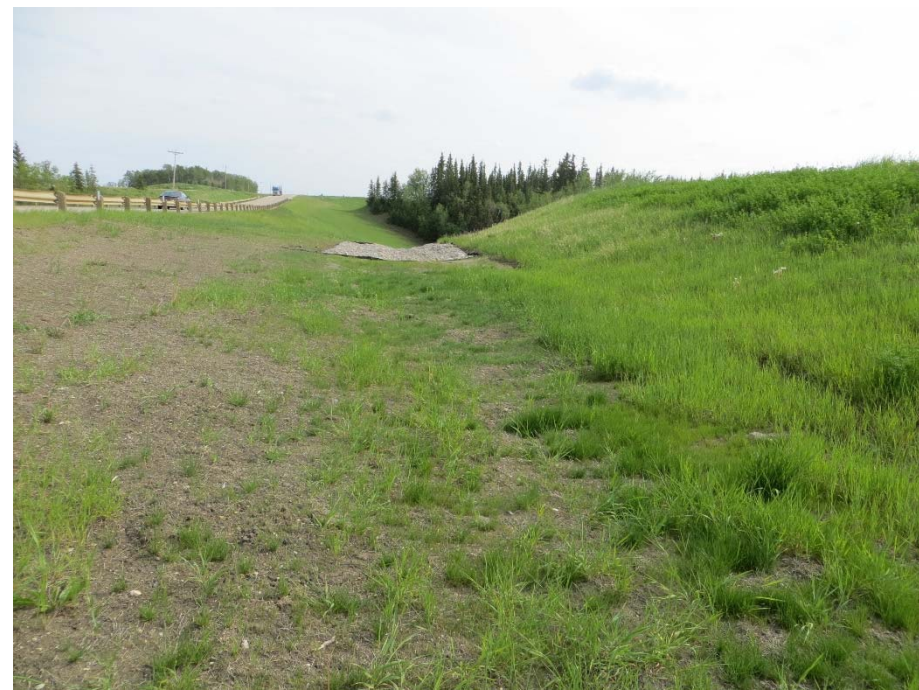
Photo 1. Looking south at RECP and gabion mattress placed in 2014 in NW corner of the site in ditch along the cut/fill contact.
