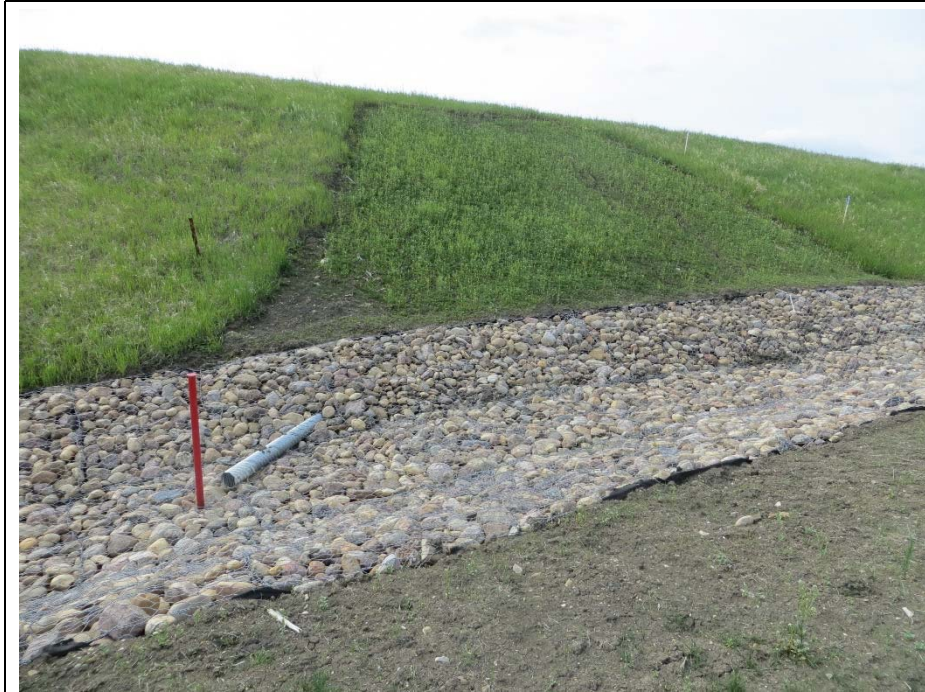
Photo 3. Looking northwest at a repaired backslope slump in the NW corner of the site. Failure was excavated in June 2014, a perforated subdrain pipe was placed in the resulting base, the excavation backfilled with compacted clay and the disturbed area was topsoiled and seeded. Vegetation has taken well with a few sparse areas along the perimeter of the disturbed area.
