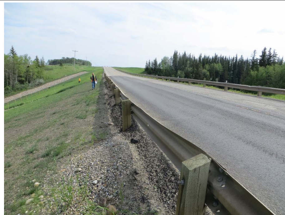
Photo 14. Looking southwest from the north end of the previous landslide backscarp in the roadway pavement. The asphalt pavement from the 2013/2014 repair has performed well. Some settlement is visible along the sawcuts and are reflecting through the new patch from October 2014.
