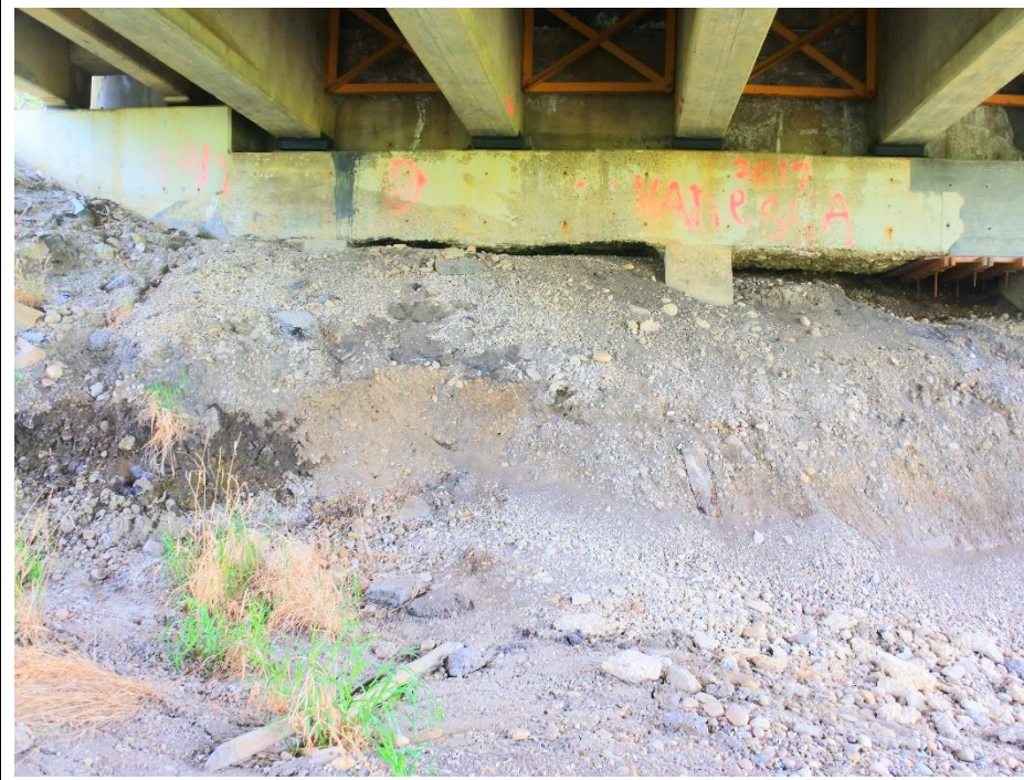
Photo 4. Looking south at the west side of the south abutment. Note the settlement of the soil. It appears that the bridge was widened after the original construction. Concrete counterforts are under the original bridge and steel H piles with cables are under the widened part.
