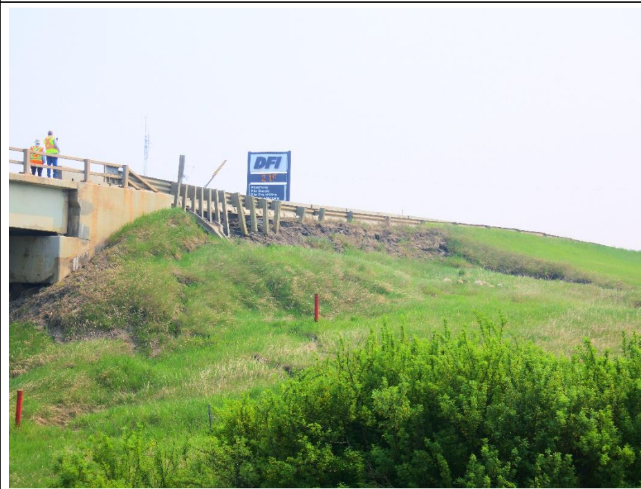
Photo 2. Looking east at the Slide 1 scarp along the edge of the road.
