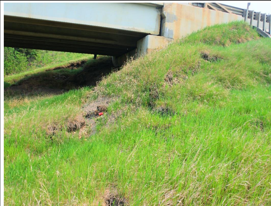
Photo 3. Looking east at the flank of Slide 1.
