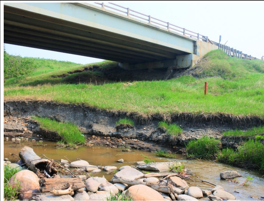
Photo 6. Looking at the south abutment. Note the river bank slumping.
