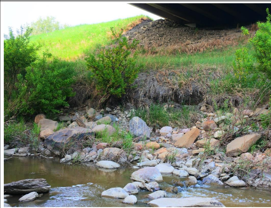
Photo 10. Looking north at 1m high scarp on north abutment.
