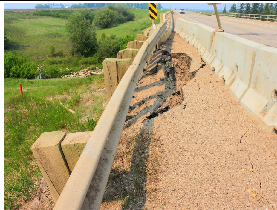
Photo 1. Looking north at the Slide 1 scarp cracks along the edge of the SBL.
