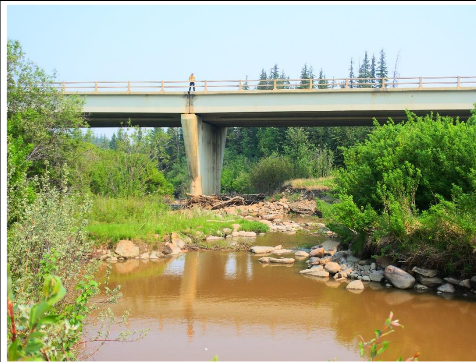
Photo 8. Looking downstream towards the bridge pier and bank erosion below the south abutment.
