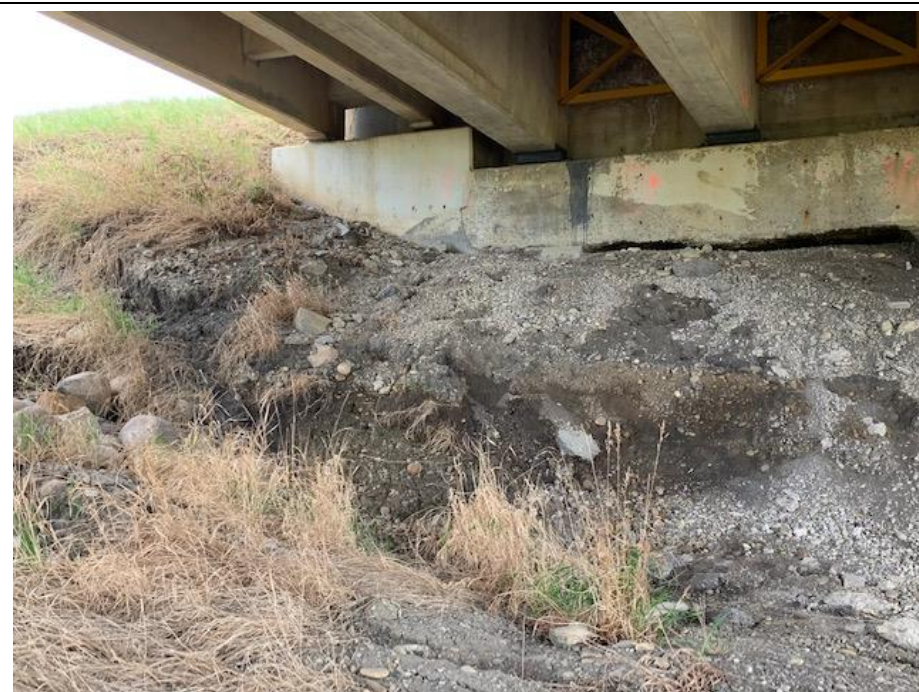
Photo 6. Looking at the south abutment and seepage coming out of it.
