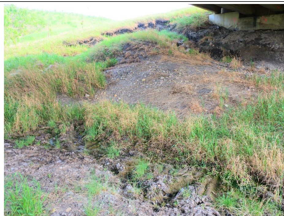
Photo 5. Looking southeast at the scarp and flank of Slide 2.
