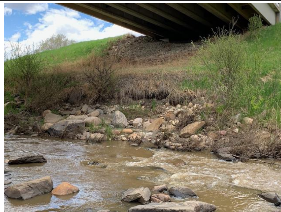
Photo 10. Looking north at 1m high scap on north abutment.
