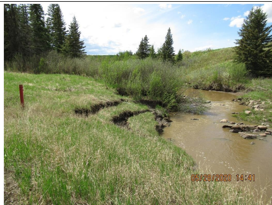
Photo 7. Looking upstream of the bridge at the river bank erosion/slumping. The toe of Slide 1 is located at the caragana bushes.
