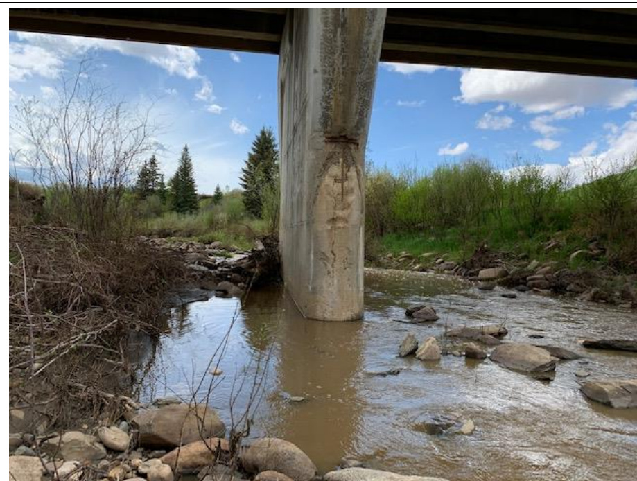
Photo 8. Looking upstream towards the bridge pier and build of debris against the pier.
