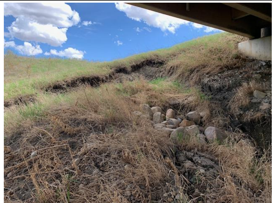
Photo 12. Looking southeast at the scarp and flank of Slide 2.
