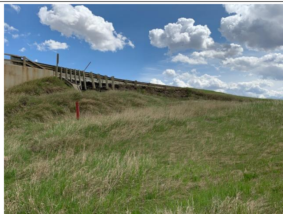
Photo 2. Looking east at the Slide 1 scarp along the edge of the road.
