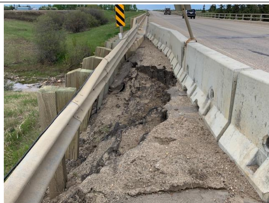
Photo 1. Looking north at the Slide 1 scarp cracks along the edge of the SBL.
