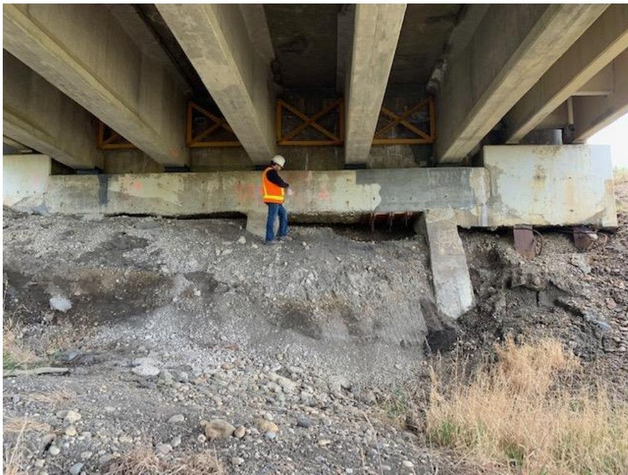
Photo 4. Looking south at the south abutment. Note the settlement of the soil. It appears that the bridge was widened after the original construction. Concrete counterforts are under the original bridge and steel H piles with cables are under the widened part.
