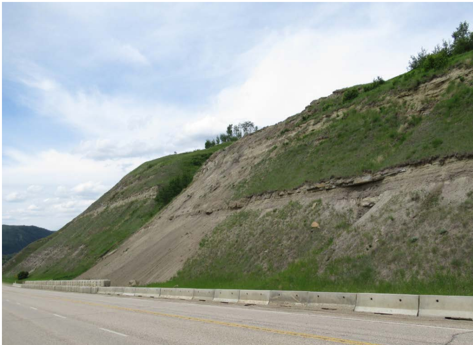
Photo 2: Looking northwest at the highway backslope below the landslide and concrete barriers
