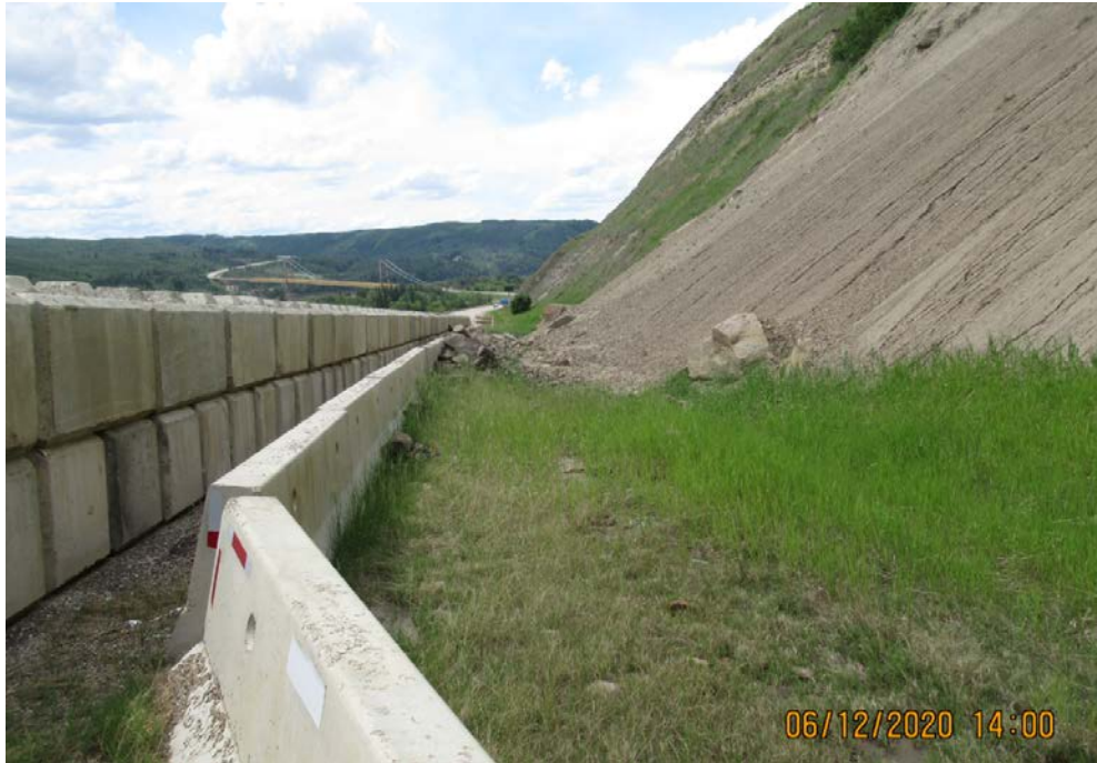
Photo 3: Looking west at accumulated debris from the SBL ditch of Hwy 2:68 at the highway backslope below the landslide
