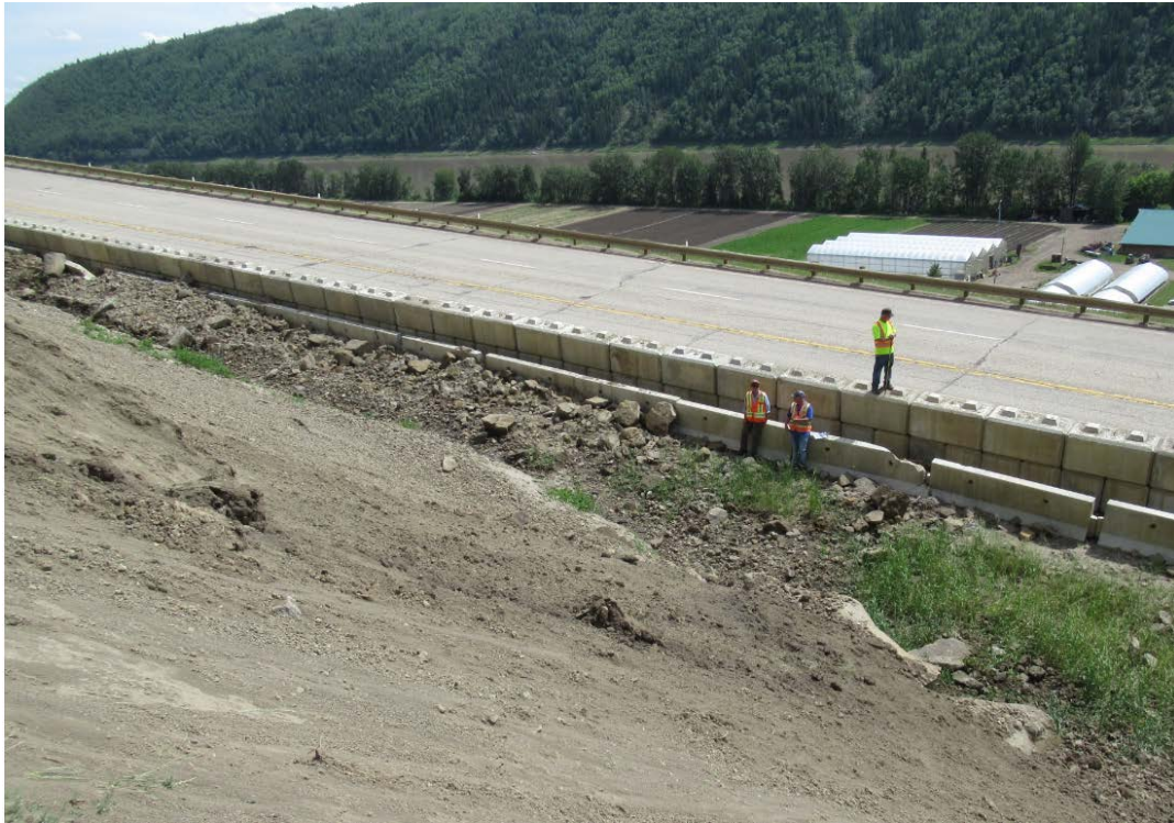
Photo 5: Looking southeast at landslide debris; note talus, boulders, and soil chunks that have accumulated in the ditch below the landslide
