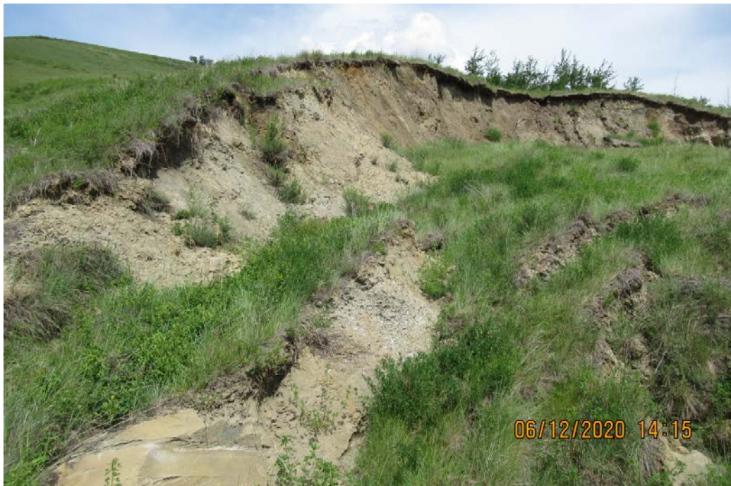
Photo 6: Looking northeast along backscarp of the landslide
