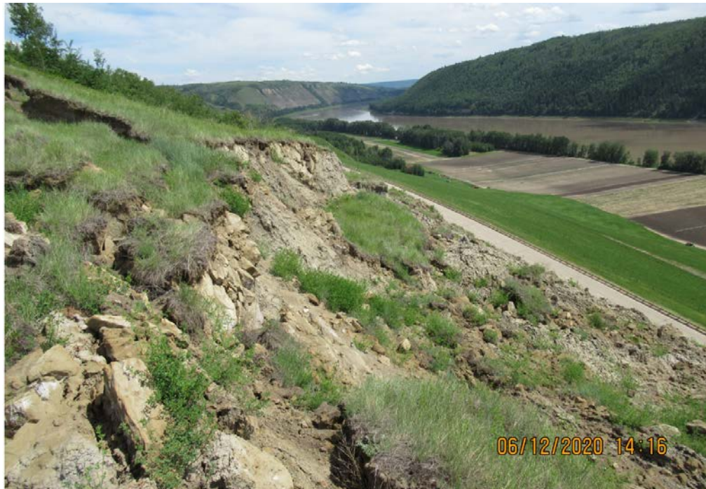
Photo 7: Looking east from landslide backscarp
