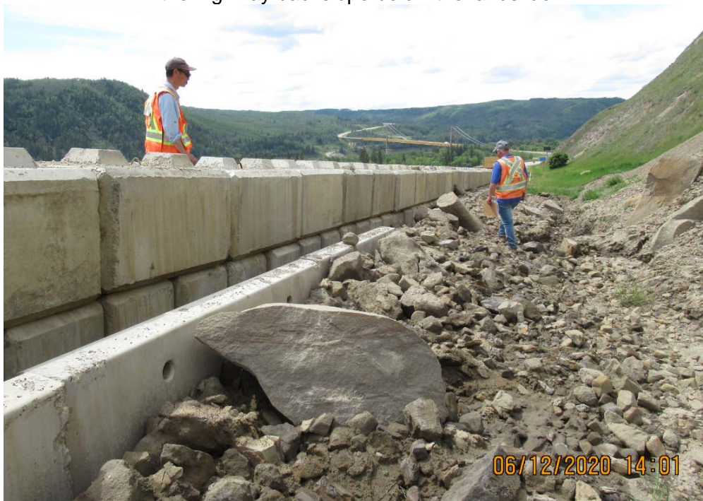
Photo 4: Looking west from SBL ditch of Hwy 2:68 at sandstone slabs, talus, boulders, and soil chunks that have accumulated between the ditch below the landslide and the Jersey Barrier
