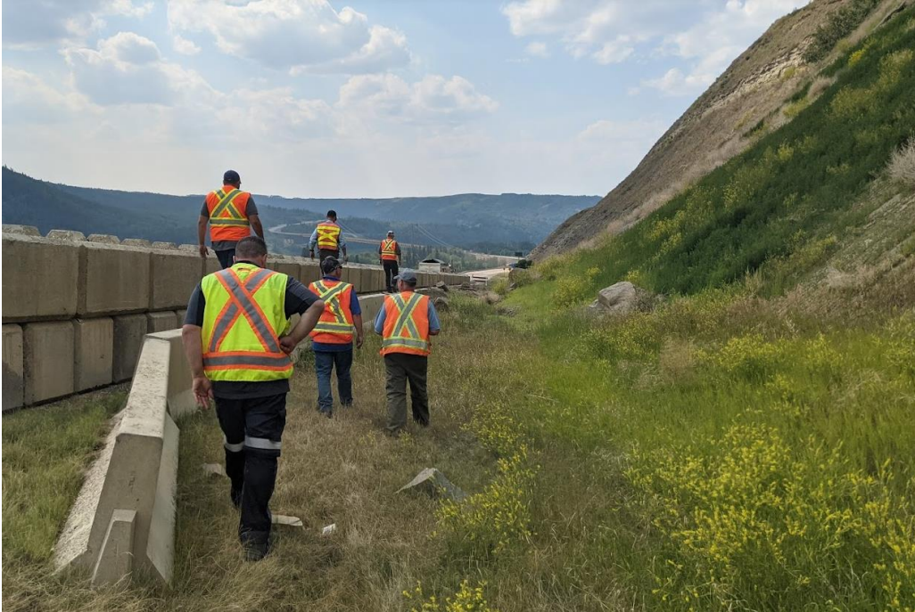
Photo 3: Looking west at accumulated debris in the ditch below the landslide. Note vegetation starting to grow on the backslope
