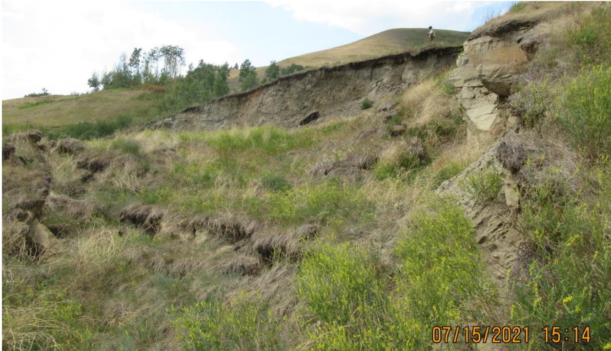
Photo 9: Looking west along the backscarp
