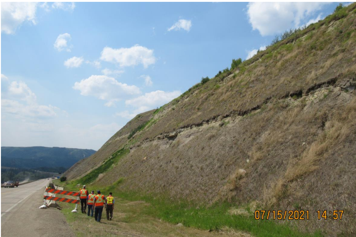
Photo 2: Looking west at the highway backslope below the landslide and concrete barriers
