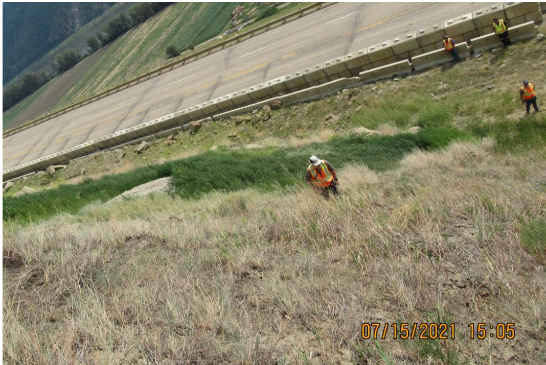
Photo 5: Looking southeast at landslide debris; note talus, boulders, and soil chunks that have accumulated in the ditch below the landslide
