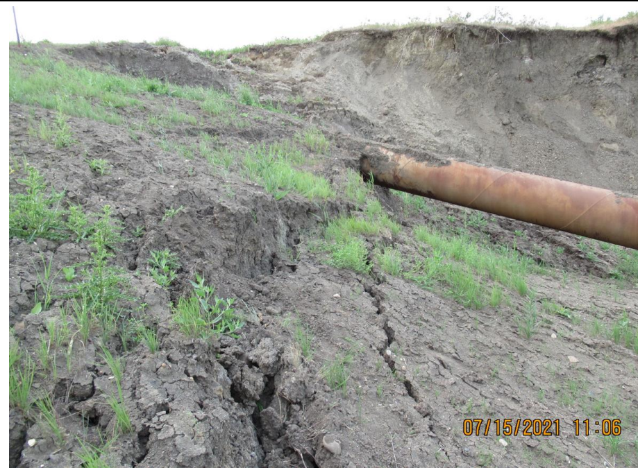
Photo 4. Close up of the settlement gap mentioned in Photo 3.
