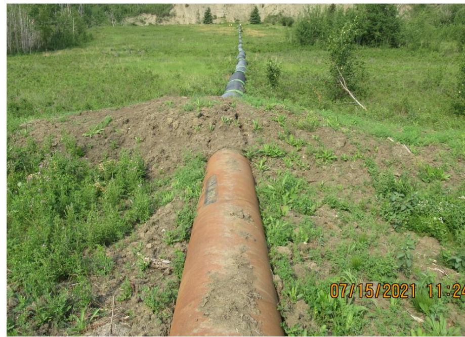
Photo 9. Looking downslope at SWSP connection into O pipe under a soil berm. Note how the pipe thermal movement resulted in 120 mm shift horizontal and some vertical cracks in the soil berm.
