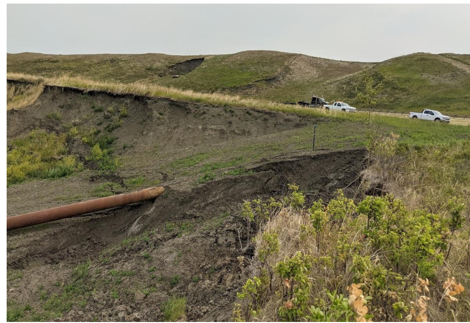
Photo 1. Looking northeast from Sta. 2+320 towards the Dunvegan Elephant Trunk consisting of a 760 mm diameter smooth wall steel pipe installed in 2020. Note vent pipe near the scarp crack.
