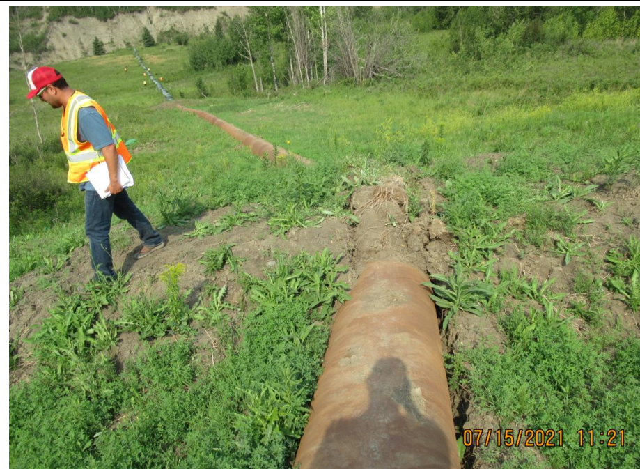
Photo 8. Looking downslope at SWSP lower bend and soil berm. Note how the pipe thermal movement resulted in 120 mm shift horizontal and some vertical cracks in the soil berm.
