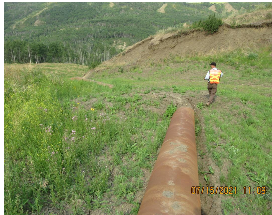
Photo 5. Looking west at the upper most pipe bend. Note the pipe shifted by about 250 mm at this location due to thermal effects
