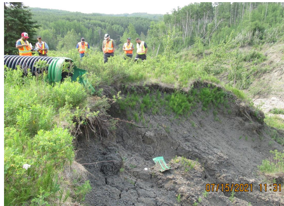
Photo 10. Looking south at big O pipe outlet at the Creek's top of bank.
