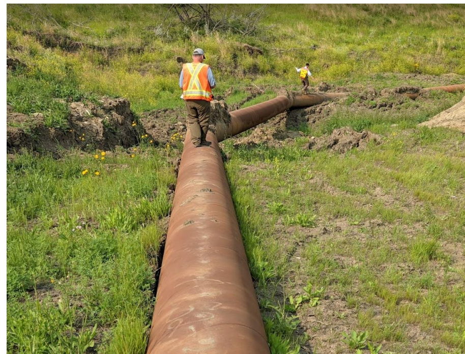
Photo 6. Looking west at the middle pipe bend. Note how the movement of the landslide under the pipe results in a gap approximately 1 m high.
