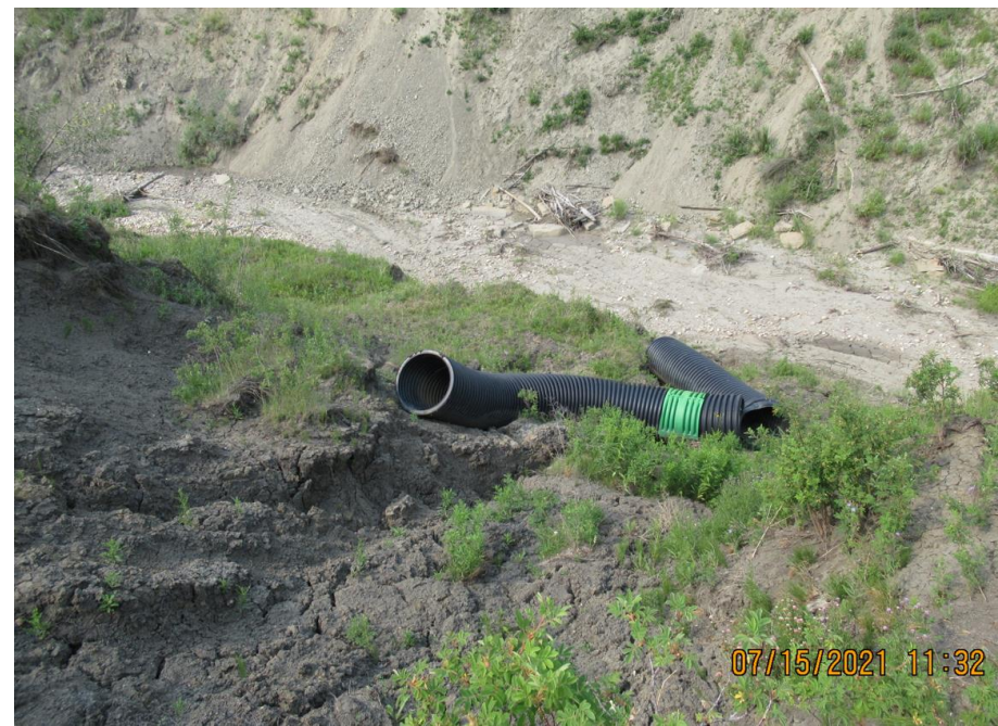
Photo 11. On going erosion along the Creek's bank has resulted in multiple dislocation of the big O pipe outlet.
