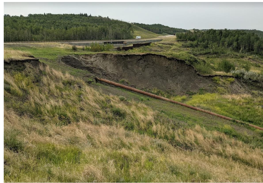
Photo 3. Looking south from 2+200, about 110m west of Hwy 2:68. Overall increase in slide activity along the backscarp in the upper portion of the Elephant Trunk drainpipe since 2020. Note up to 1.8 m of settlement of slide mass under the SWSP downslope of where it exits the fill cover.
