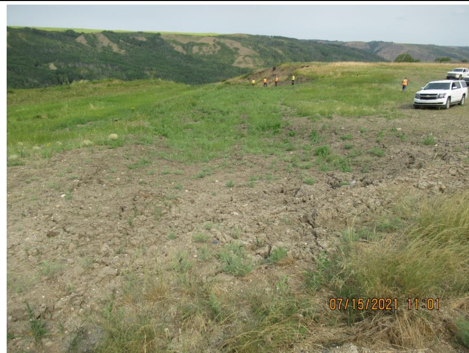
Photo 12. The trench backfill over the new SWSP has settled. The fill was placed in winter conditions.
